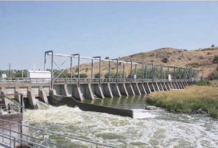
Courtesy Klamath Water Users Association Language in the the recent Klamath Basin Water Agreement Support Act doesn't allow water to be diverted from the Link River Dam if that would be detrimental to water contractors, according to the U.S. Department of the Interior.
