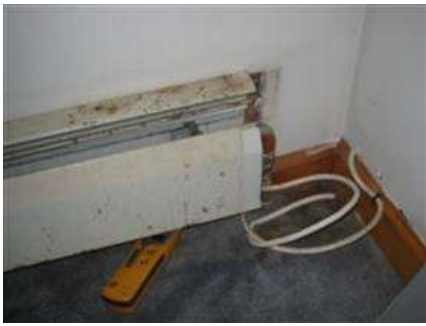
Photo 41 Front room near electric circuit box
