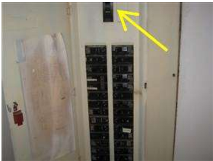
Photo 40 Main electric shut-off
