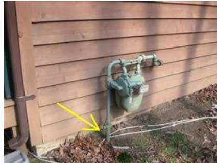
Photo 27 Main gas shut-off
