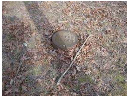
Photo 104 Water meter in front yard
