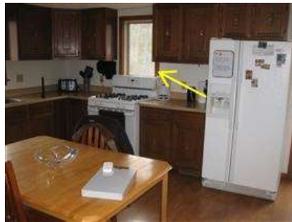
Photo 106 Kitchen. Wouldn't close.
