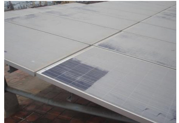
Left top corner coated with "Solar Glass Shield" and the difference after 21 days
