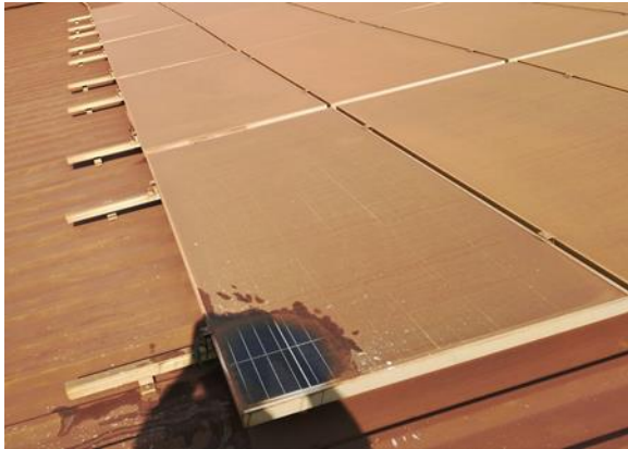
Panel covered with Industrial Dust as it was next to Foundry.
