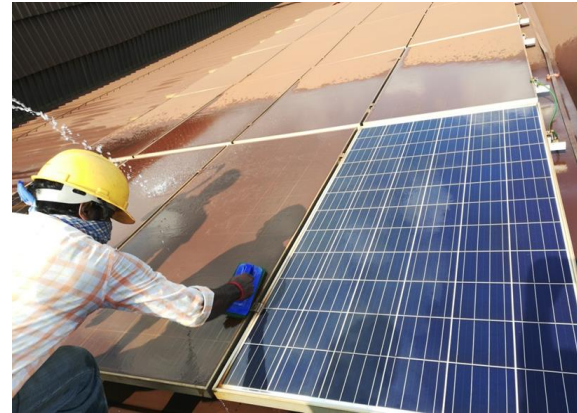
Few Panels of one String cleaned and then "Solar Glass Shield" applied.
