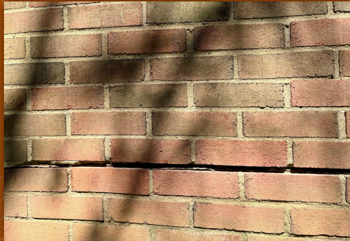
Cracks and missing mortar
