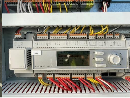
Photo 20 - Daikin Rooftop Air-Handling Unit Controller
