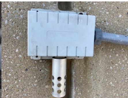
Photo 284 - Outdoor-Air Carbon Dioxide Transmitter
