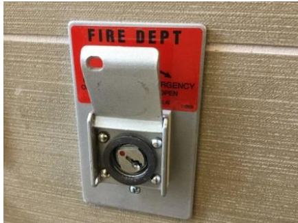
Photo 202 - Keyed HVAC Shutdown Switch
