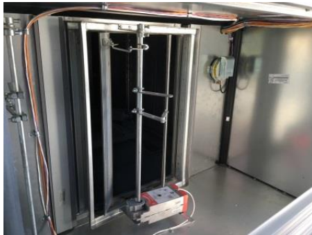
Photo 362 - Modulating Electric Actuator on Return Air Damper
