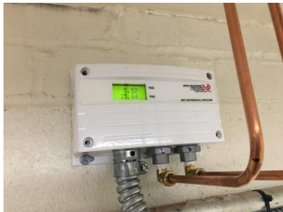
Photo 292 - HDPT (No Manifold)
