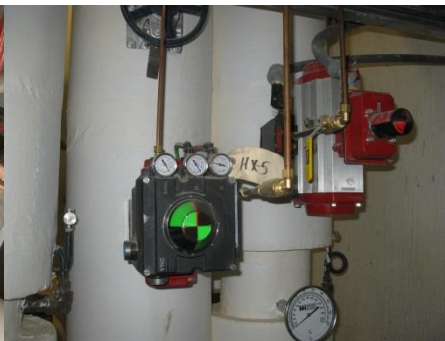
Photo 372 - Pneumatic High Temp. Hot Water Valve Actuators
