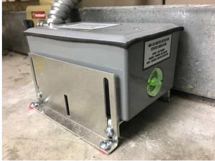
Photo 238 - Conductance Detector in an Elevator Pit
