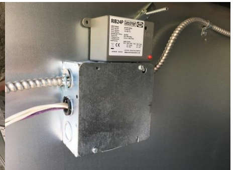
Photo 343 - RIB® Used for Electric Finned-Tube Radiation
