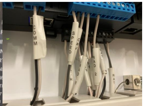
Photo 126 - Label Tape Wrapped Around Wire Sheath
