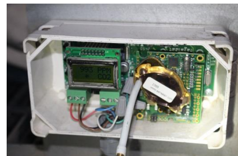
Photo 183 - Carbon Dioxide Gas Connected to CO2 Transmitter
