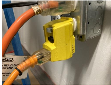
Photo 90 - Single Outlet Ground Fault Current Interrupter
