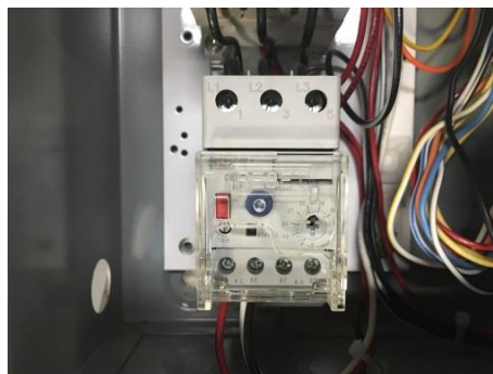
Photo 68 - Electronic Overload Protection
