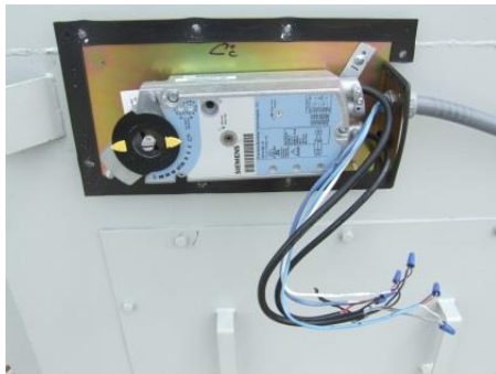
Photo 335 - Exhaust Damper Actuator with Position Feedback
