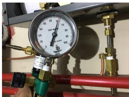
Photo 31 - Hydronic Diff. Press. Transmitter Comparison with Calibration Pump and Test Gauge
