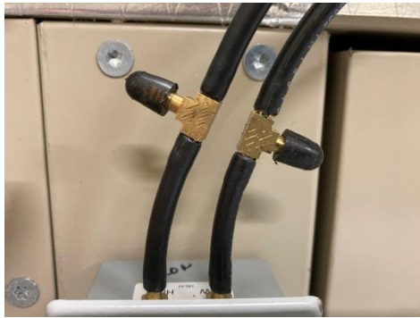
Photo 286 - Test Tees in Pneumatic Pressure Sensing Lines
