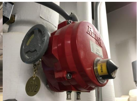
Photo 352 - Two-Position Heat Exchanger Control Valve
