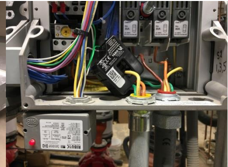
Photo 346 - RIB® Used for Three-Phase Pump Enable
