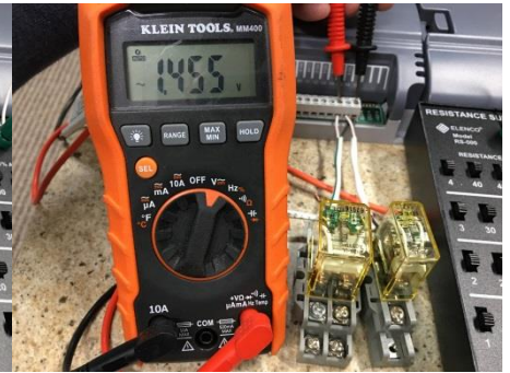
Photo 52 - Testing Binary Triac Output with DPDT Relay (De-energized)
