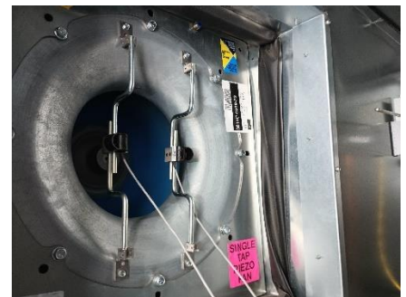
Photo 324 - Ebtron Thermal Dispersion Probes (Fan Inlet)
