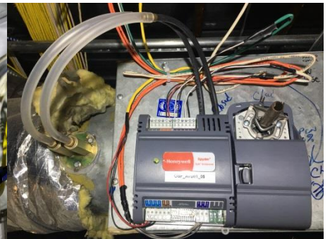
Photo 306 - Terminal Unit Controller Example #3
