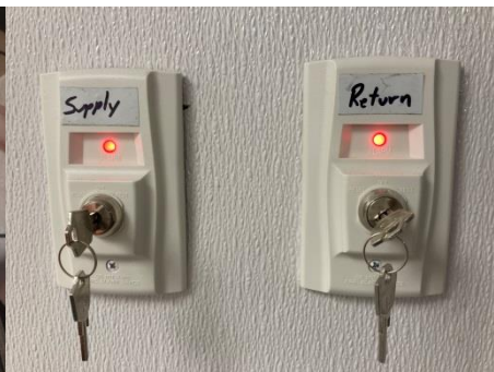
Photo 201 - Remote Smoke Detector Test Stations
