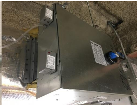
Photo 342 - RIBs® Used for Enabling Terminal Unit Heat Stages
