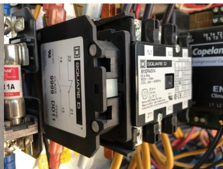
Photo 61 - Auxiliary Contacts of a Supply Fan Contactor
