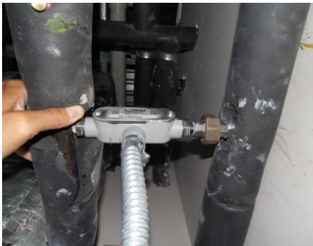
Photo 295 - HDPT Initially Installed without a Thermal Trap
