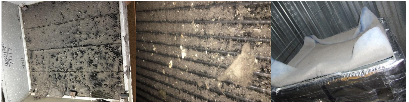
Photo 169 - Forgotten Supply Airflow Straightener
