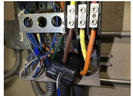
Photo 282 - Current Transmitter Installed in an Air-Handling Unit VFD
