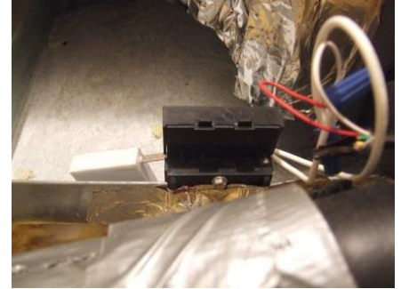
Photo 240 - Float Switch in a Condensate Drain Pan
