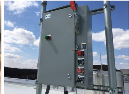
Photo 64 - Rooftop Exhaust Fan Combination Motor Starter/Disconnect Switch
