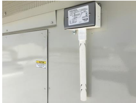
Photo 263 - Combination Temp. and Hum. Sensor (Under Rain Hood)
