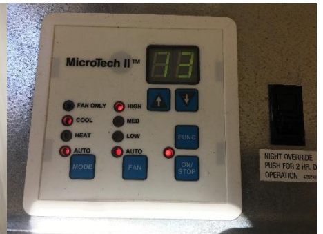
Photo 9 - Microtech II Controller in a Fan Coil Unit
