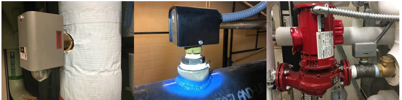
Photo 220 - Chilled Water Flow Switch Photo 221 - Condenser Water Flow Switch Photo 222 - Hot Water Flow Switch
