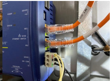
Photo 321 - Ethernet Communications Daisy-Chain Wiring
