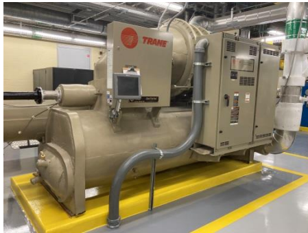
Photo 359 - Chilled Water Supply Temperature Setpoint Adjustment
