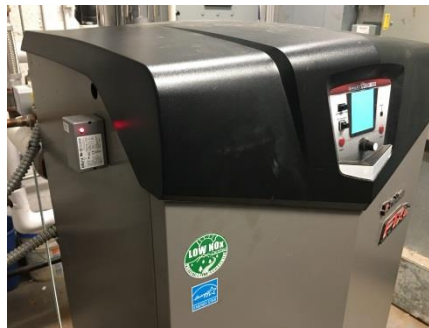
Photo 339 - RIBU1C Isolation Relay for Boiler Enable
