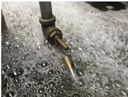
Photo 241 - Cooling Tower Float Switch
