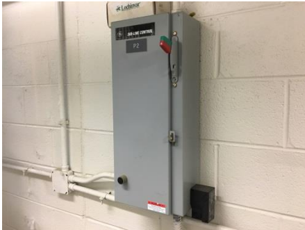
Photo 62 - Pump Combination Motor Starter/Disconnect Switch
