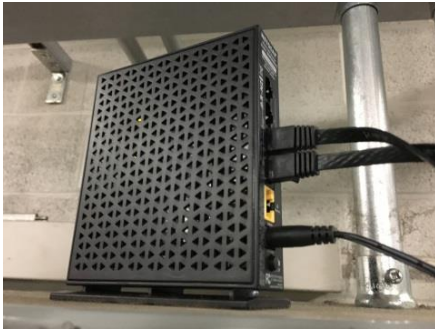
Photo 184 - Field Wi-Fi Router
