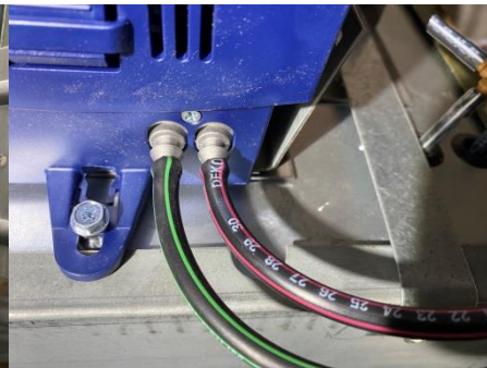
Photo 320 - Pneumatic Velocity Pressure Tubing Connections
