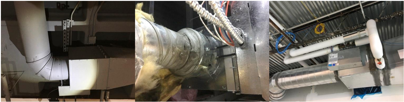
Photo 316 - 90-Degree Elbow at Terminal Unit Inlet
