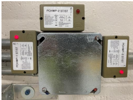
Photo 341 - RIB® Used for Single-Phase Pump Enable
