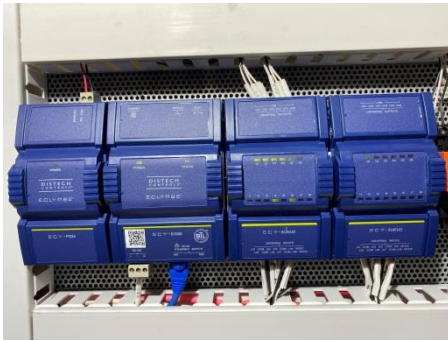
Photo 35 - Distech ECY-S1000 Controller with Expansion Modules
