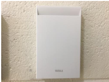
Photo 277 - Combination Temperature Sensor and Humidity Transmitter
