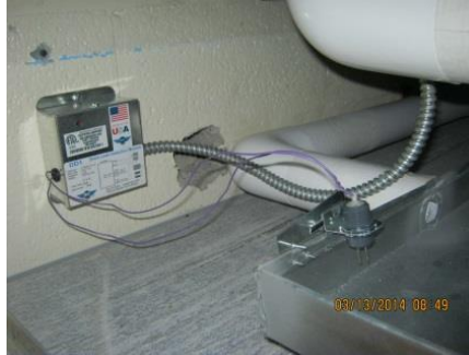
Photo 239 - Conductance Detector on a Condensate Drain Pan
