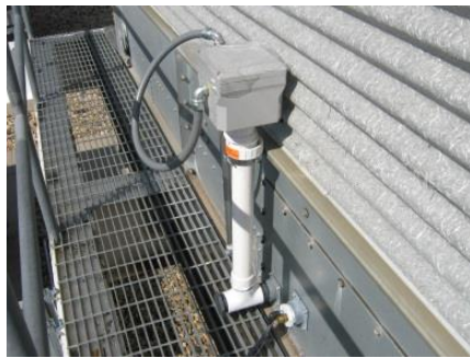
Photo 242 - Cooling Tower Conductance Level Indicator
