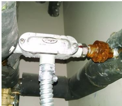
Photo 296 - Condensation On and Inside HDPT Enclosure
