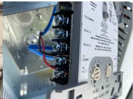
Photo 198 - Typical Fire Alarm Relay Module Contacts (Without Cover)
