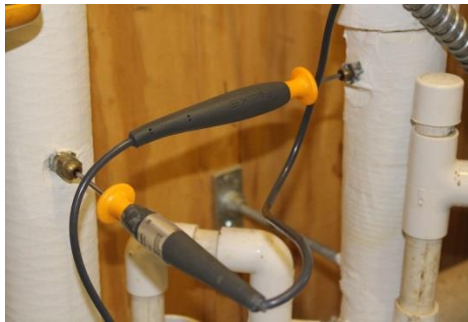
Photo 95 - P/T Ports Used for Temperature Differential Measurement
