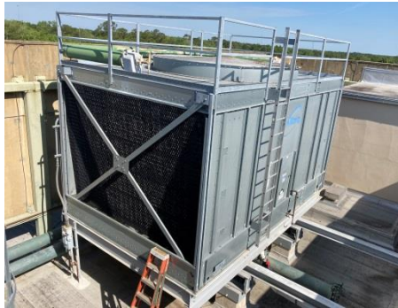
Photo 386 - Cooling Tower Fan Speed Control
