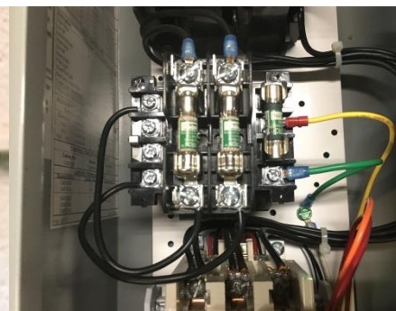
Photo 70 - Control Transformer and Fuses
