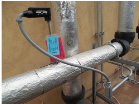
Photo 332 - Onicon Turbine Insertion Flow Meter
