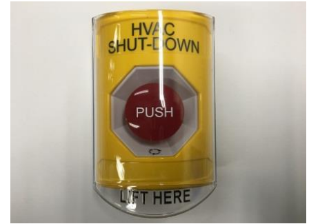
Photo 204 - Push Button Emergency Shutdown Switch
