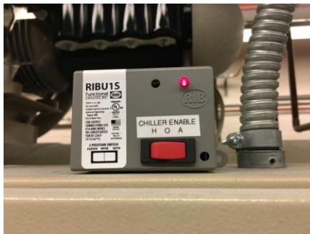
Photo 338 - RIBU1S Isolation Relay for Chiller Enable
