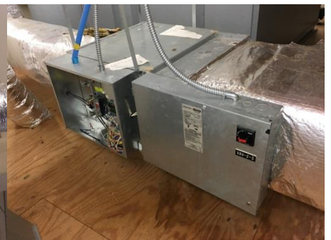
Photo 309 - Typical Single-Duct Terminal Unit with Electric Heat
