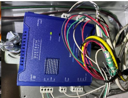
Photo 305 - Terminal Unit Controller Example #2
