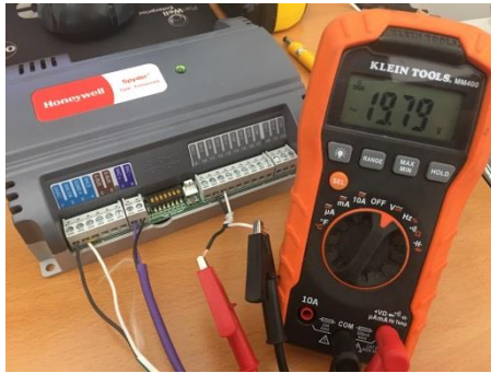
Photo 50 - Testing Binary Triac Output with No Load (De-energized)
