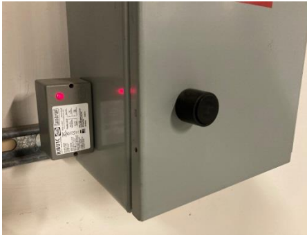
Photo 344 - RIB® Used for Three-Phase Exhaust Fan Enable
