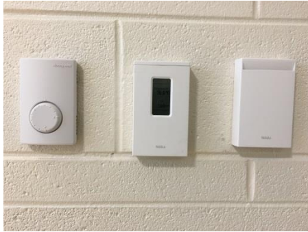
Photo 244 - Individual Temperature, Humidity, and CO2 Sensors
