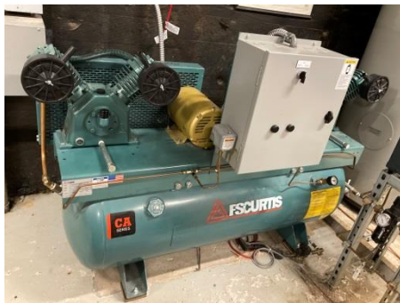
Photo 374 - Control Air Compressor
