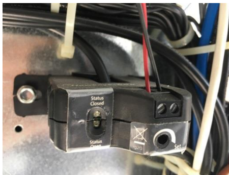
Photo 205 - CSR on a Hot Water Pump
