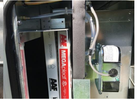
Photo 213 - Automatic Reset ADPS for Filter Monitoring
