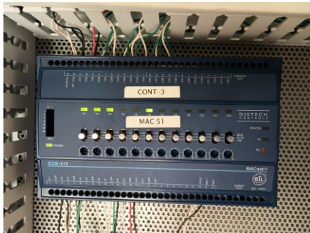
Photo 4 - Distech ECB-410 Programmable Controller
