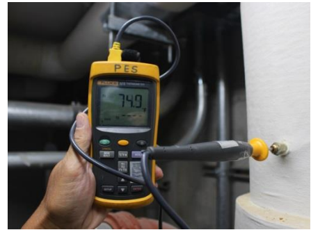
Photo 153 - Piercing Probe at P/T Port (Condenser Water)
