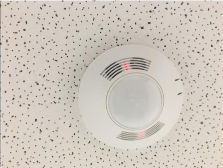
Photo 227 - Ceiling-Mounted Occupancy Detector
