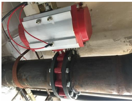
Photo 353 - Pneumatic Two-Position Condenser Water Valve Actuator
