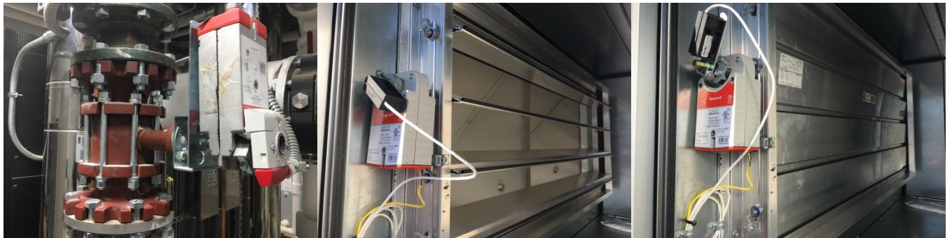
Photo 347 - Two-Position Boiler Isolation Control Valve
