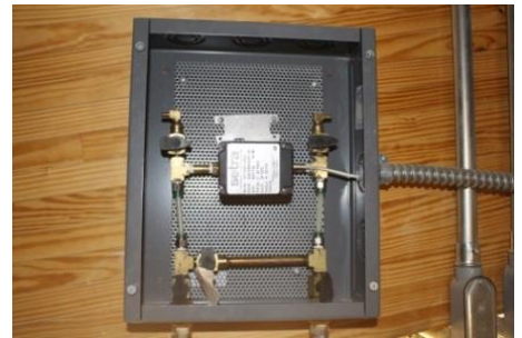
Photo 294 - HDPT with Five-Port Manifold
