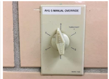
Photo 231 - Occupancy Override Timer Switch
