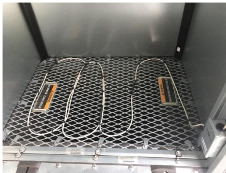
Photo 259 - Flexible Averaging Temperature Sensor at Supply
