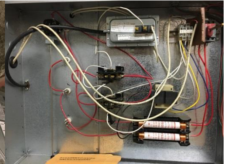
Photo 358 - Electric Duct Heater Control Panel
