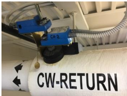
Photo 236 - Chilled Water Control Valves with Auxiliary Contacts
