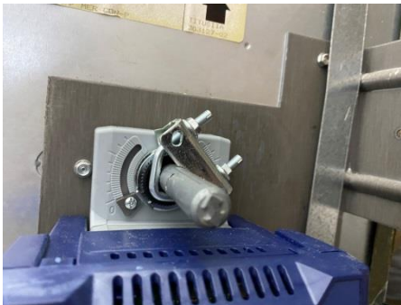
Photo 319 - Actuator/Damper Shaft Connection
