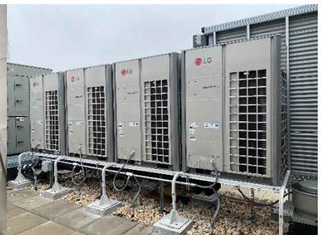
Photo 18 - LG Variable Refrigerant Flow (VRF) Condensing Units
