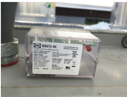
Photo 56 - RIBU1C-N4 on a Rooftop Exhaust Fan Motor Starter Enclosure
