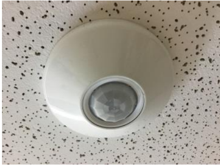
Photo 226 - Ceiling-Mounted Occupancy Detector
