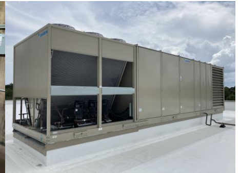
Photo 15 - Rooftop Air-Handling Unit
