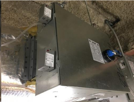
Photo 357 - Staged Electric Duct Heater for VAV Box
