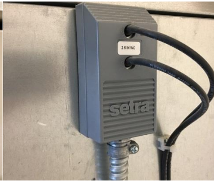
Photo 287 - Filter Differential Pressure Monitoring
