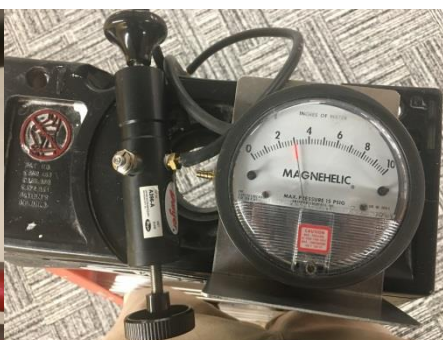
Photo 32 - Magnehelic® Gauge and Calibration Pump to Calibrate an Air Differential Pressure Transmitter
