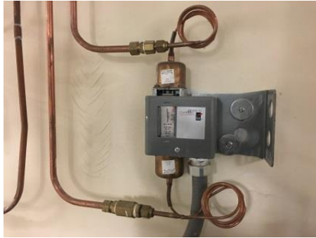
Photo 217 - Differential Pressure Switch #1
