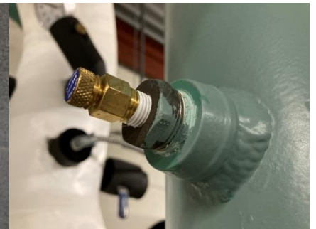
Photo 97 - Close up of P/T Port On Condenser-Water Piping
