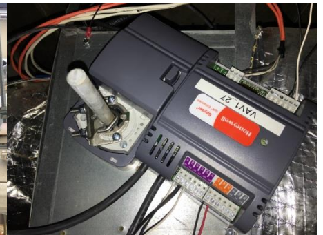
Photo 370 - VAV Controller with a Floating Damper Actuator
