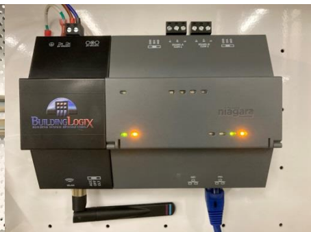
Photo 3 - Building Logix JACE
