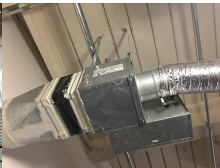
Photo 308 - Typical Single-Duct Terminal Unit with No Heat Coil
