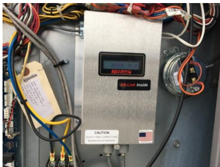
Photo 322 - Ebtron Thermal Dispersion Control Panel
