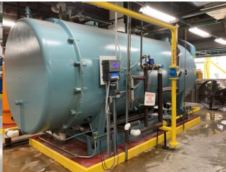
Photo 360 - Boiler Steam Pressure Setpoint Adjustment
