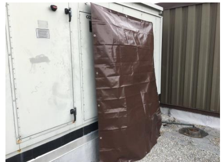
Photo 120 - Temporary Cover for Controls Laptop
