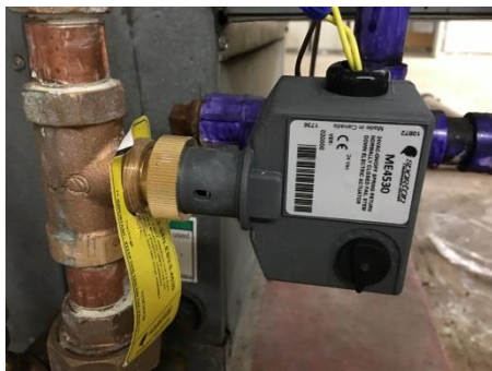
Photo 350 - Two-Position Water Source Heat Pump Control Valve
