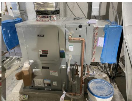
Photo 17 - Water-Source Heat Pump Air-Handling Unit
