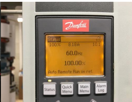
Photo 26 - VFD Commanded to 100% Speed Output (60 Hertz)
