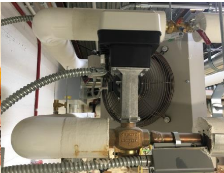
Photo 369 - Hot Water Control Valve with a Floating Actuator
