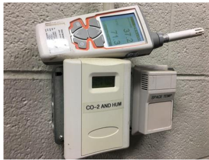
Photo 158 - Humidity Meter at Space Humidity Transmitter
