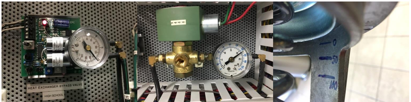
Photo 377 - Electric to Pneumatic Transducer
