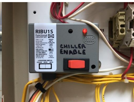
Photo 57 - RIBU1S in a Chiller Control Panel
