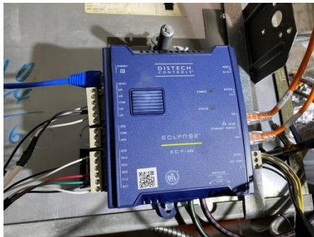
Photo 304 - Terminal Unit Controller Example #1
