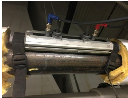
Photo 143 - Ultrasonic Sensor /Transmitter on Pipe Surface
