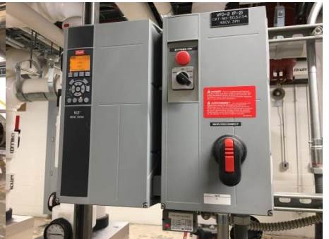
Photo 361 - Pump VFD Speed Command
