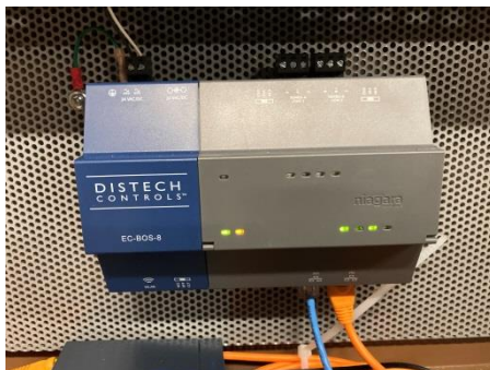
Photo 1 - Distech Controls EC-BOS-8 JACE
