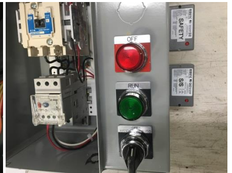
Photo 67 - Enable & Safety Relays
