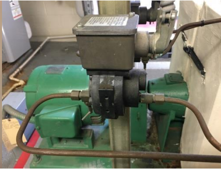
Photo 218 - Differential Pressure Switch #2
