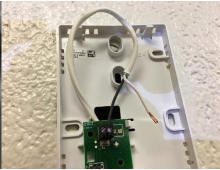
Photo 23 - Wire Removed from Space Temp Sensor
