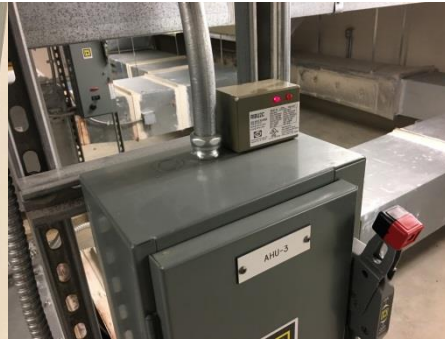
Photo 345 - RIB® Used for Three-Phase Air-Handling Unit Enable
