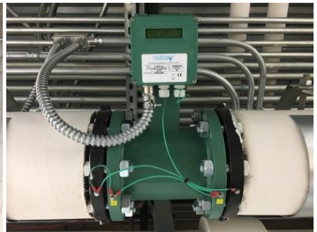
Photo 334 - Onicon Magnetic Inline Flow Meter
