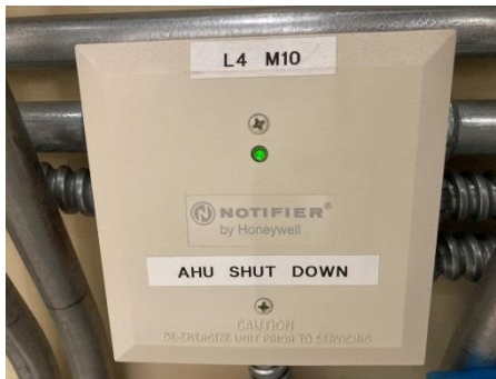
Photo 196 - Fire Alarm Relay Module for Air-Handling Unit Shutdown
