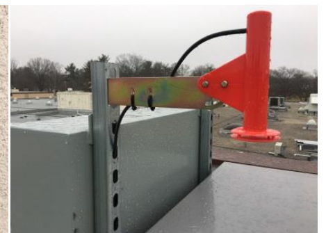
Photo 291 - Outdoor Air Reference Static Pressure Pickup
