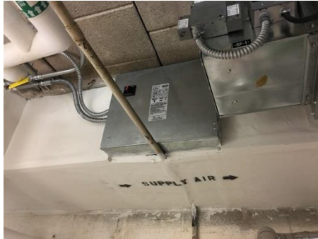
Photo 356 - Staged Electric Duct Heater on Make-Up Air Unit
