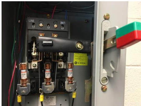
Photo 65 - Disconnect Switch & Fuses
