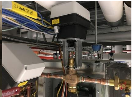
Photo 364 - Modulating Electric Actuator on Two-Way Control Valve
