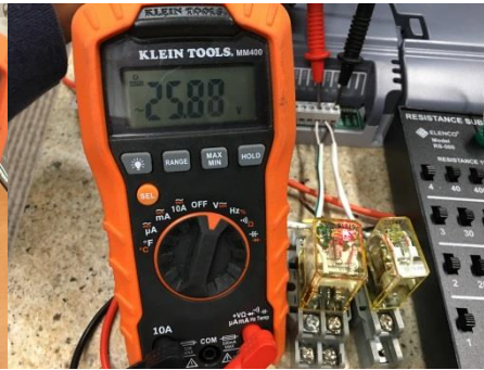
Photo 51 - Testing Binary Triac Output with DPDT Relay (Energized)
