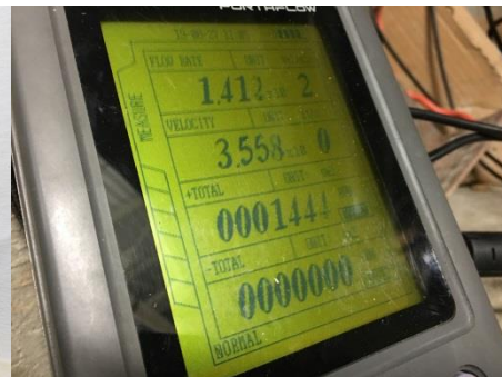
Photo 30 - Hydronic Flow Comparison with Ultrasonic Flow Meter
