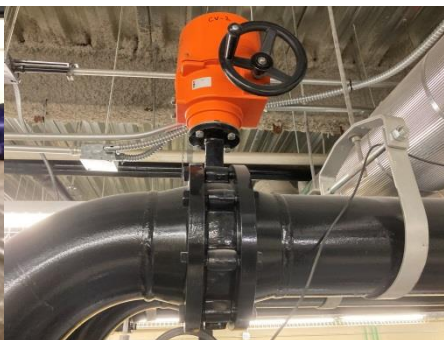
Photo 351 - Two-Position Condenser Water Isolation Control Valve
