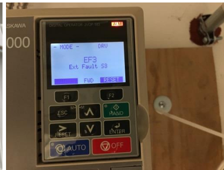
Photo 394 - Yaskawa External Fault Code
