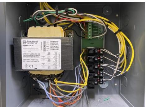
Photo 40 - 500 VA Enclosed Transformer with Five 100 VA Switched Circuits
