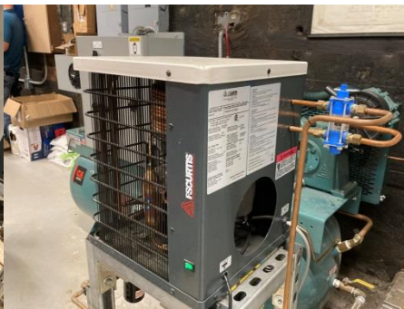
Photo 375 - Compressed Air Dryer
