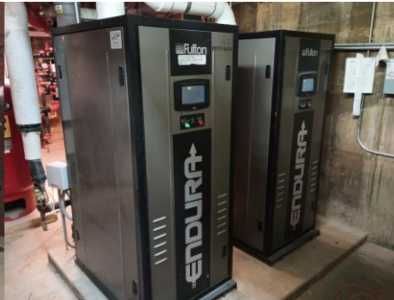
Photo 14 - High Efficiency Modular Boiler Plant
