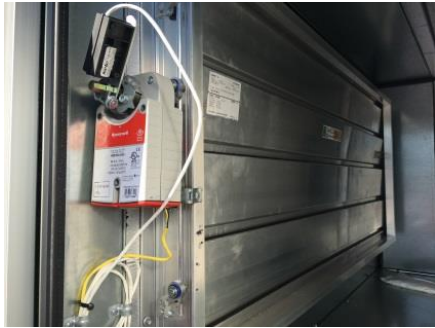
Photo 232 - Position Switch on Outdoor Air Damper
