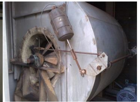
Photo 373 - Pneumatic Inlet Guide Vane Actuator
