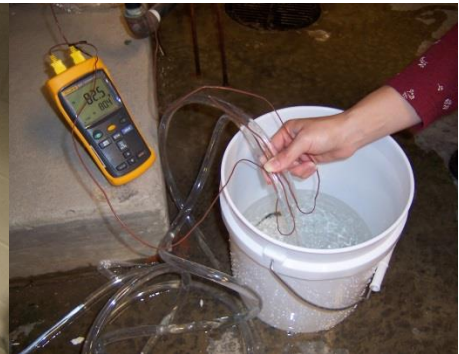
Photo 101 - Measurement of Chiller Condenser Water Temps.
