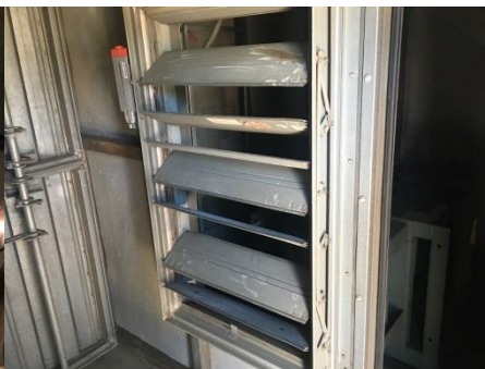
Photo 366 - Modulating Electric Return Air Damper Actuator
