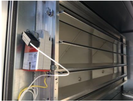
Photo 233 - Position Switch on Outdoor Air Damper
