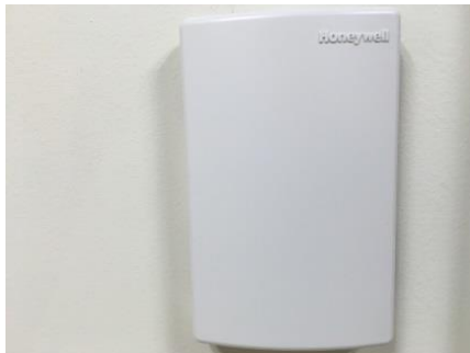
Photo 250 - Space Temperature Sensor
