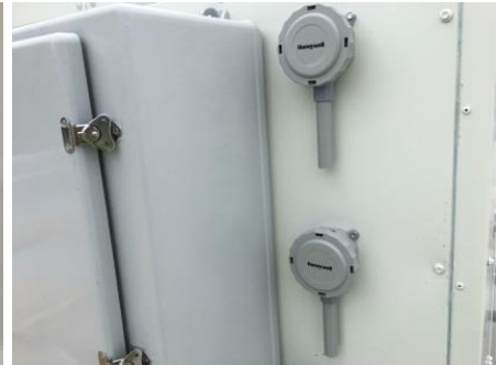
Photo 264 - Outdoor Air Temp. Sensor Mounted on Rooftop Unit
