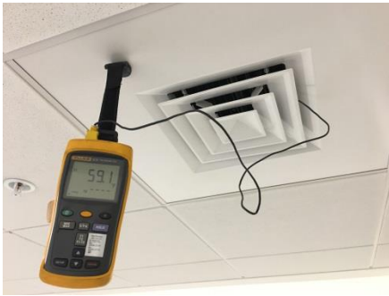
Photo 151 - Bead Probe in Supply Air Diffuser
