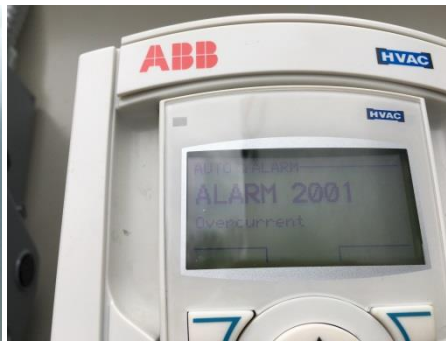
Photo 393 - ABB VFD Overcurrent Fault Code
