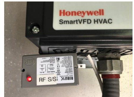
Photo 340 - RIBU1C Isolation Relay for Return Fan VFD Enable
