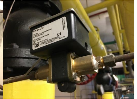
Photo 219 - Differential Pressure Switch #3
