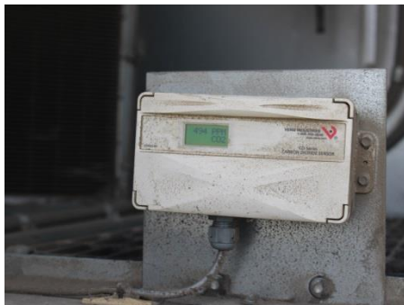
Photo 283 - Duct-Mounted Carbon Dioxide Transmitter
