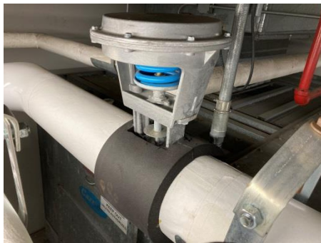
Photo 371 - Pneumatic Chilled Water Valve Actuator
