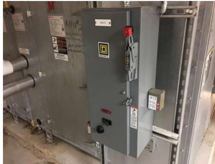
Photo 63 - Air-Handling Unit Combination Motor Starter/Disconnect Switch
