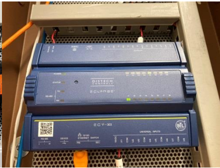
Photo 36 - Distech ECY-303 Controller
