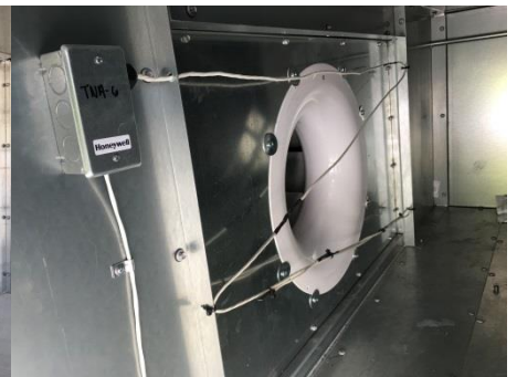
Photo 261 - Flexible Averaging Temperature Sensor at Supply Fan
