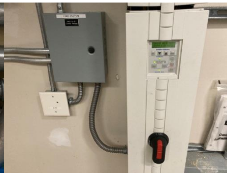
Photo 197 - Fire Alarm Relay Module next to VFD
