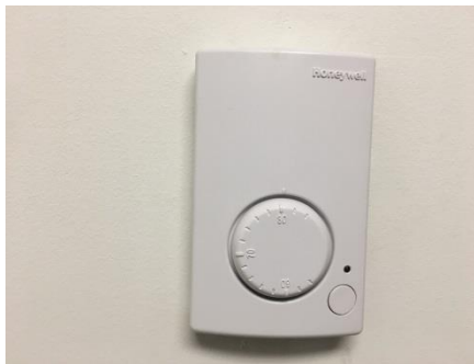
Photo 230 - Occupancy Override Button
