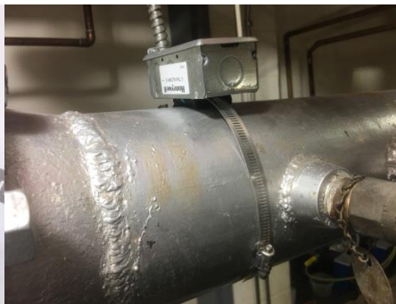
Photo 269 - Strap-On Temperature Sensor on Condenser Water Piping
