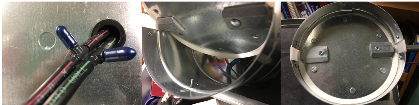
Photo 313 - VAV Terminal Unit Test Tees with Caps
