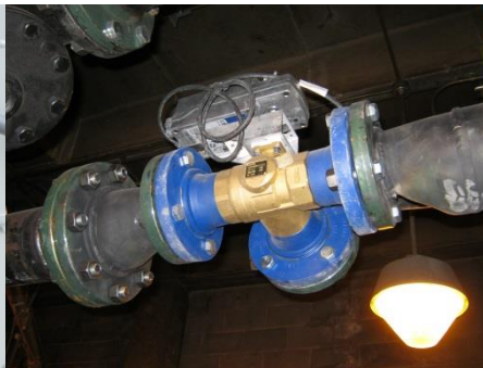
Photo 336 - Chilled Water Bypass Valve with Position Feedback
