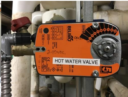
Photo 363 - Modulating Electric Actuator on Two-Way Control Valve
