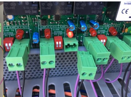
Photo 82 - Safety Device Terminal Lifted to Simulate an Alarm Condition
