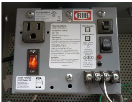
Photo 38 - Enclosed Transformer with High/Low Switches and Circuit Breaker
