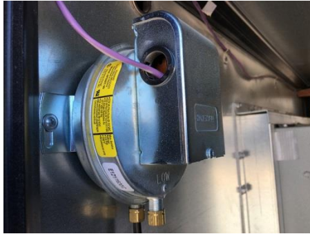
Photo 211 - Automatic Reset ADPS for Fan Status Monitoring
