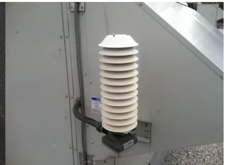
Photo 279 - Outdoor Air Humidity Transmitter
