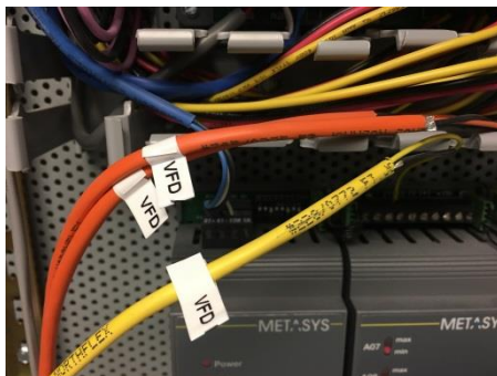
Photo 124 - Label Tape Wrapped around Control Wires
