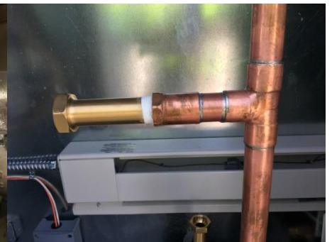
Photo 270 - Thermowell in Small Diameter Piping
