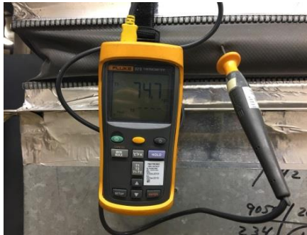
Photo 152 - Piercing Probe at Air-Handling Unit Flexible Connection
