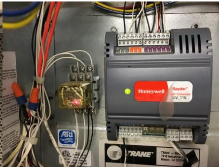
Photo 5 - Honeywell Spyder PUB4024S Programmable Controller
