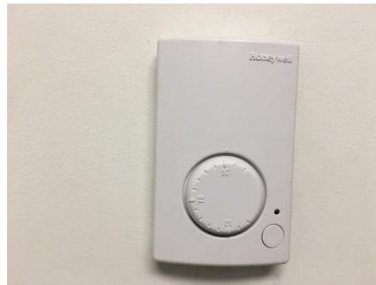
Photo 251 - Space Temp. with Occ. Override and Setpoint Adjustment
