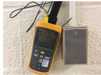
Photo 159 - Bead Probe at Space Temperature Sensor
