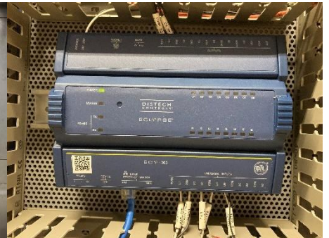
Photo 6 - Distech ECY-303 Programmable Controller
