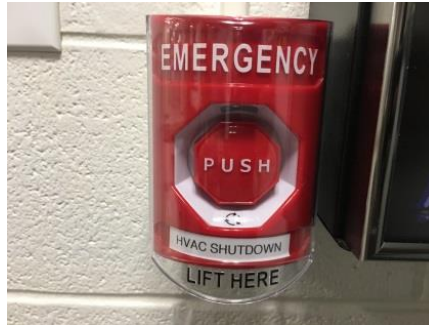
Photo 203 - Push Button Emergency Shutdown Switch
