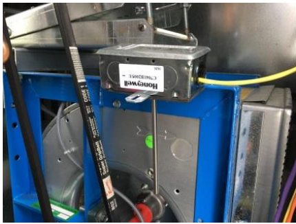
Photo 253 - Probe Temperature Sensor (Monitoring Exhaust Air Temp.)
