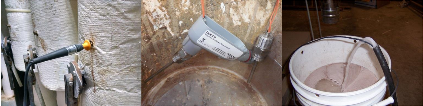
Photo 274 - Piercing Probe Temperature Readings
