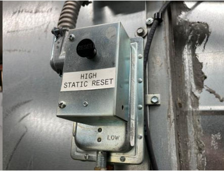
Photo 212 - Manual Reset High Static Safety Switch
