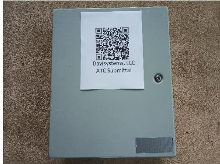
Photo 187 - QR Code for ATC Submittal on Local Control Panel
