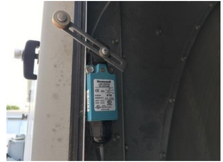
Photo 234 - Rocker Switch on Air-Handling Unit Door
