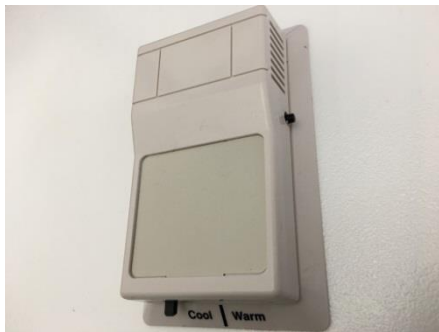
Photo 229 - Occupancy Override Button (Side)
