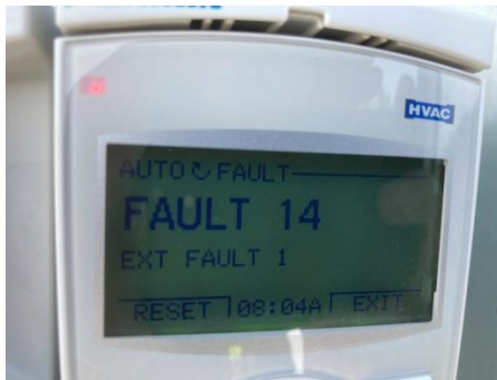
Photo 392 - ABB VFD External Fault Code
