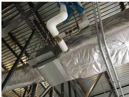
Photo 307 - Typical Single-Duct Terminal Unit with Hot Water Heat Coil
