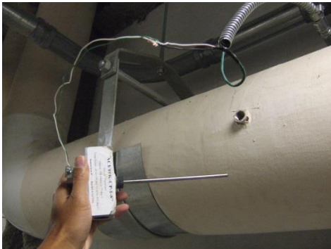
Photo 99 - Removal of Immersion Temp. Sensor from Thermowell
