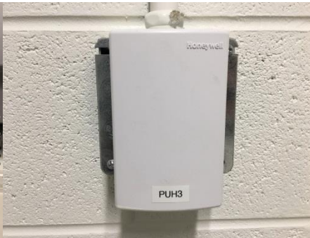
Photo 128 - Label Tape on Space Temperature Sensor
