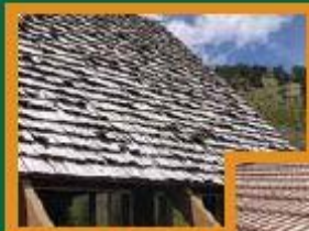
Figure 8: (above) Wood shingle roofs are highly flammable and not recommended. Photo: CSFS
