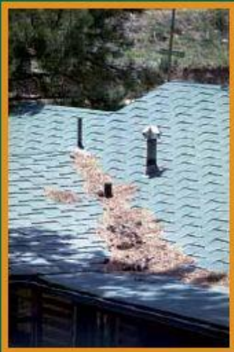
Figure 15: Clearing pine needles and other debris from the roof and gutters is an easy task that should be done at least once a year. Photo: CSFS
