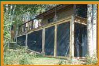
Figure 16: Enclosing decks with metal screens can prevent embers from igniting a house. Photo: Marilyn Brown, La Plata County
