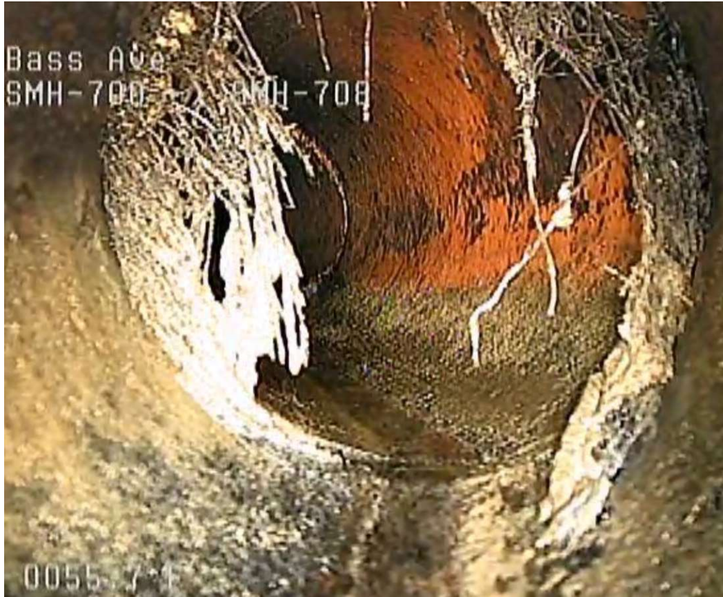
Photograph 5: Sewer service located approximately 56 linear feet down stream of SMH_700
