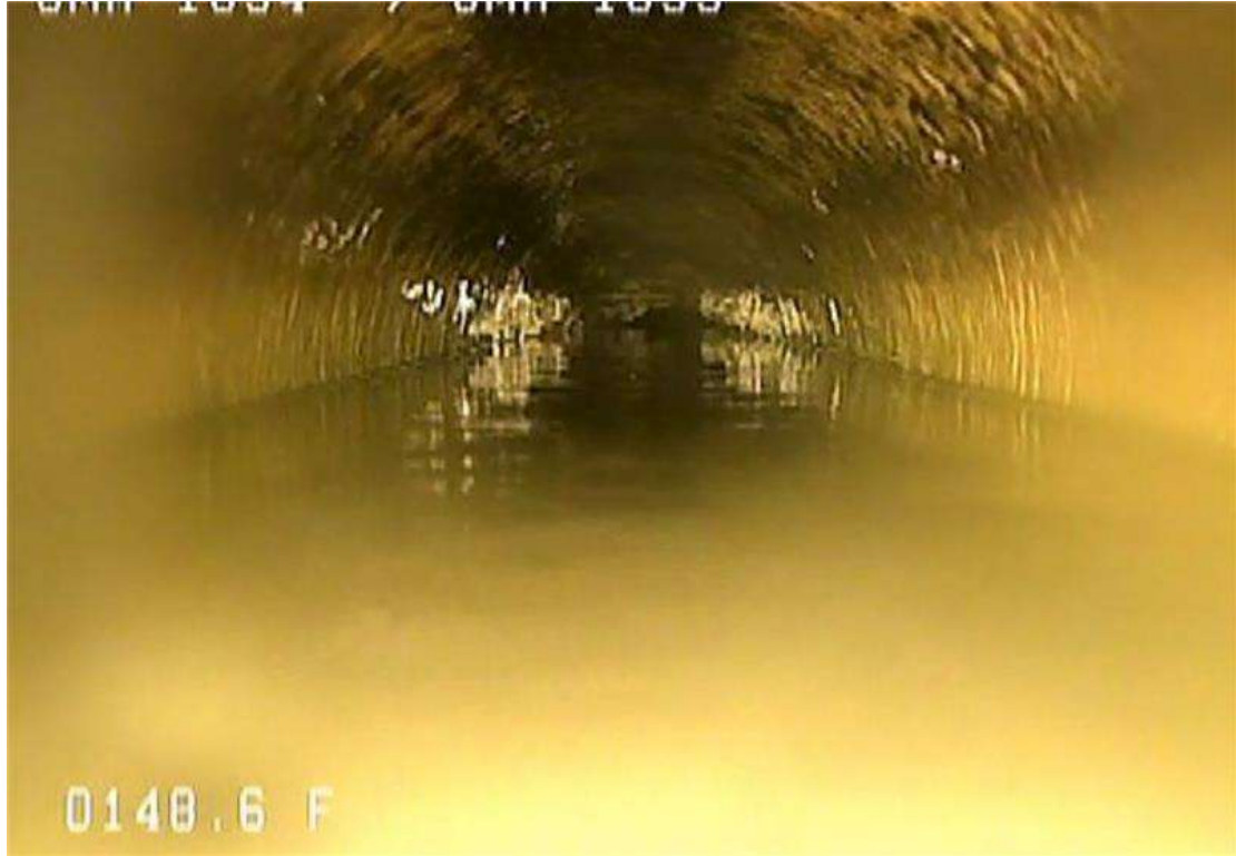
Photograph 3: Major pipe sag observed 145 linear feet downstream of SMH_1894
