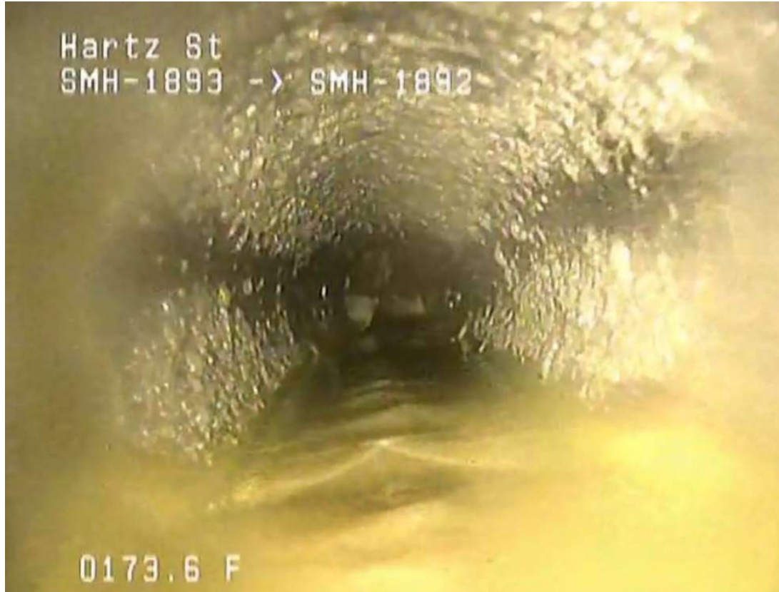
Photograph 4: Grease observed at the top of the pipe approximately 110 linear feet downstream of SMH_1893.
