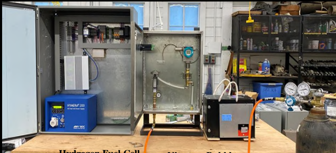
Hydrogen Fuel Cell
