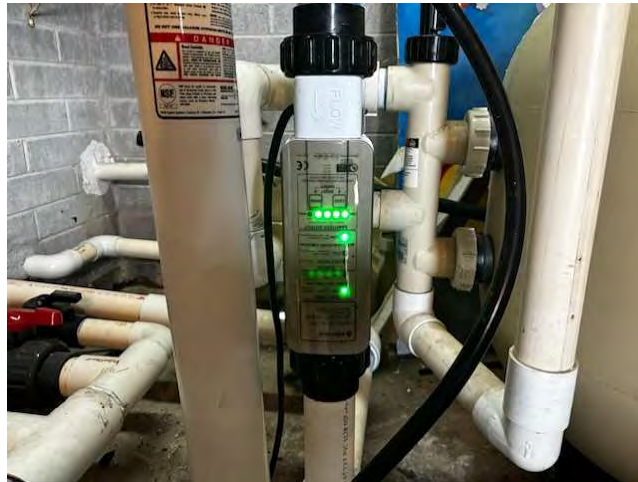
This is a Pentair, Intellichlor, salt cell that was installed in 7/2023. Current cost is $1,800.
