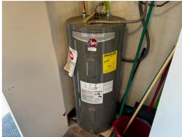
This is a Rheem, 40 gallon electric water heater (4/20/2017).
