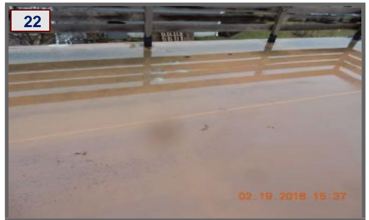
Pooling water noted on the low slope roof. (2)
