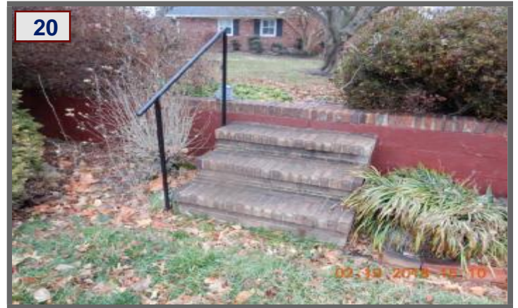
The rear steps have uneven rise and the railings are incorrect. (2) (4)
