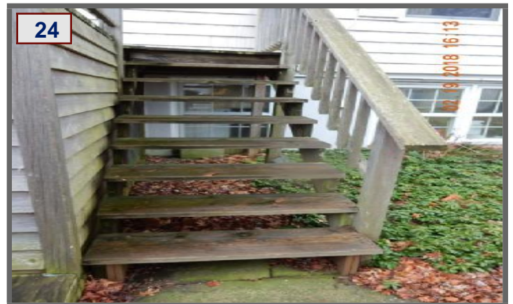
The rear deck steps are loose, the railings are too wide and rot was noted. (2)(4)
