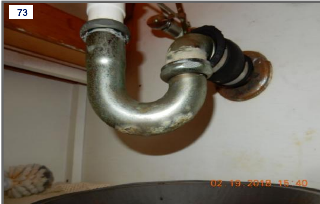
Lower Bathroom: Corroded drain trap noted. (2)
