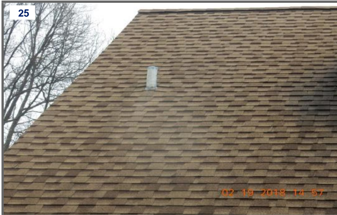
The flashing for the drain waste vent is incorrect. (2)
