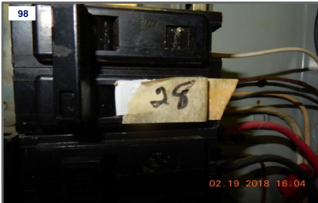
Over fusing, breaker size too large for wire at main electrical panel. (2) (4)
