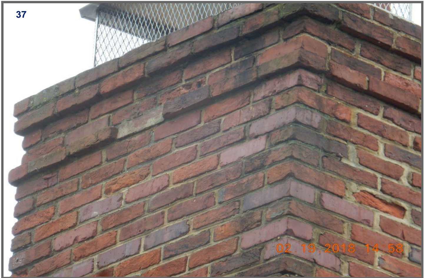
Spalling bricks noted on the chimney. (2)
