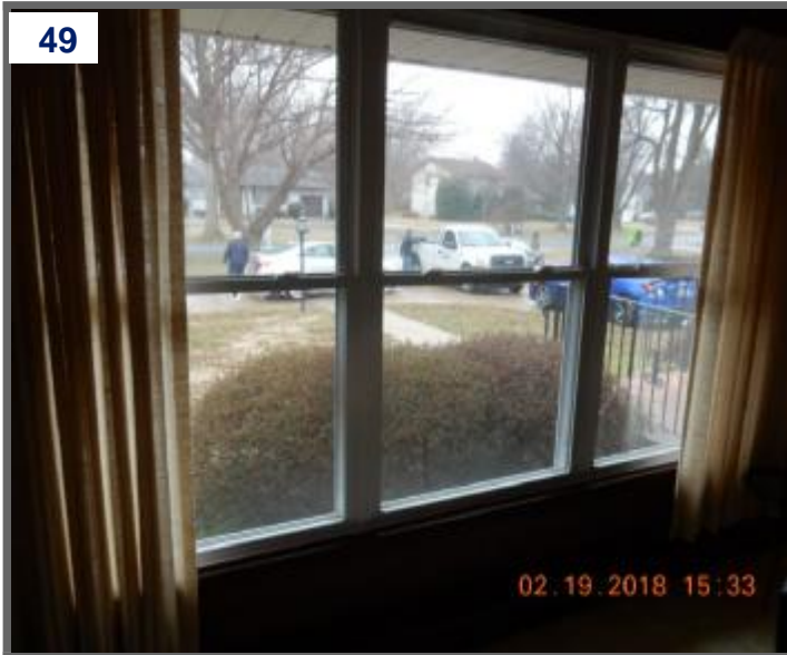
The front living room windows do not lock. (2)
