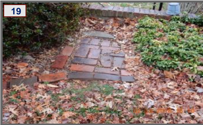
Pavers for sidewalks are a trip hazard. (2)(4)
