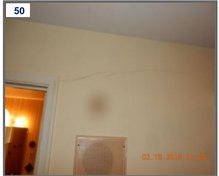
Unusual cracks noted around the doors at the jack and jill bathroom. (2)
