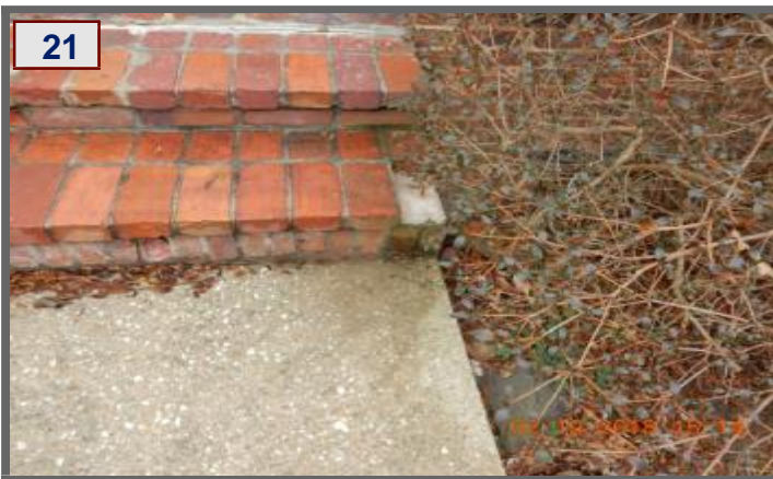
Missing bricks noted at the front entry steps. (2)(4) See
