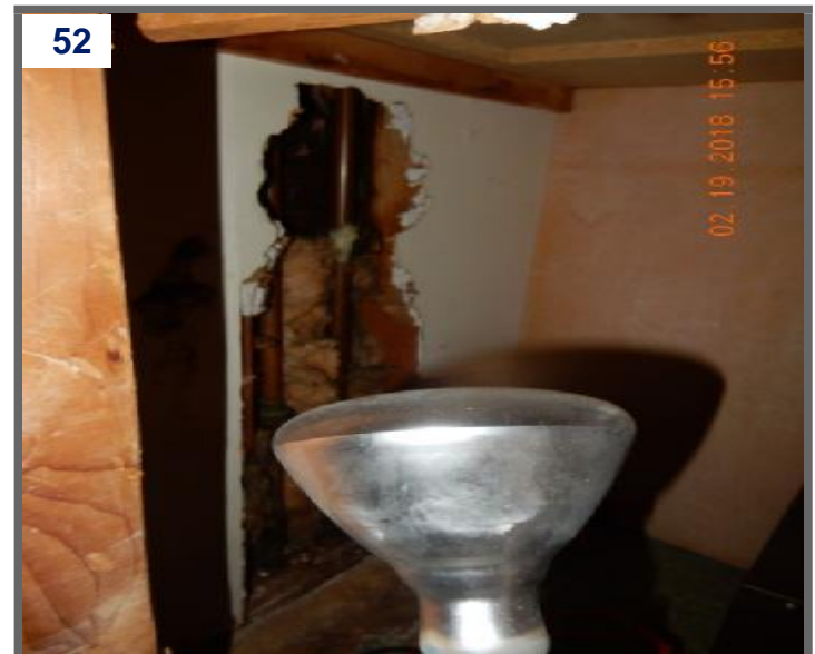
Evidence of freezing pipes noted at the lower level master bedroom closet. (2)
