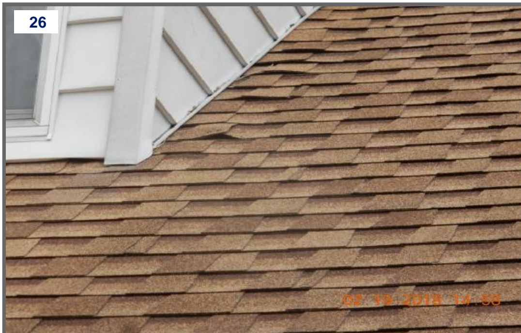
Appears to be some nail heads starting to pop up on roof, which is causing to raise at some locations. This is in the very early stages. Recommend addressing this in the near future. (2)
