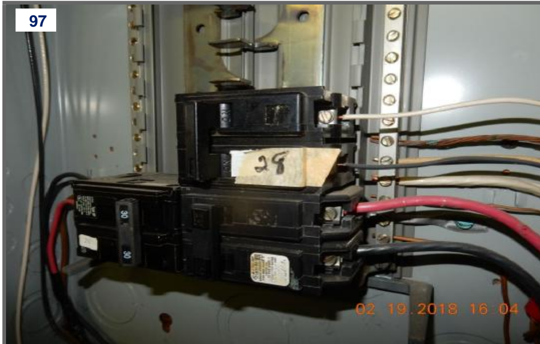
Over fusing, breaker size too large for wire at main electrical panel. (2) (4)
