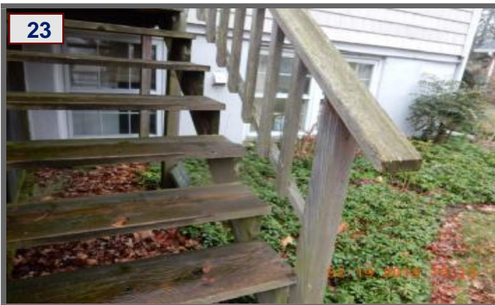
The rear deck steps are loose, the railings are too wide and rot was noted. (2)(4)
