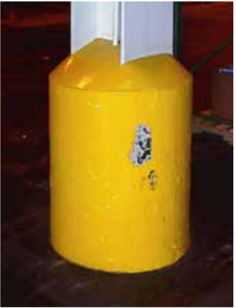
Damaged unprotected column
