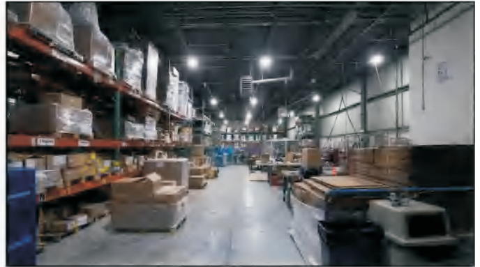
Production Area AFTER: 13 LED High Bays @ 160W each = 2,080 total watts = 74% Energy Savings, a much cleaner appearance, a better, more accurate color temperature, very even lighting - 55 to 65 footcandles everywhere, instant ON, and no heat or humming or flickering!
