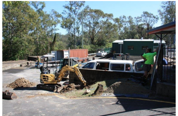
Construction work commences on the art centre, as a further development of the Kenmore Community Centre.
