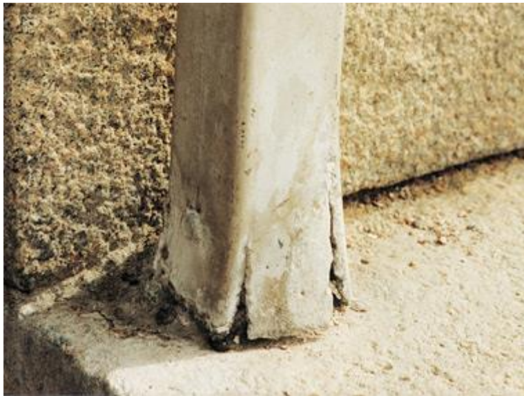
Close-up of galvanic corrosion in an aluminium rail post (25 year's use). The rectangular hollow profile was held in place by a carbon steel bolt. The contact surfaces between the steel and the aluminium were often wet and attack was aggravated by wintertime salting.
