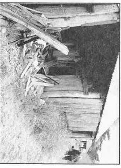
The original 'hut' that John and Bridget Guerin lived in until the house was built - originally it would have had a thatched roof.
