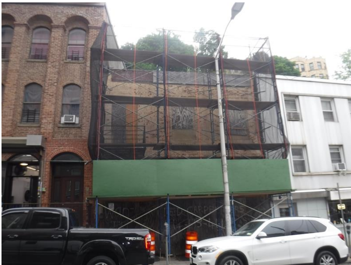
Photo 2: View of front face of building, showing plywood covering façade to prevent bricks from falling.
