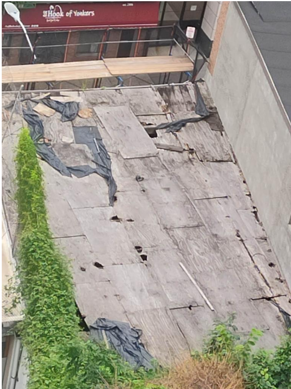
Photo 1: View of existing roof from above. No signs of any repair or shoring work can be seen.
