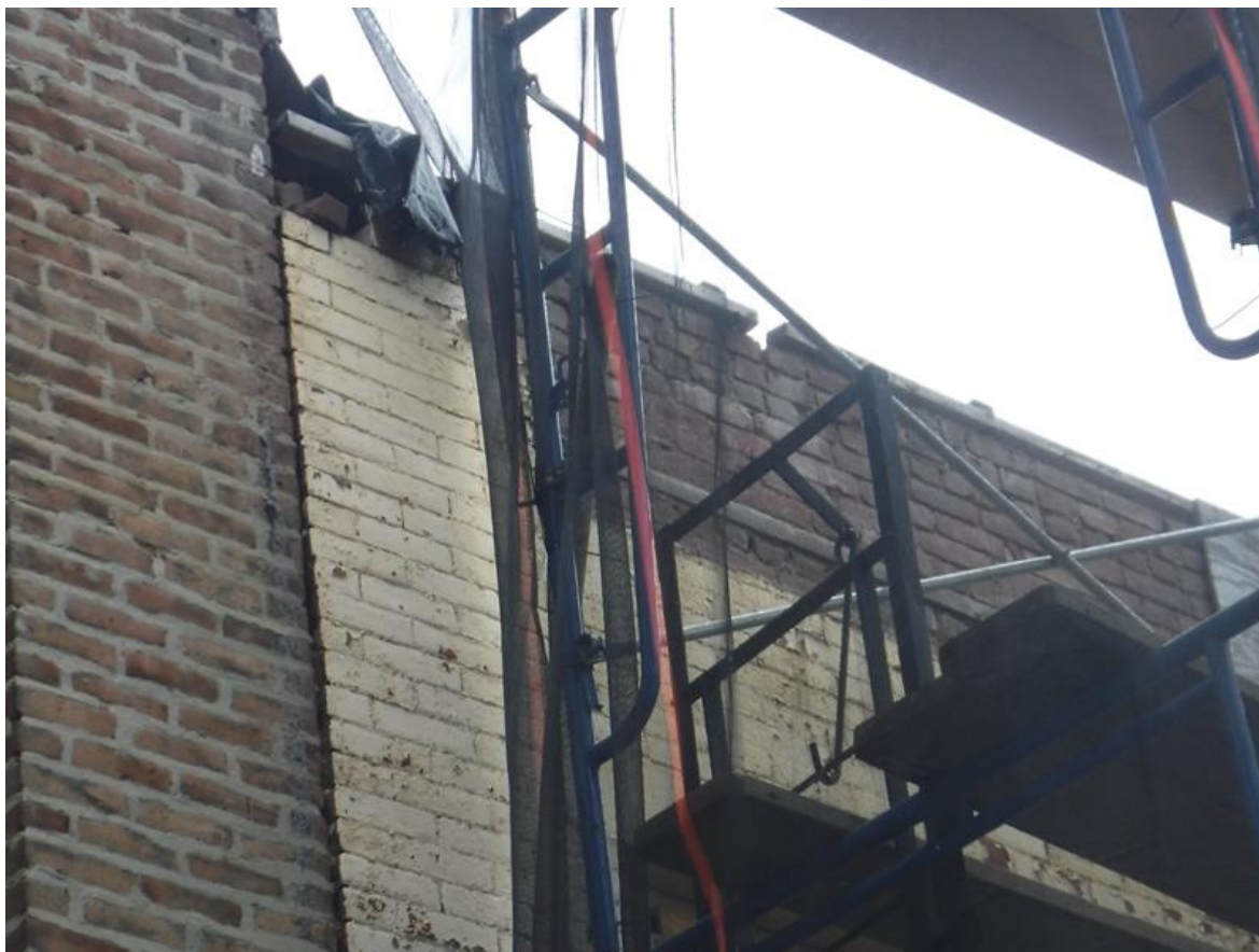
Photo 3: View of brick façade, showing missing bricks and mortar.
