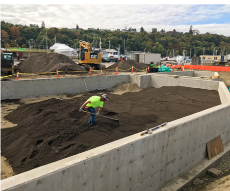
Stormwater vault. Photo by Sarah Burch
