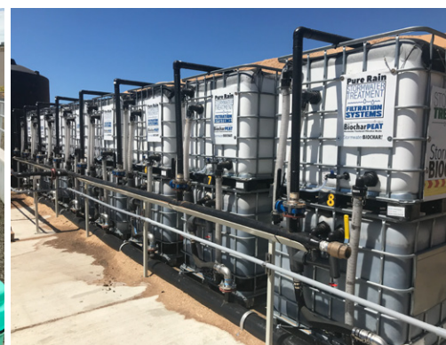
Stand alone filter system to filter metals from industrial sites. Photo by Ryan Holmann, Stormwater Biochar; filters by BioLogical Carbon
