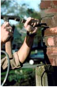
Here, a hammer and chisel are being correctly used to prepare a joint for repointing. Photo: John P. Spweik.
