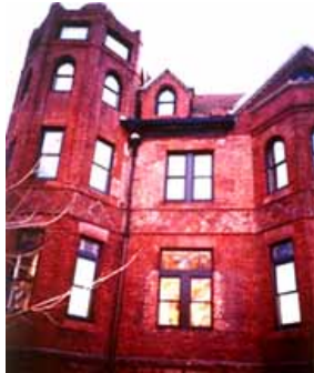
Unskilled repointing has negatively impacted the character of this late-19th century building. Photo: NPS files.
