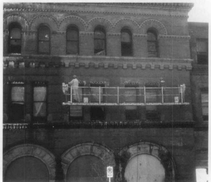
Figure 12. A mild acidic cleaning agent is being used to clean this heavily soiled brick and granite building. Additional applications of the cleaner and hand-scrubbing, and even poulticing, may be necessary to remove the dark stains on the granite arches below. Photo: Sharon C. Park, FAIA.
