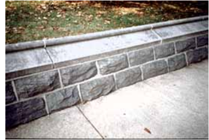
Caulking was inappropriately used here in place of mortar on the top of the wall. As a result, it has not been durable. Photo: NPS files.
