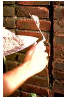
This mortar is the proper consistency for repointing historic brick. Photo: John P. Speweik.
