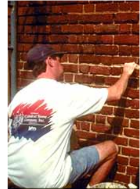
This early 19th century building is being repointed with lime mortar. Photo: Travis McDonald.
