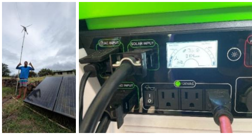
Fig.11: Off-grid Plug-n-Play solar-battery generator with wind turbine.
