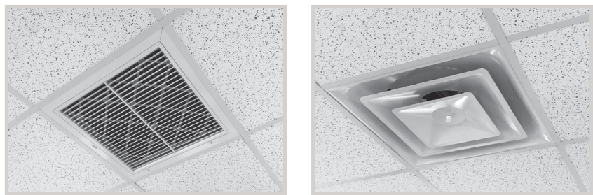
Return grill attached to filter assembly
