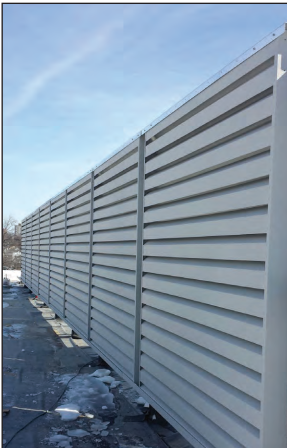
Rooftop Louvered Equipment Barrier
