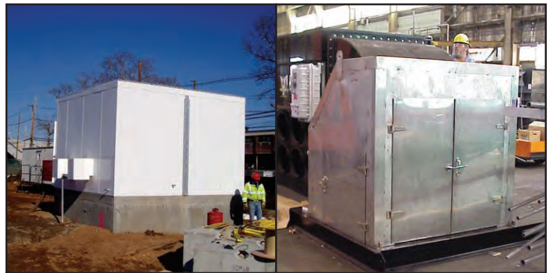
Air Compressor Enclosure
