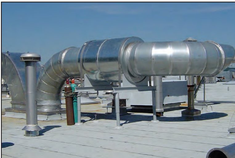
Roof Top Factory Exhaust Silencer
