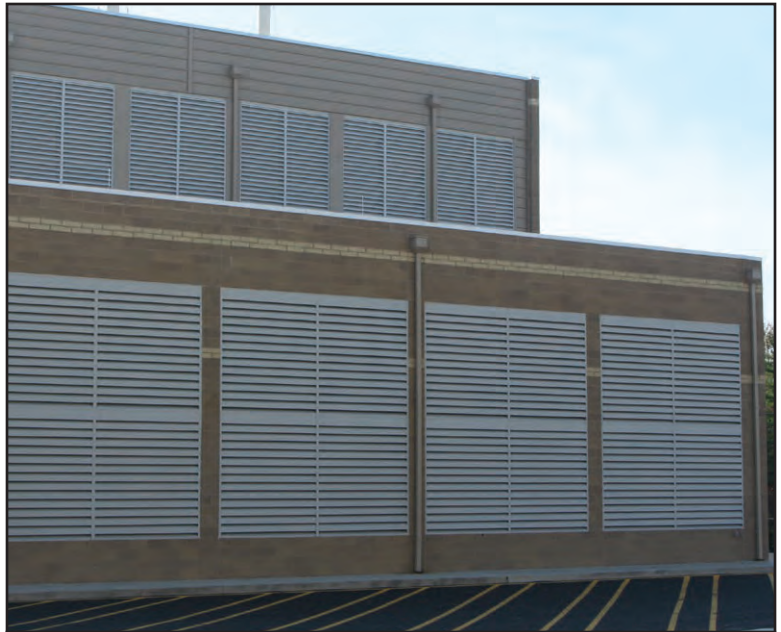
Central Energy Plant Louvers
