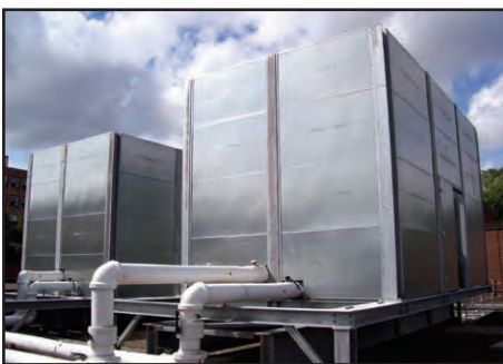
Roof Top Chiller Barrier Wall
