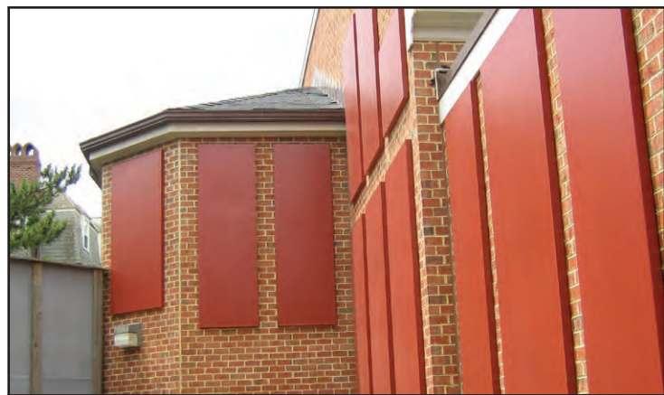
Chiller Yard Wall Absorption Panels
