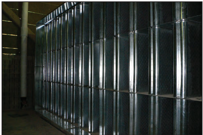
Generator Room Intake Silencer Bank
