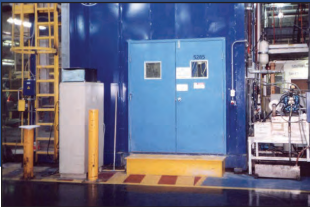
In-Plant Equipment Enclosure
