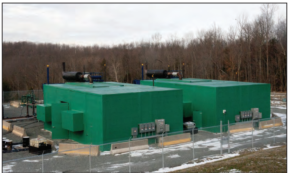
Midstream Compressor Buildings
