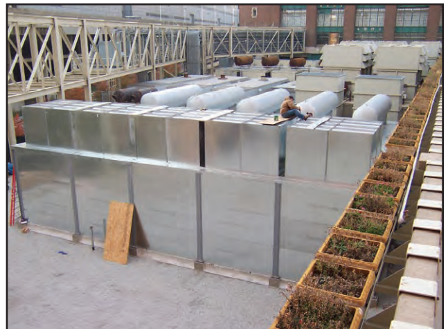
Multiple Generator Enclosure
