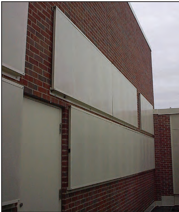
Equipment Yard Absorption
