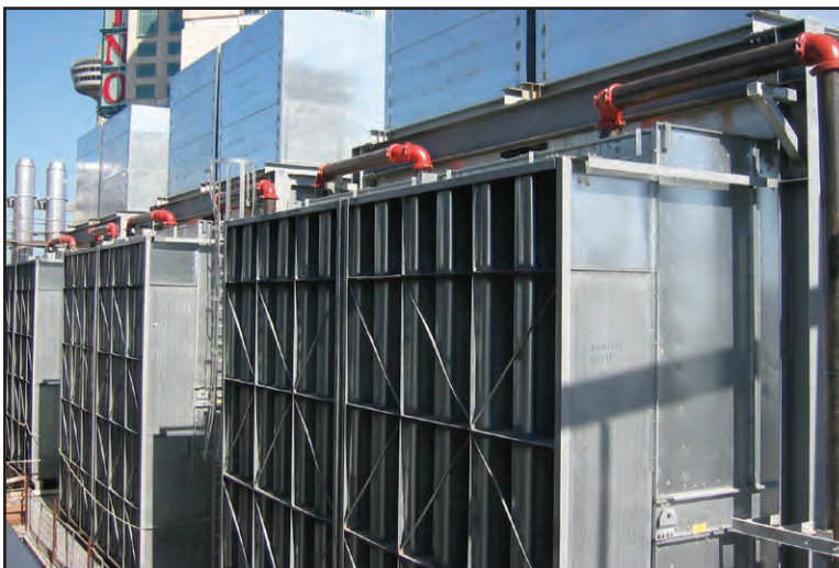
Cooling Tower Inlet and Discharge Silencers
