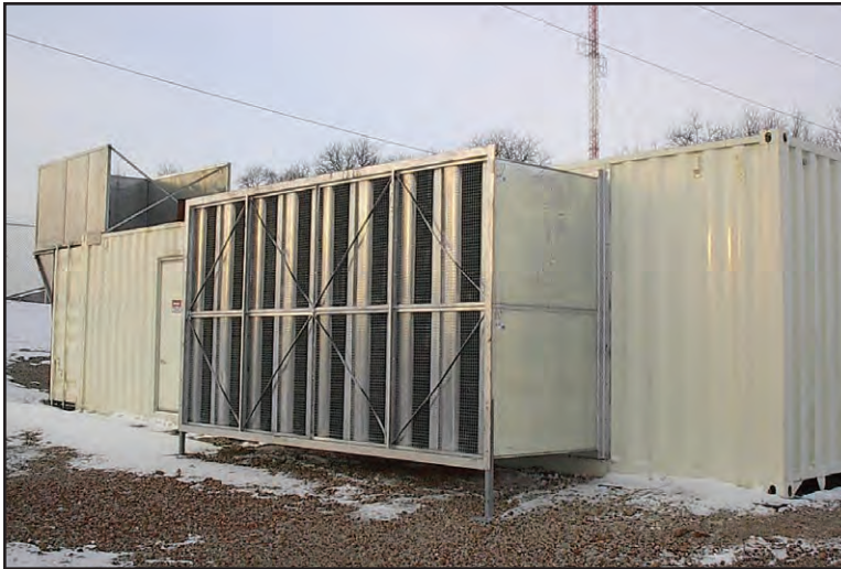
Generator Enclosure Ventilation Silencers
