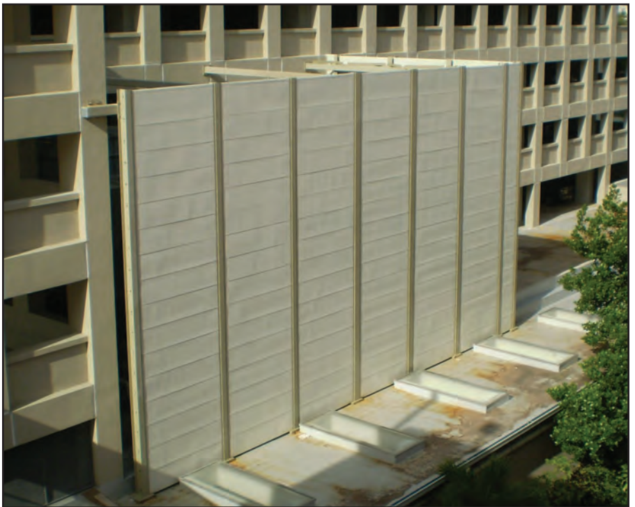
Cooling Tower Barrier Wall System
