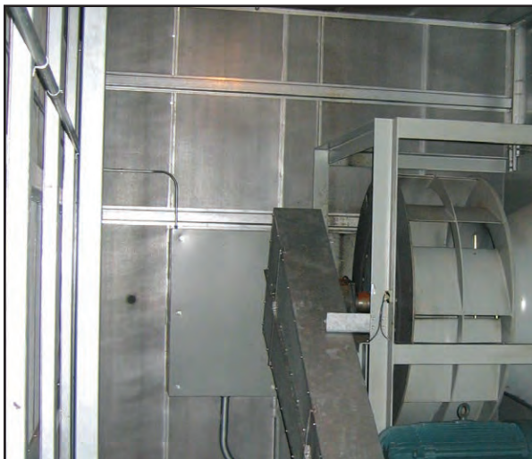
AHU Plenum Interior
