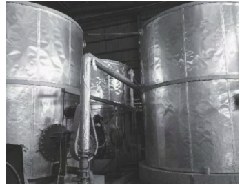
Small paper-plastic pulping system-dry and wet pressing demonstration line
