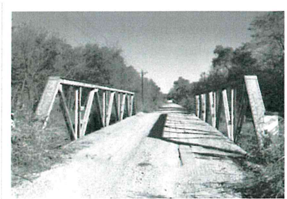
Functionally Obsolete: Single lane on Salt Creek Bridge, Seminole County OK
