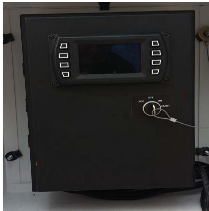
Heater Control Panel
