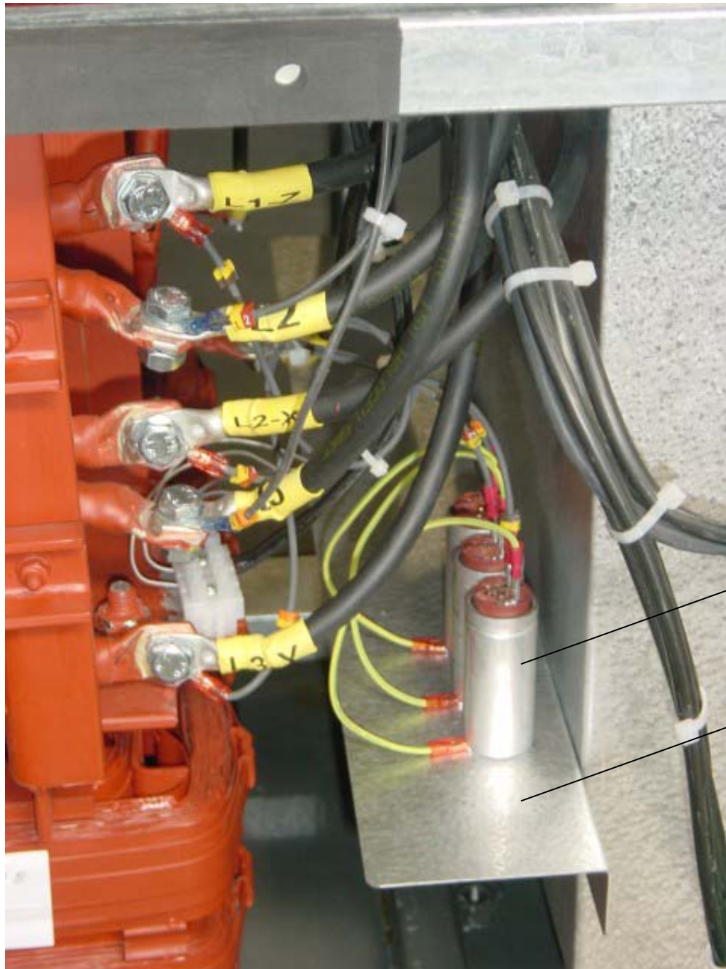
DC Filter Capacitor Bank Assembly Figure 8
