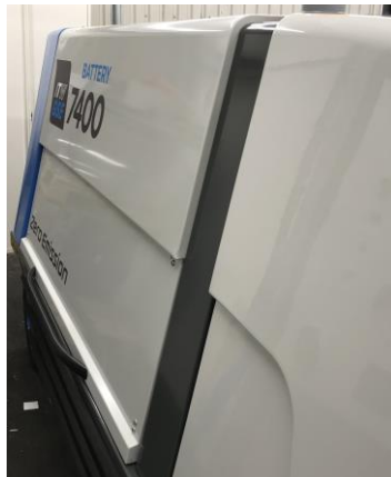
Fig 3.2.1b Cable Compartment, 50/60 Hz (closed)
