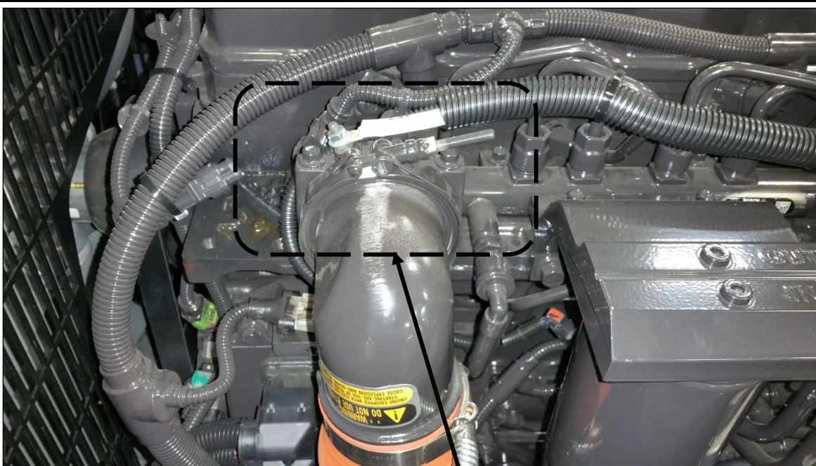
Air Intake Heater
