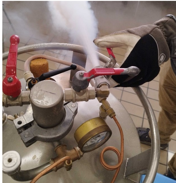
Figure 7.2 - Image of the valve opened.
