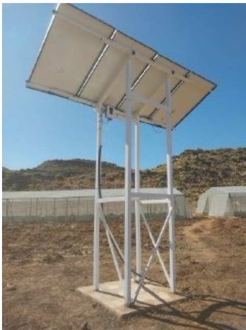
Fig. 7: Solar pump at Lithakaling.
