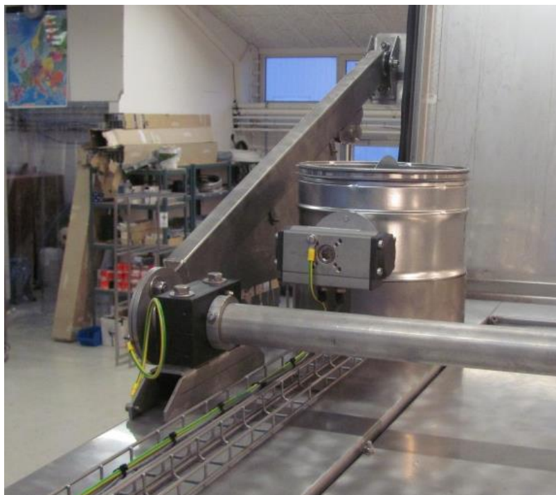
Fig. 3.5 Automatic ventilation damper
