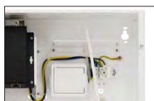
Shelf for DVR power supply unit, 230VAC socket
