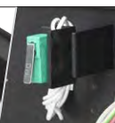
Tamper indicating patch panel opening
