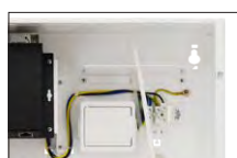
Shelf for NVR power supply unit, 230VAC socket
