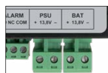
– Connector of the charging circuit – Battery connectors
