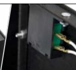
Tamper switch detecting enclosure opening
