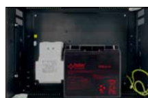
Mounting plate – for mounting transformer + place for battery
