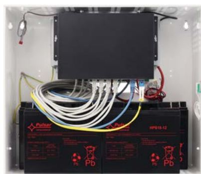
IP receivers Data + power supply 52 V DC
