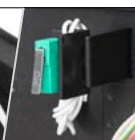
Tamper switch indicating front panel opening
