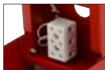
Porcelain screw connection in cabinet
