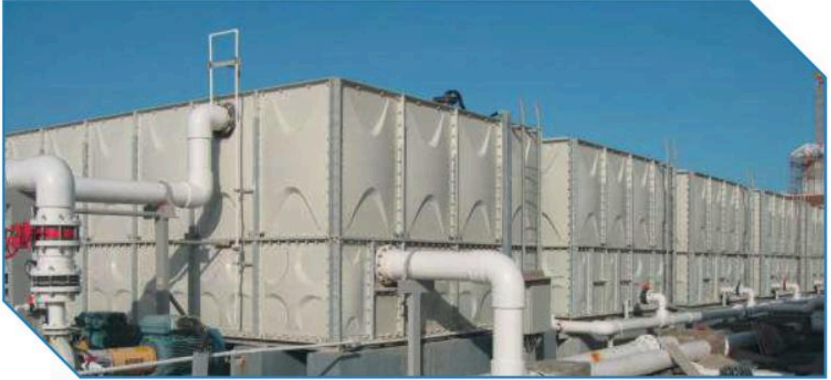
Basra / Özel Arıtma Tesisi (İRAK) - 100 ton Basra / Special Treatment Plant (IRAQ) - 100 ton
