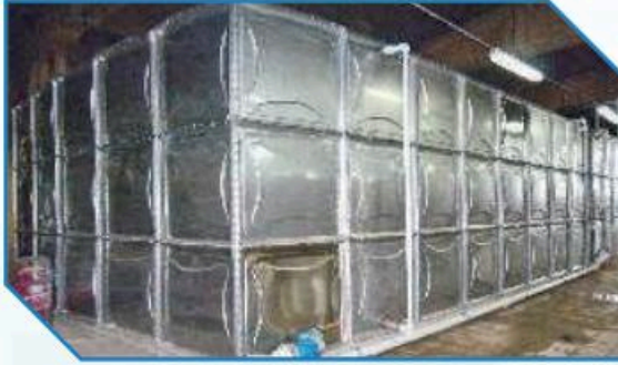
Urfa TOKİ Hastane Su Deposu (TÜRKİYE) - 150 ton Urfa TOKİ Hospital Water Tank (TURKEY) - 150 ton
