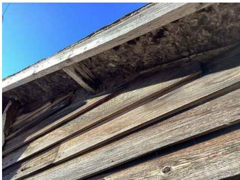
Poor Condition of Siding and Fascia
