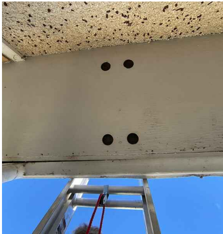
Ventilation in soffits is limited
