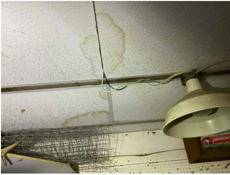
Signs of Past Water Damage
