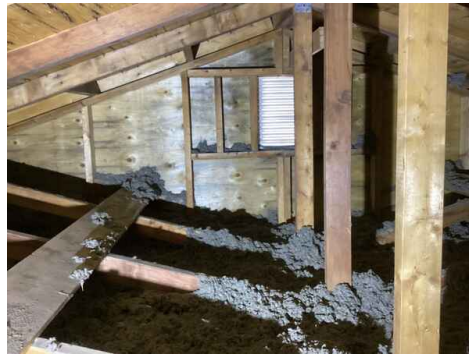
North Gable Vent
