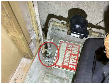
Main Water Shut Off Location
