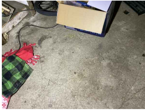
Concrete Flooring showing cracks
