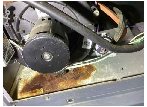
Evidence of Condensation
