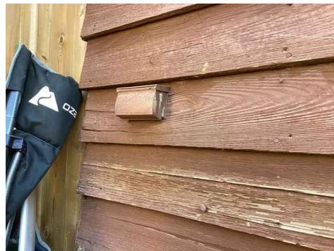
GFCI Receptacle not Operational
