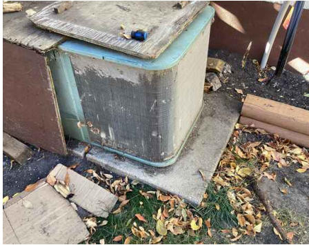
Air Cooled Condenser
