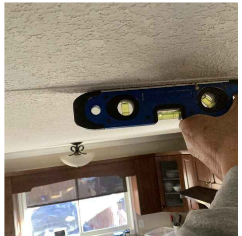
Ceiling Out of Level
