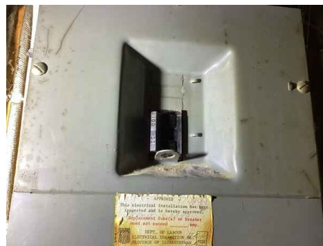
100 Amp Incoming Breaker
