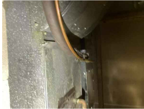
Refrigerant piping to Coil in Furnace
