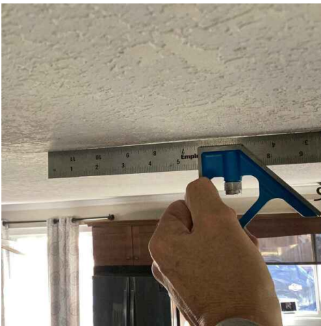
Ceiling is not level in area of concern
