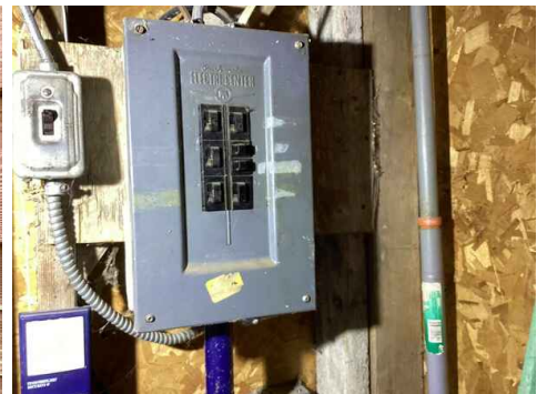
30 Amp Service from House Breaker Panel
