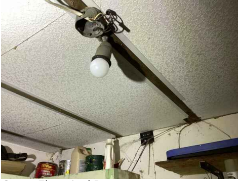
Open Electrical Box
