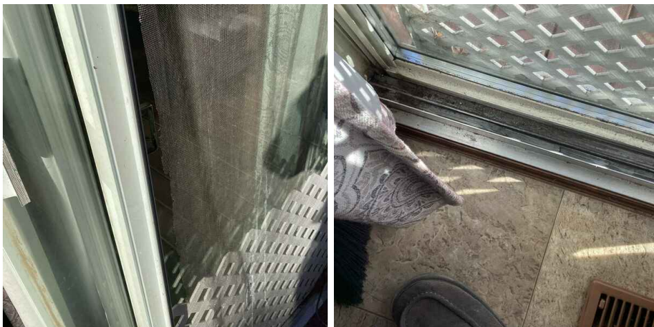
Screen repair required
