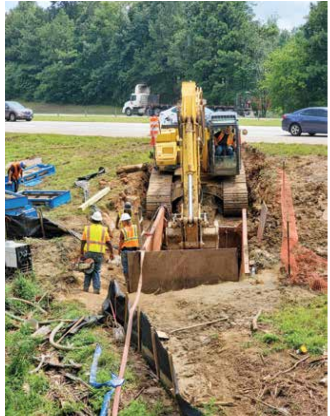
The existing trunk main was being upsized for capacity reasons. Bursting took approximately 1 hour and 30 minutes to complete
