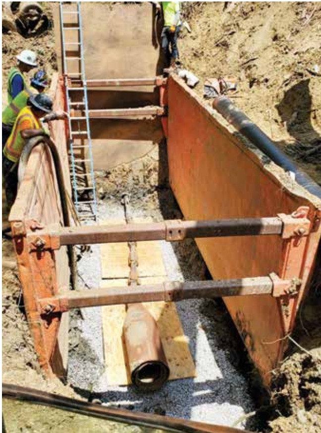
Bursting ductile iron pipe has become more prevalent with static pipe bursting systems. Special bladed rollers are needed to properly split the difficult pipe material
