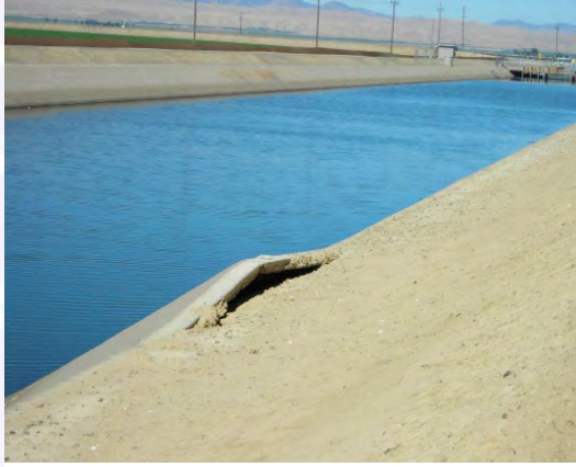
San Joaquin Valley subsidence causes buckling in an aqueduct as one type of water usage affects another
