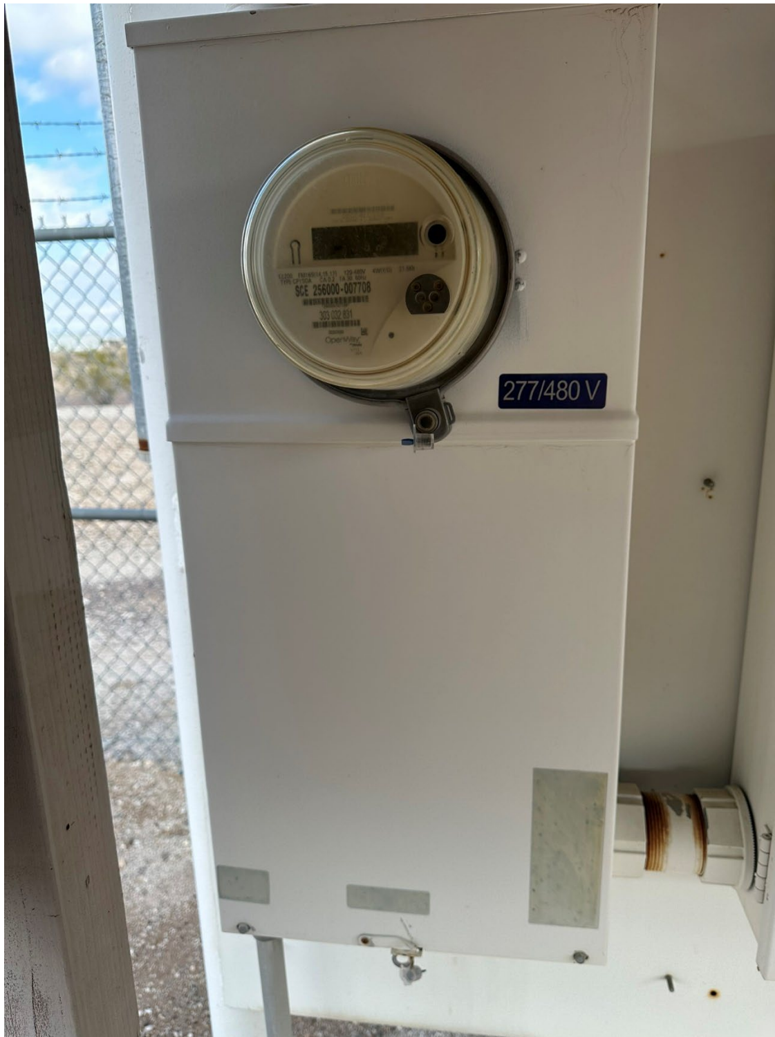
Figure 8: Well Meter and Meter Socket – East Well Site
