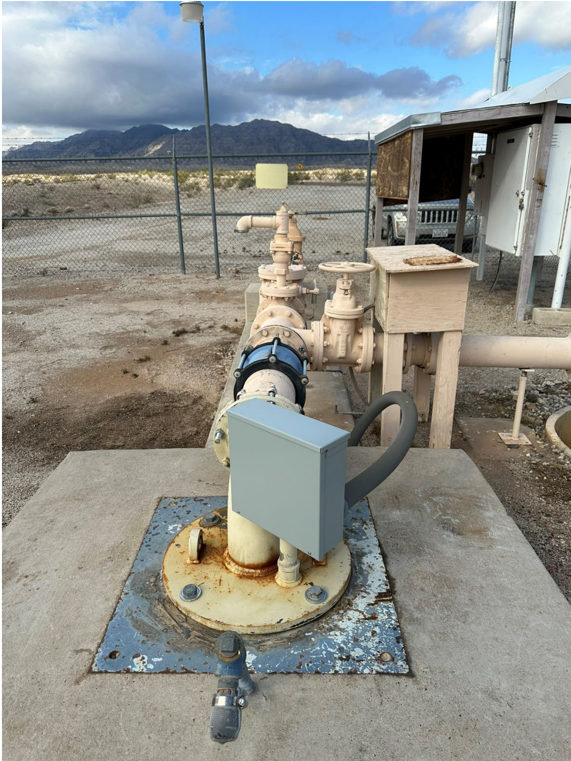
Figure 3: Close up of Well Head – East Well Site
