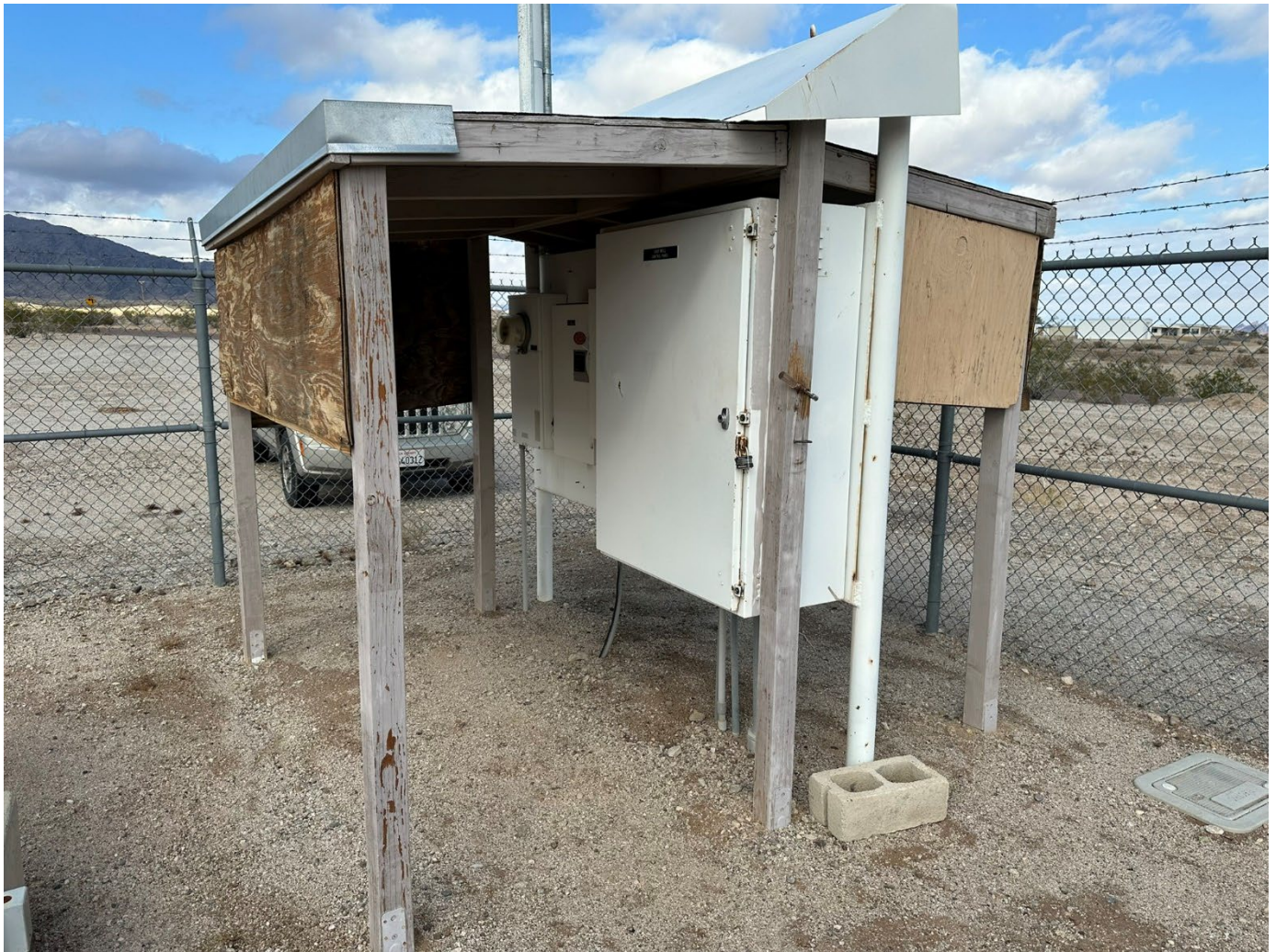
Figure 5: Overview of Well Controls and Shade Control Structure – East Well Site
