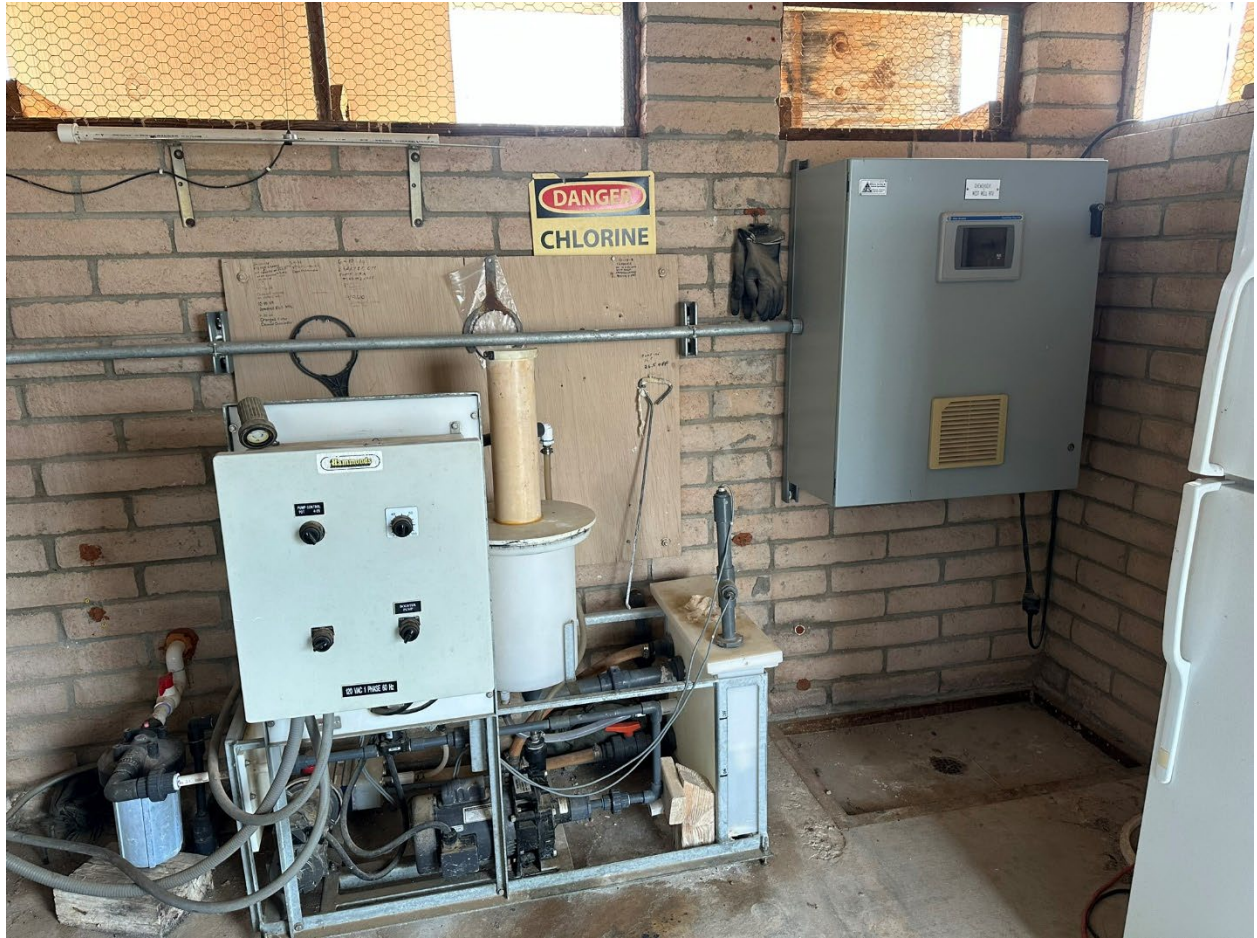
Figure 30: View #2 of Chlorinator System – West Well Site
