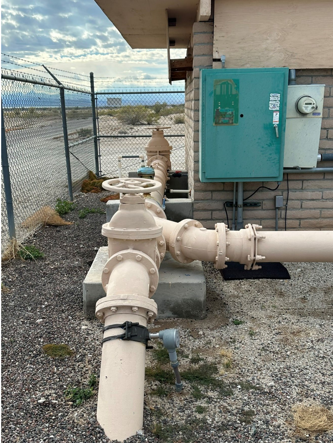
Figure 19: View of Plumbing Tree Behind Pumphouse - West Well Site
