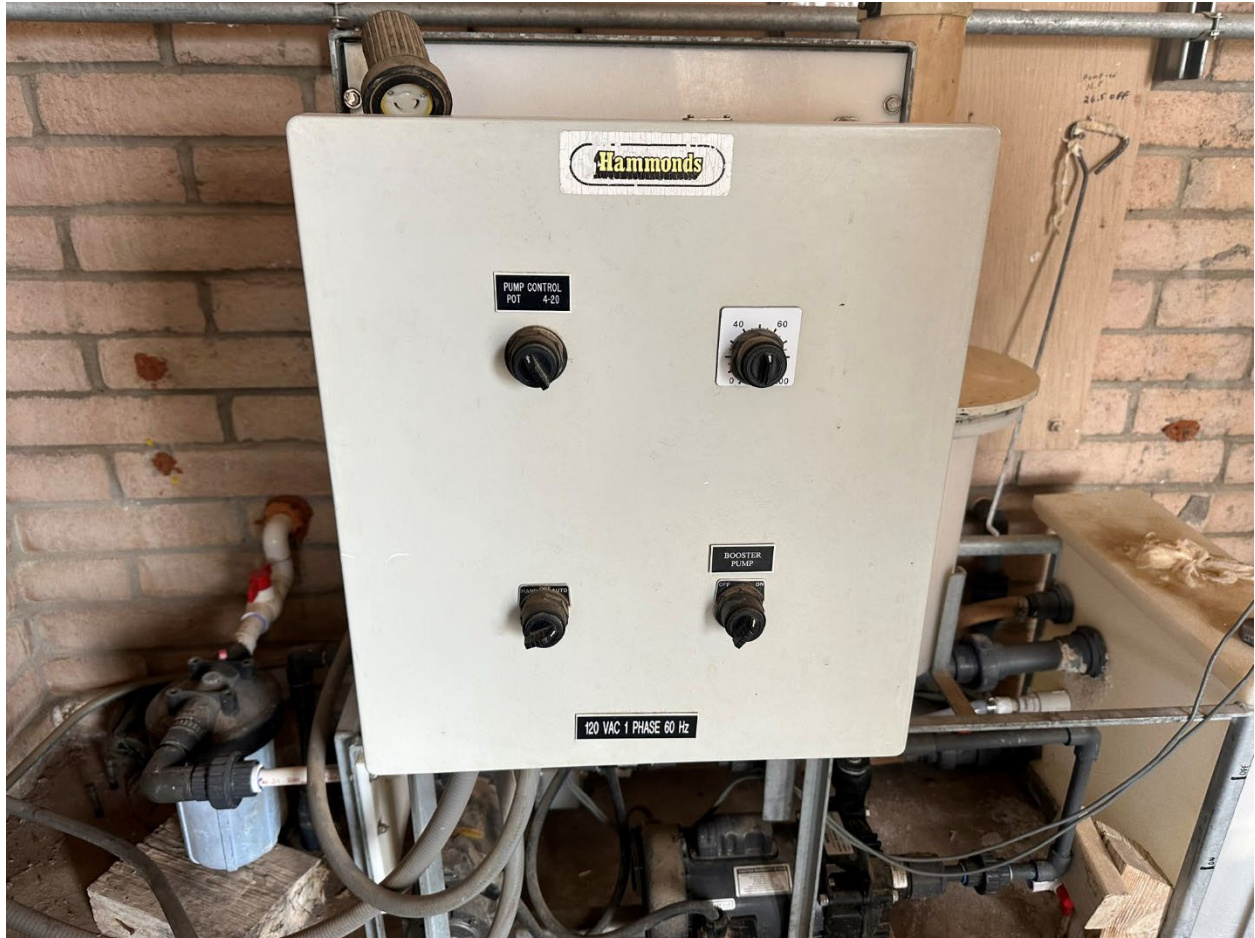
Figure 33: Chlorinator Pump Controls – West Well Site
