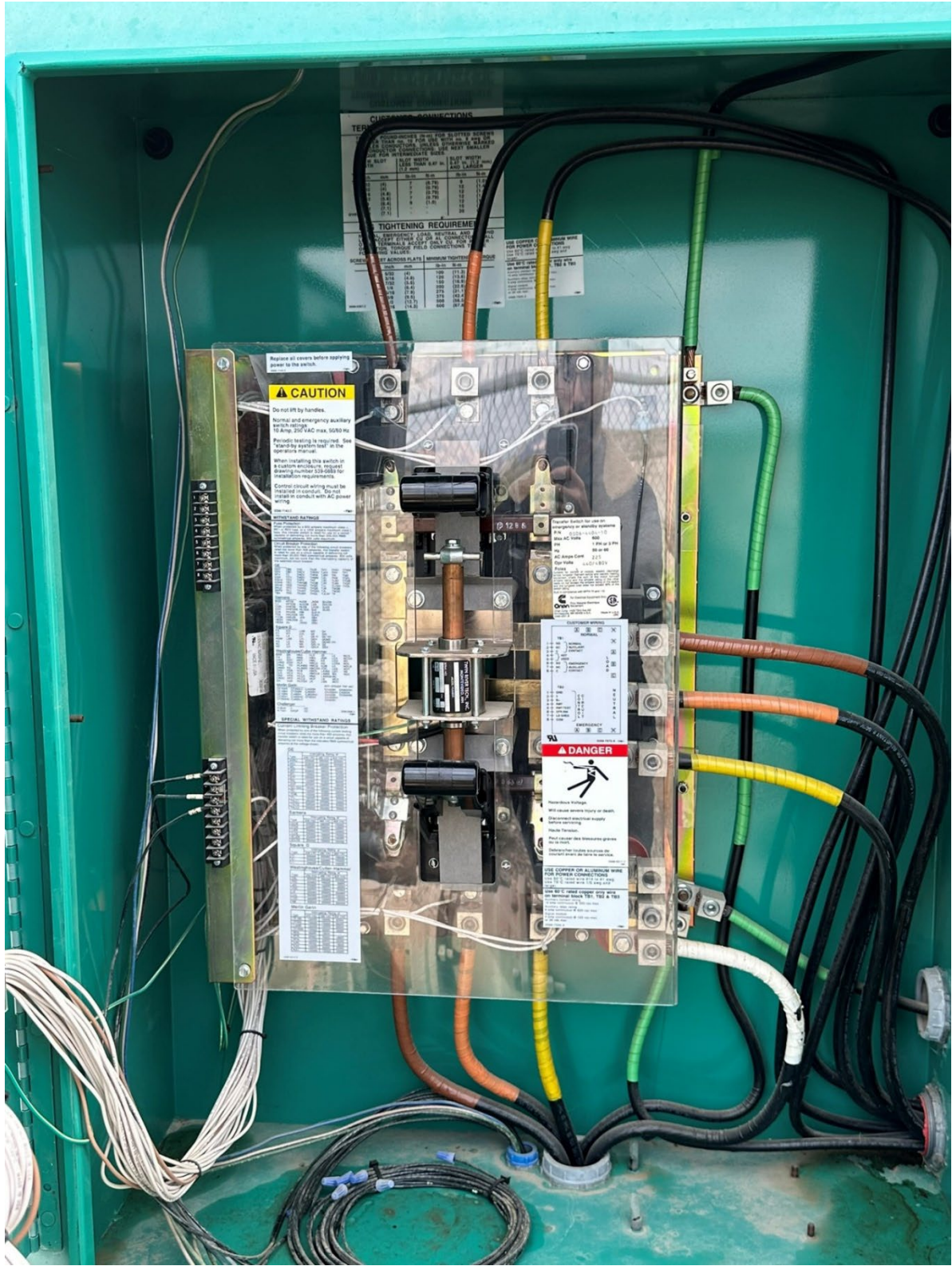
Figure 24: Inside View of Power Source #1 – West Well Site
