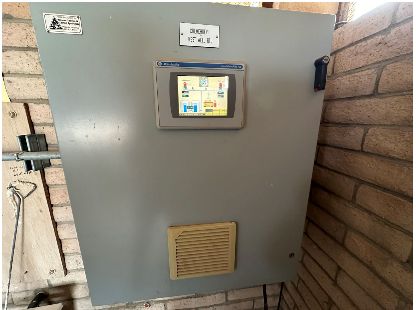
Figure 40: Well RTU – West Well Site
