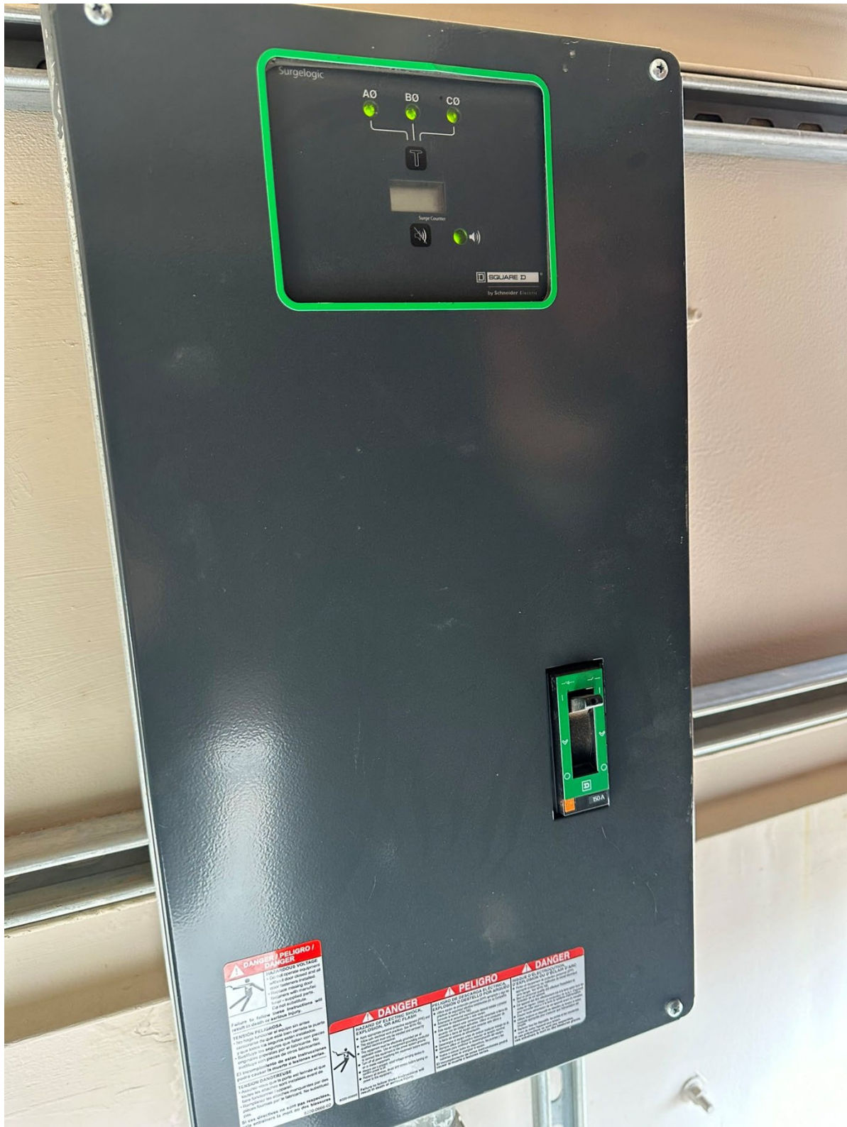
Figure 10: Well Surge Protection Device – East Well Site
