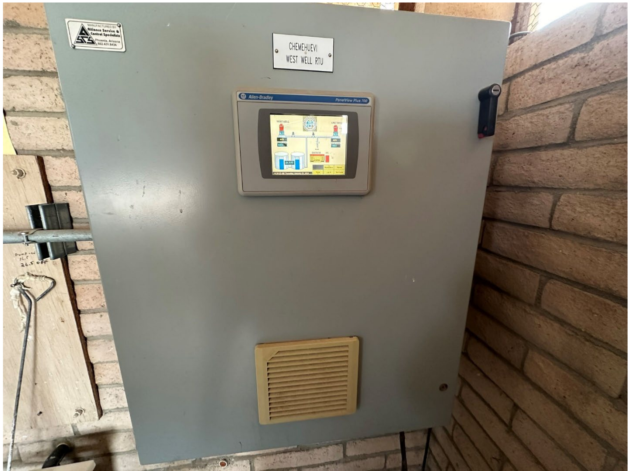
Figure 31: Well RTU – West Well Site
