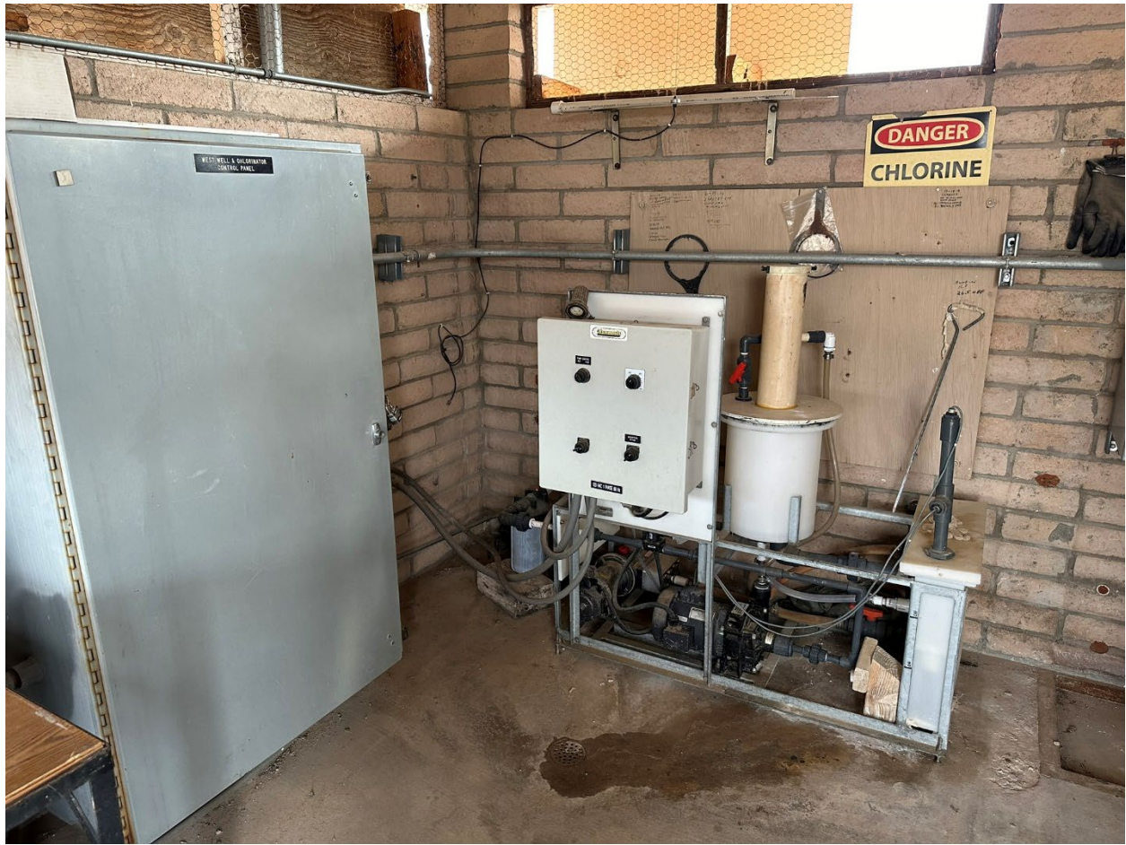
Figure 29: View #1 of Chlorinator System – West Well Site
