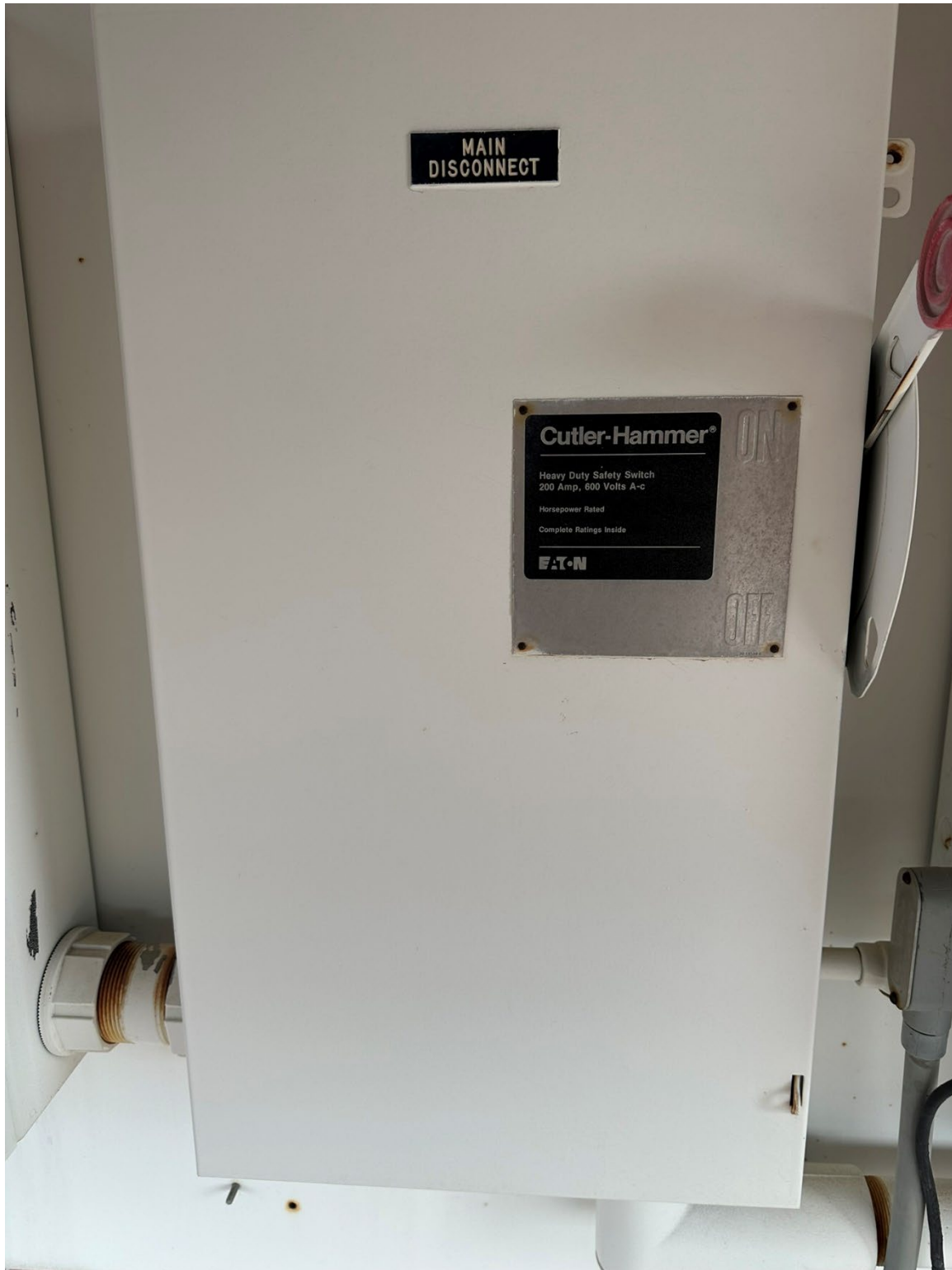
Figure 13: Well Main Disconnect – East Well Site
