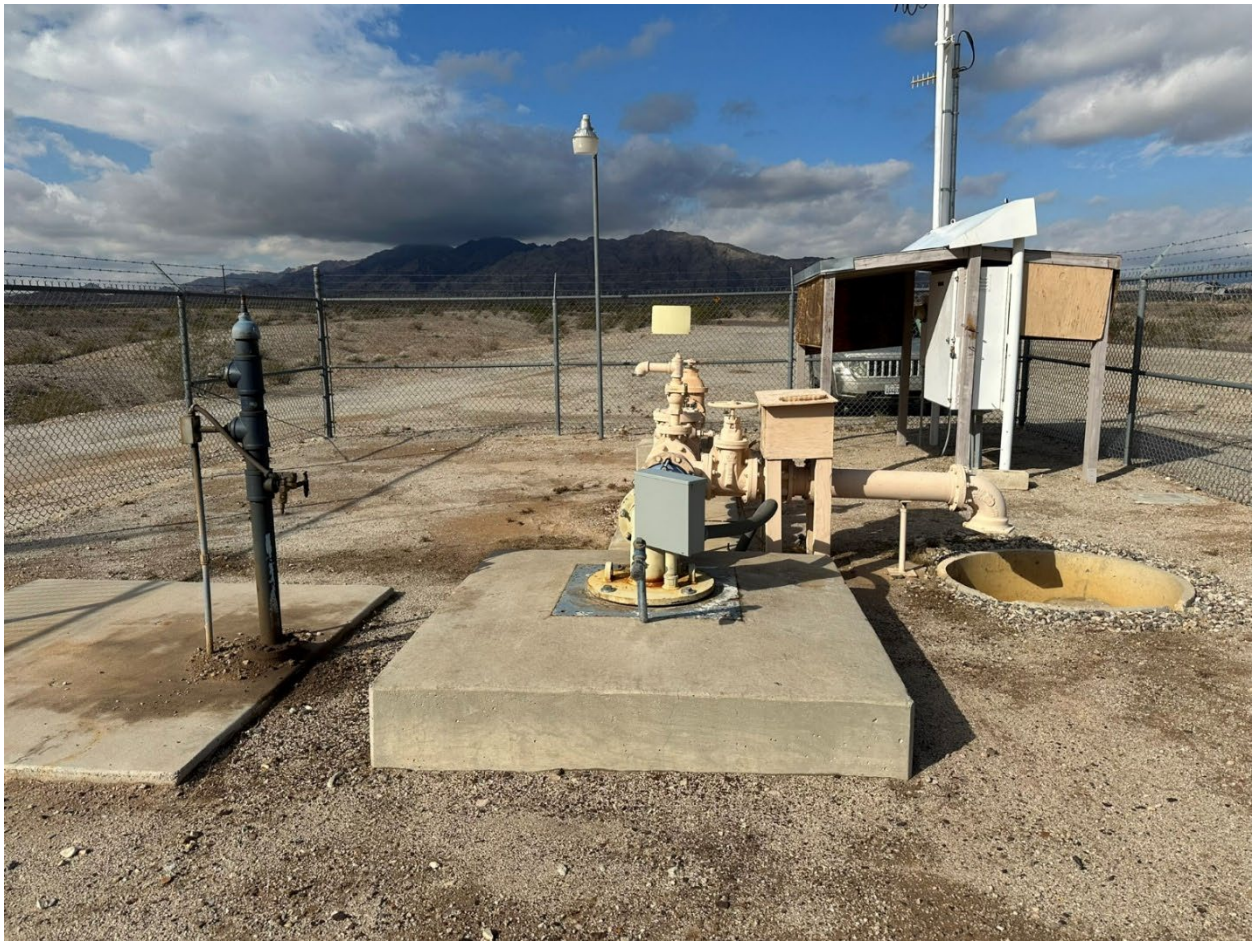
Figure 2: View of Plumbing Tree from the Northwest – East Well Site
