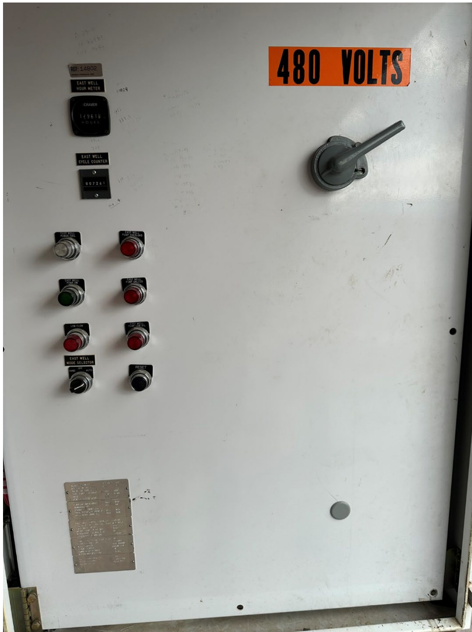
Figure 7: Well pump status indicator, mode select, and reset – East Well Site
