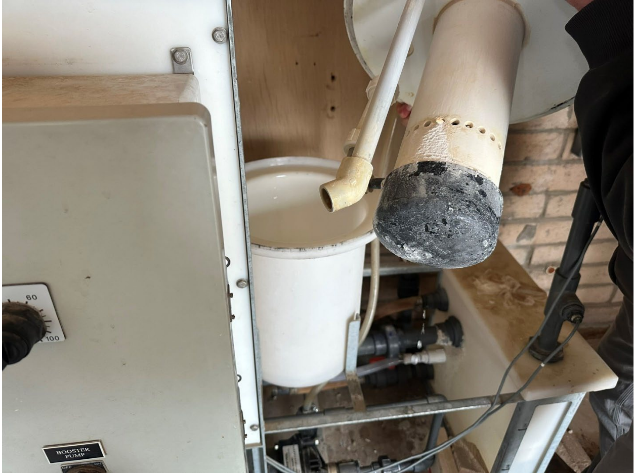
Figure 34: Broken Feeder Tube – West Well Site
