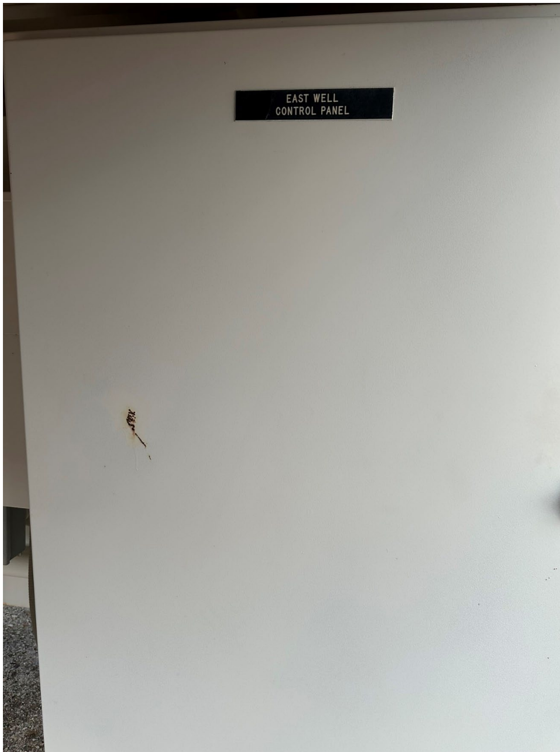
Figure 6: Well Control Panel – East Well Site
