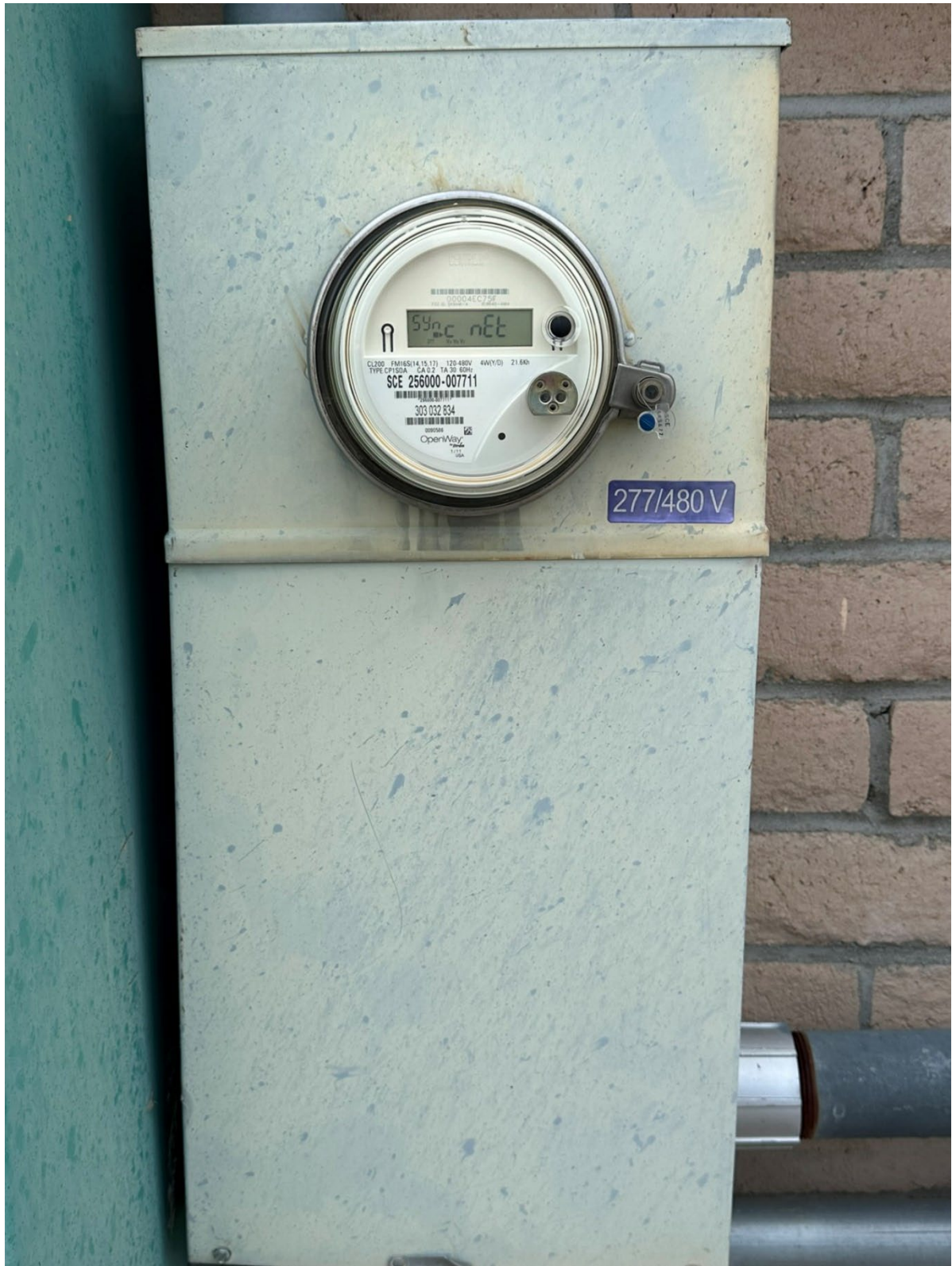
Figure 28: Electrical Meter – West Well Site
