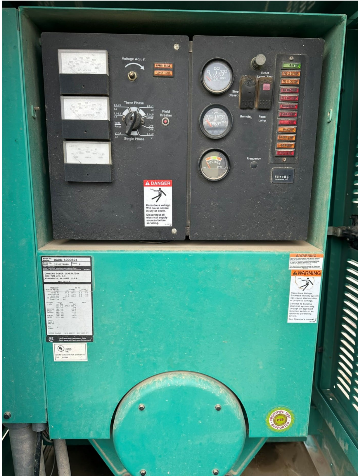
Figure 22: View of Generator Controls – West Well Site
