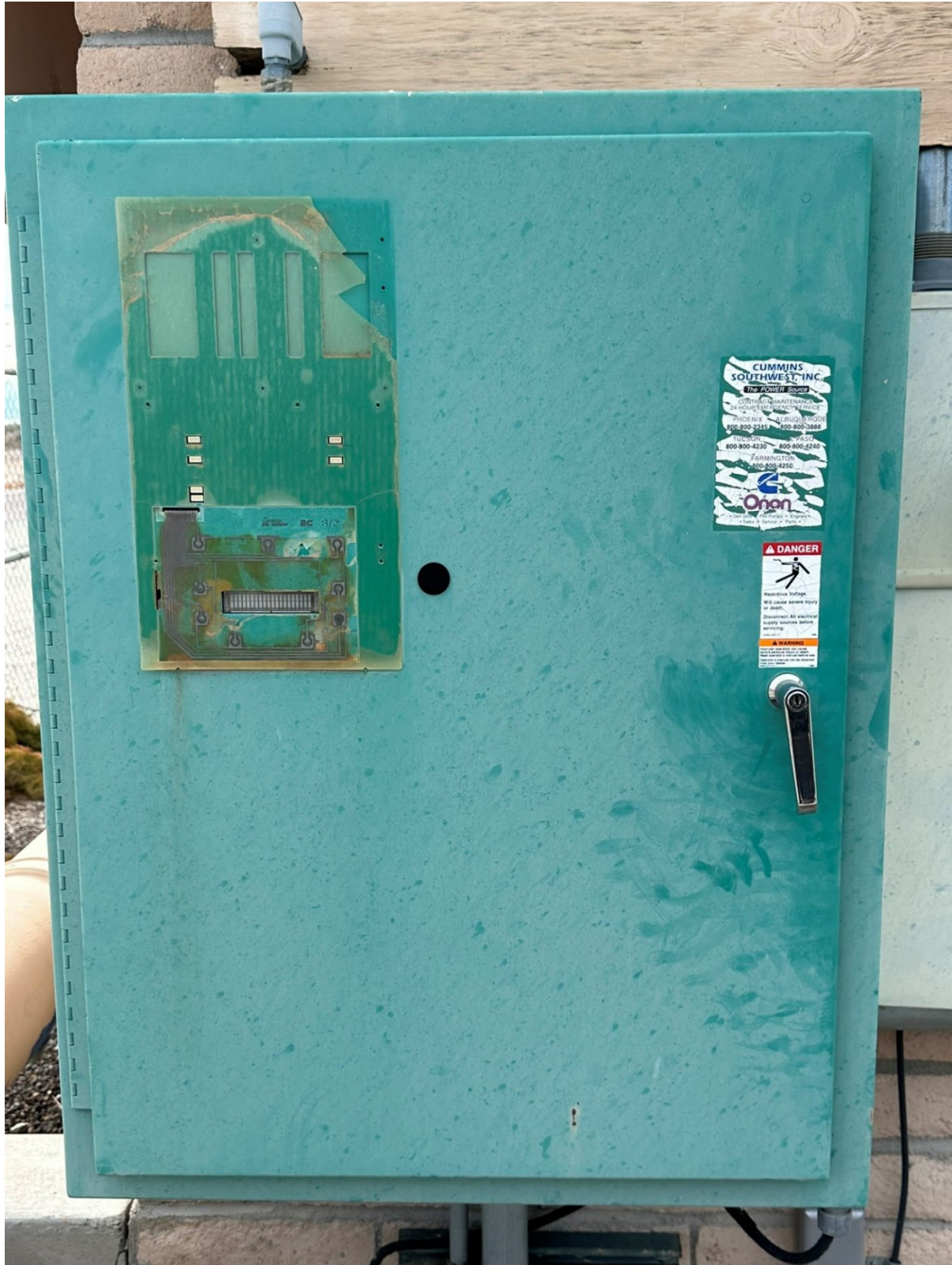
Figure 23: Power Source – West Well Site
