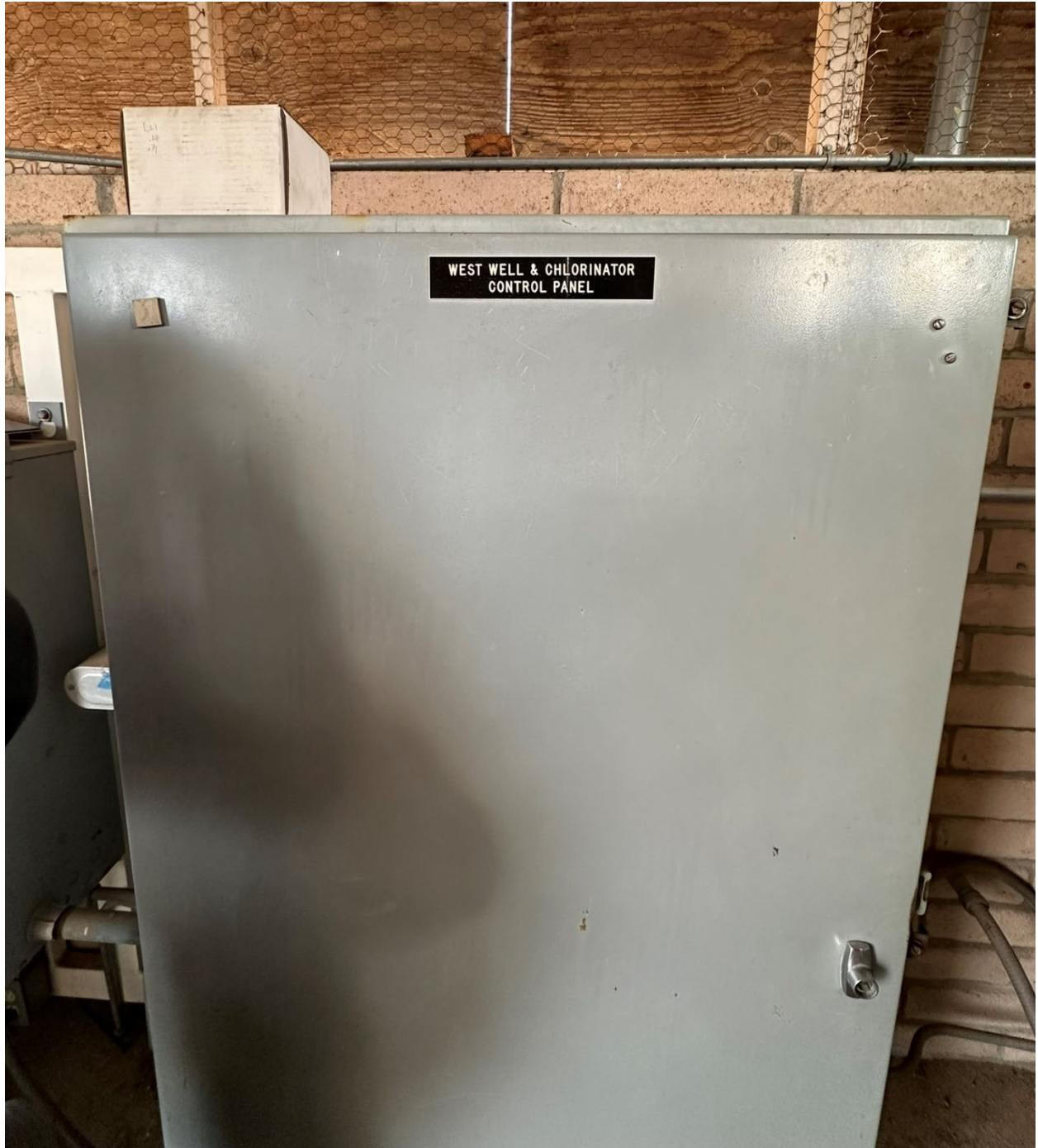
Figure 42: Well and Chlorinator Control Panel – West Well Site
