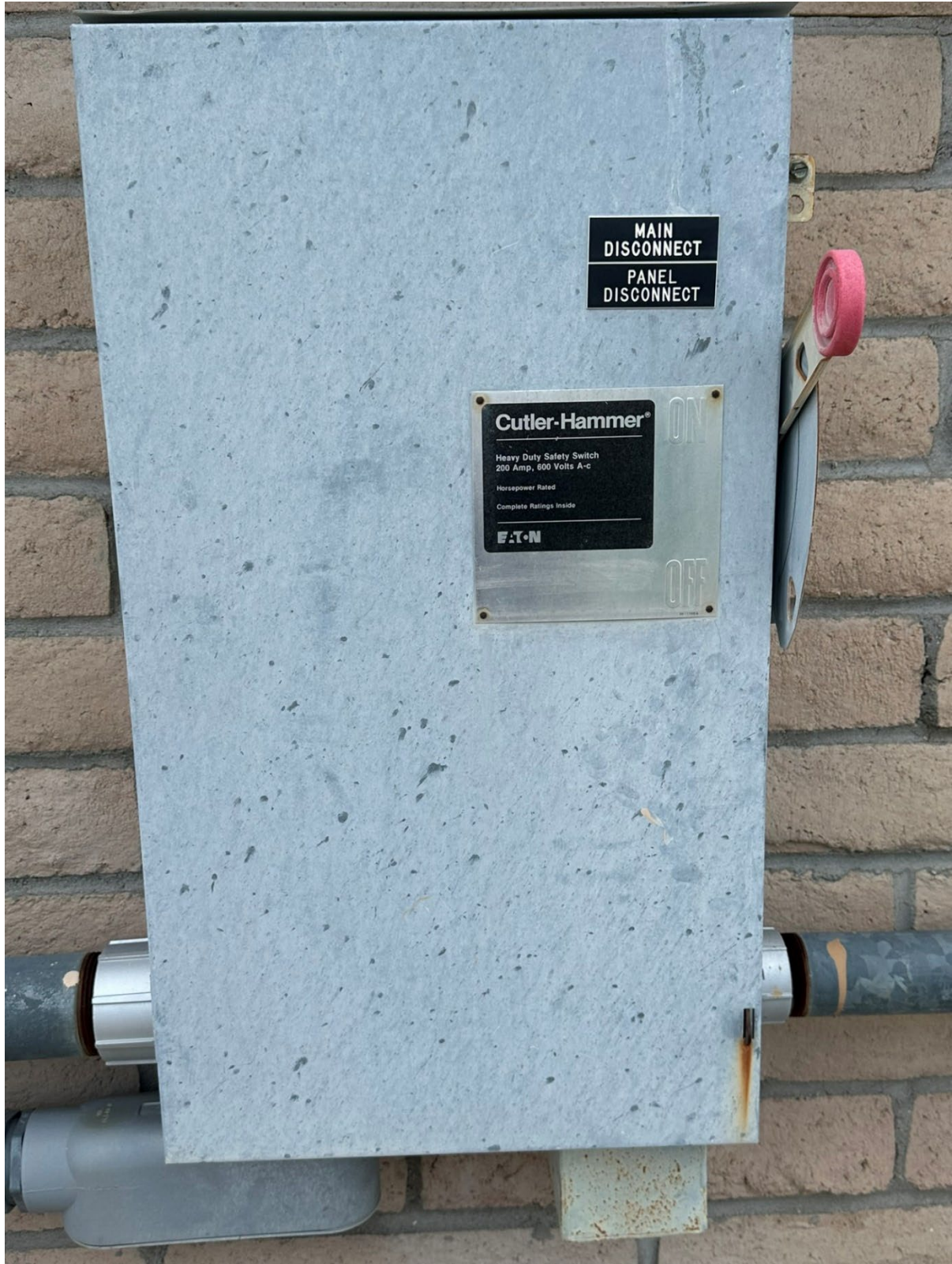
Figure 27: Main Disconnect – West Well Site
