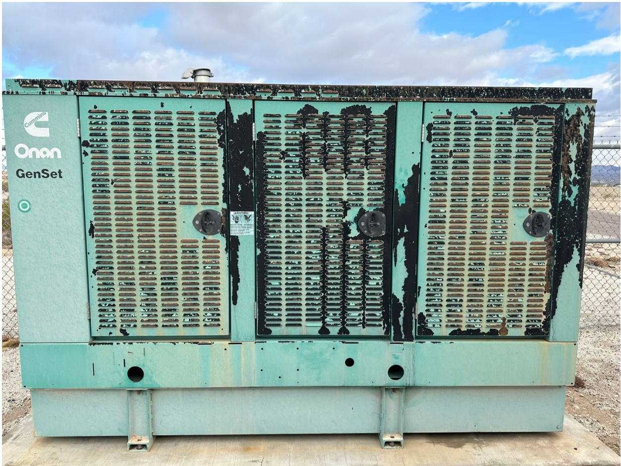
Figure 21: Standby Generator – West Well Site
