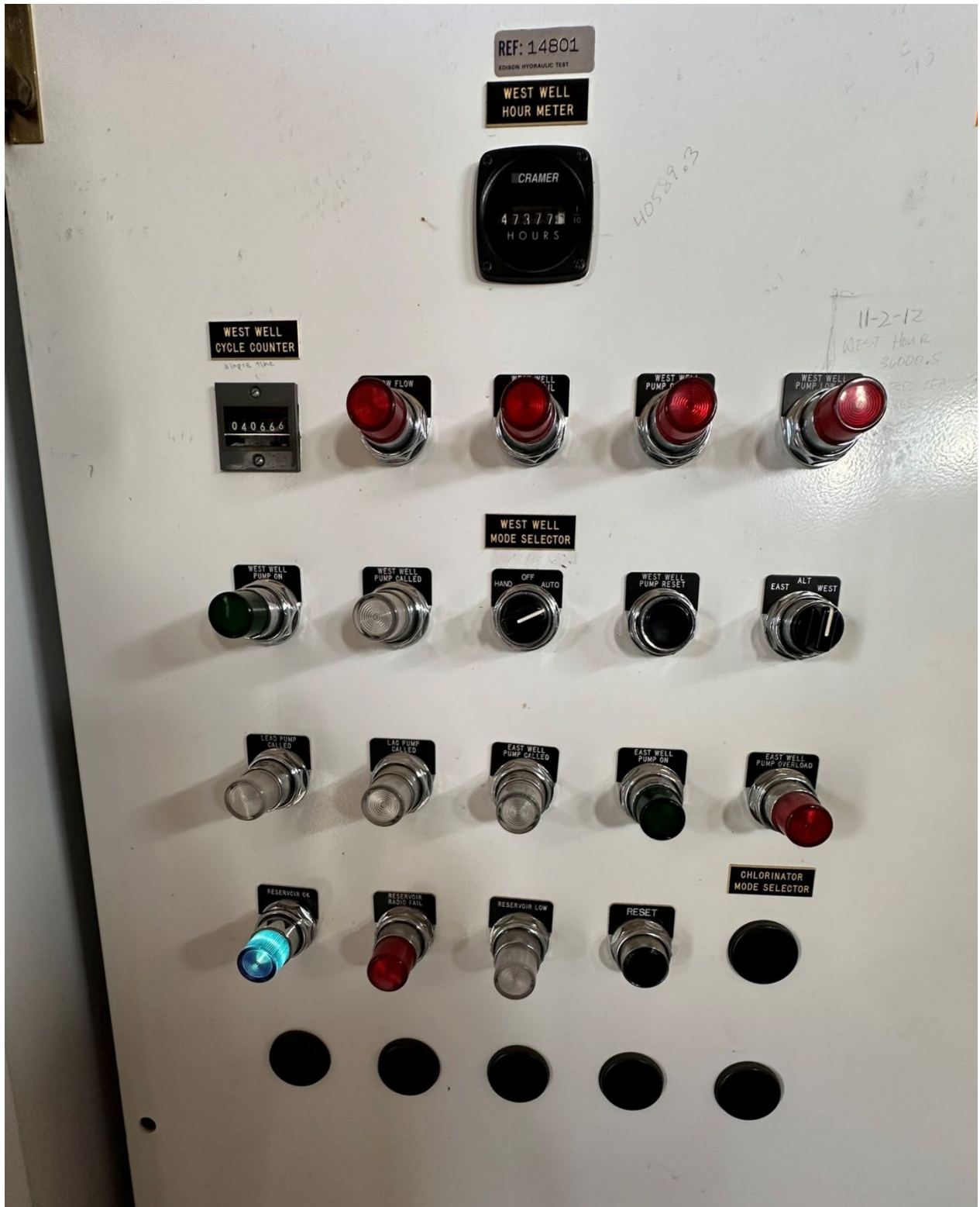
Figure 44: Close Up of Controls – West Well Site
