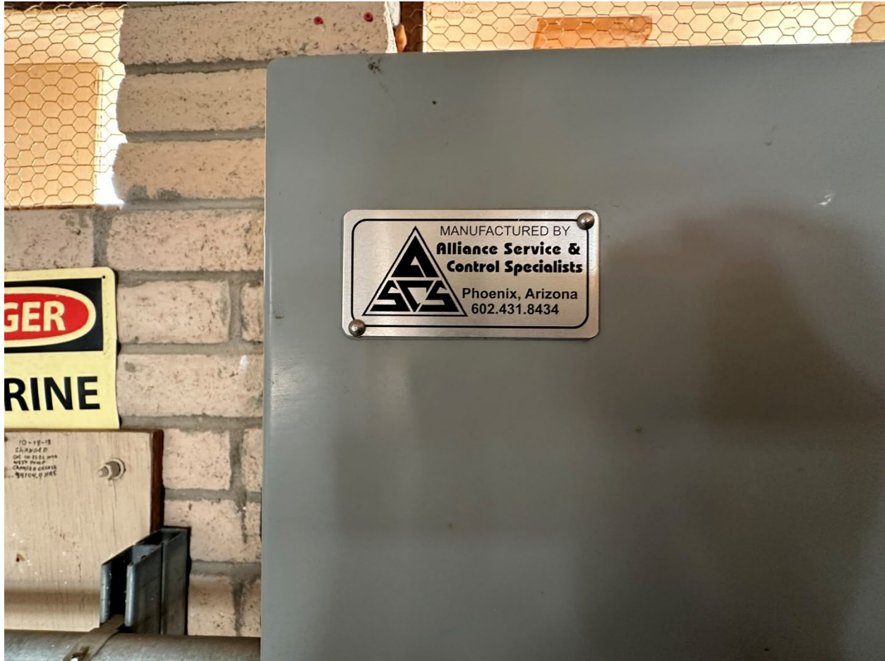
Figure 32: Well RTU Manufacturer Information – West Well Site
