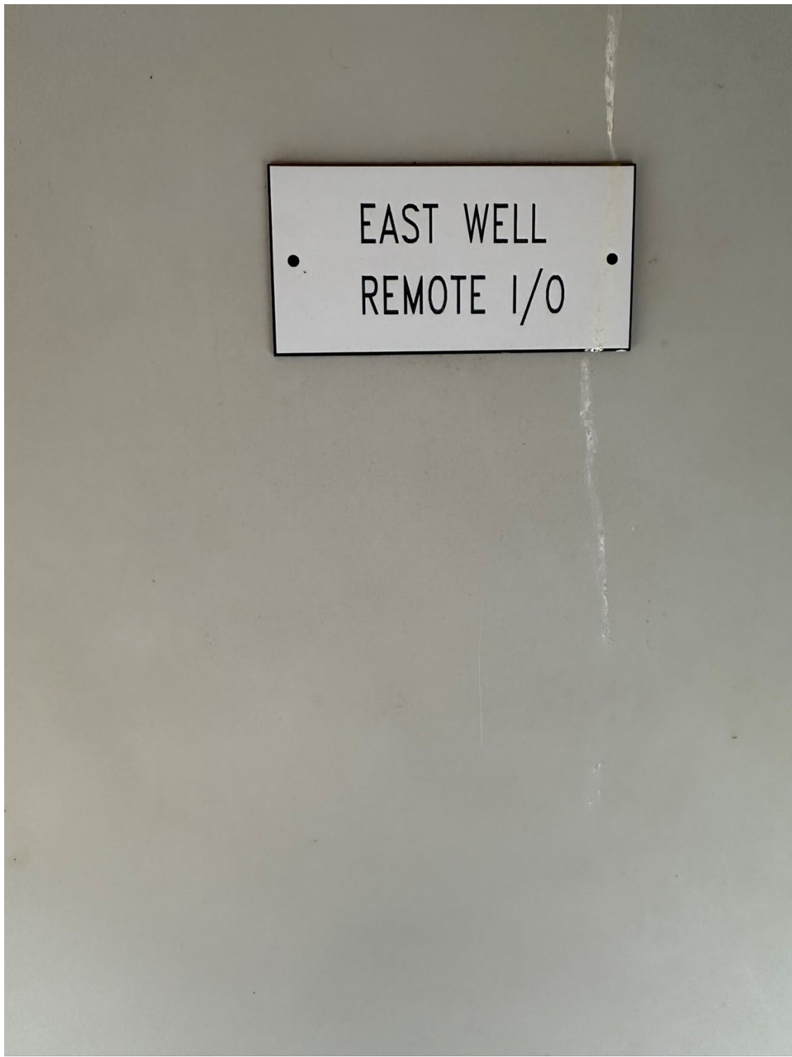
Figure 11: Well Remote I/O – East Well Site
