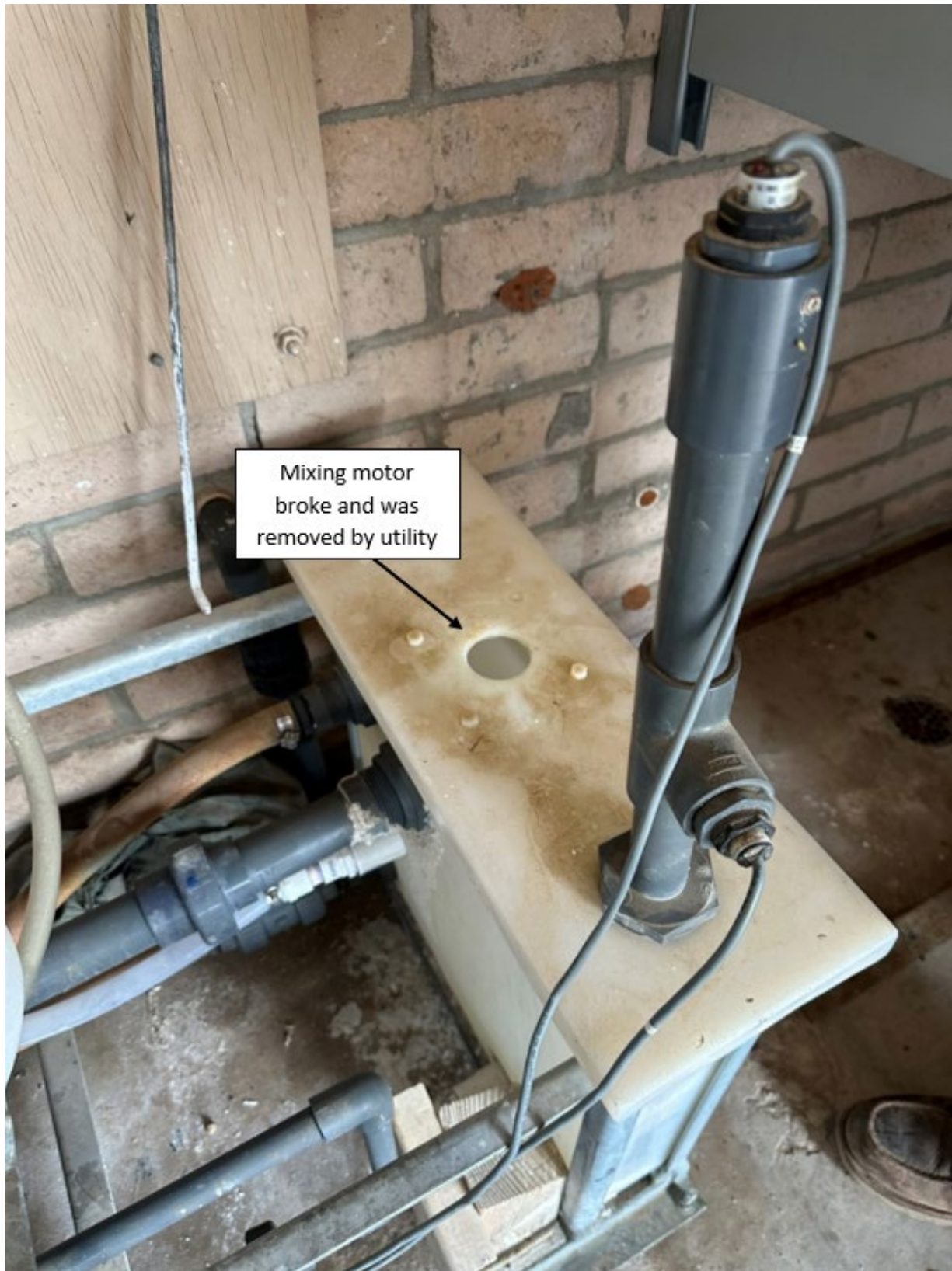
Figure 35: Missing Mixer Motor – West Well Site
