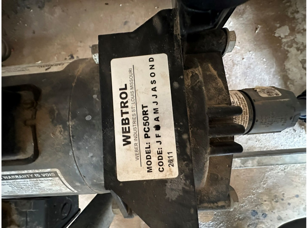
Figure 37: Chlorinator Pump Make and Model – West Well Site
