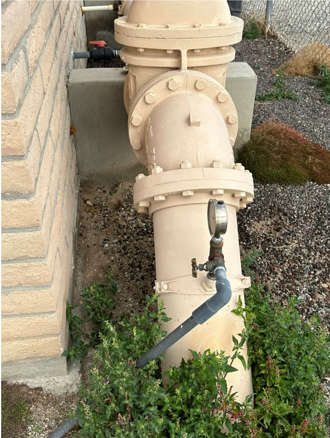
Figure 20: Close Up of Plumbing Behind Pumphouse - West Well Site
