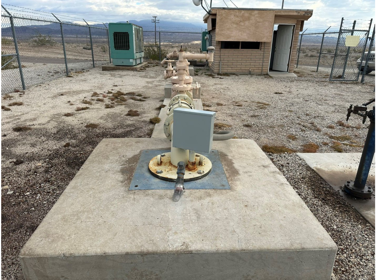
Figure 18: View from Well Head – West Well Site
