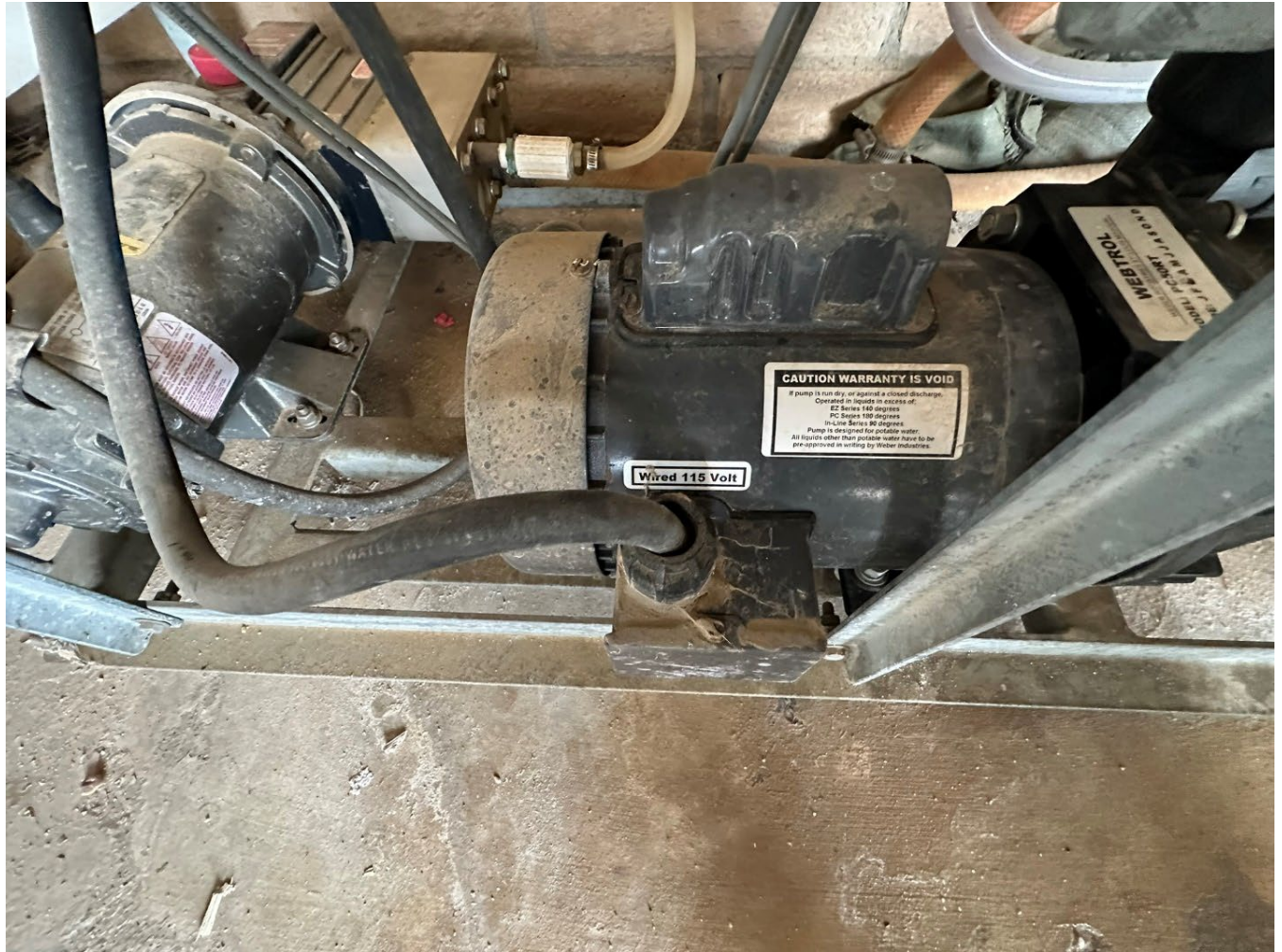
Figure 36: Chlorinator Pump – West Well Site
