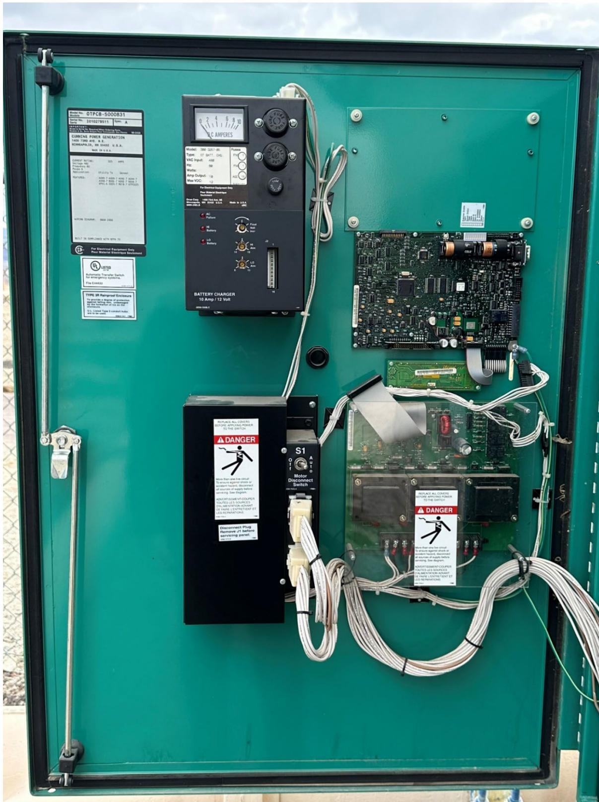
Figure 25: Inside view of Power Source #2 – West Well Site
