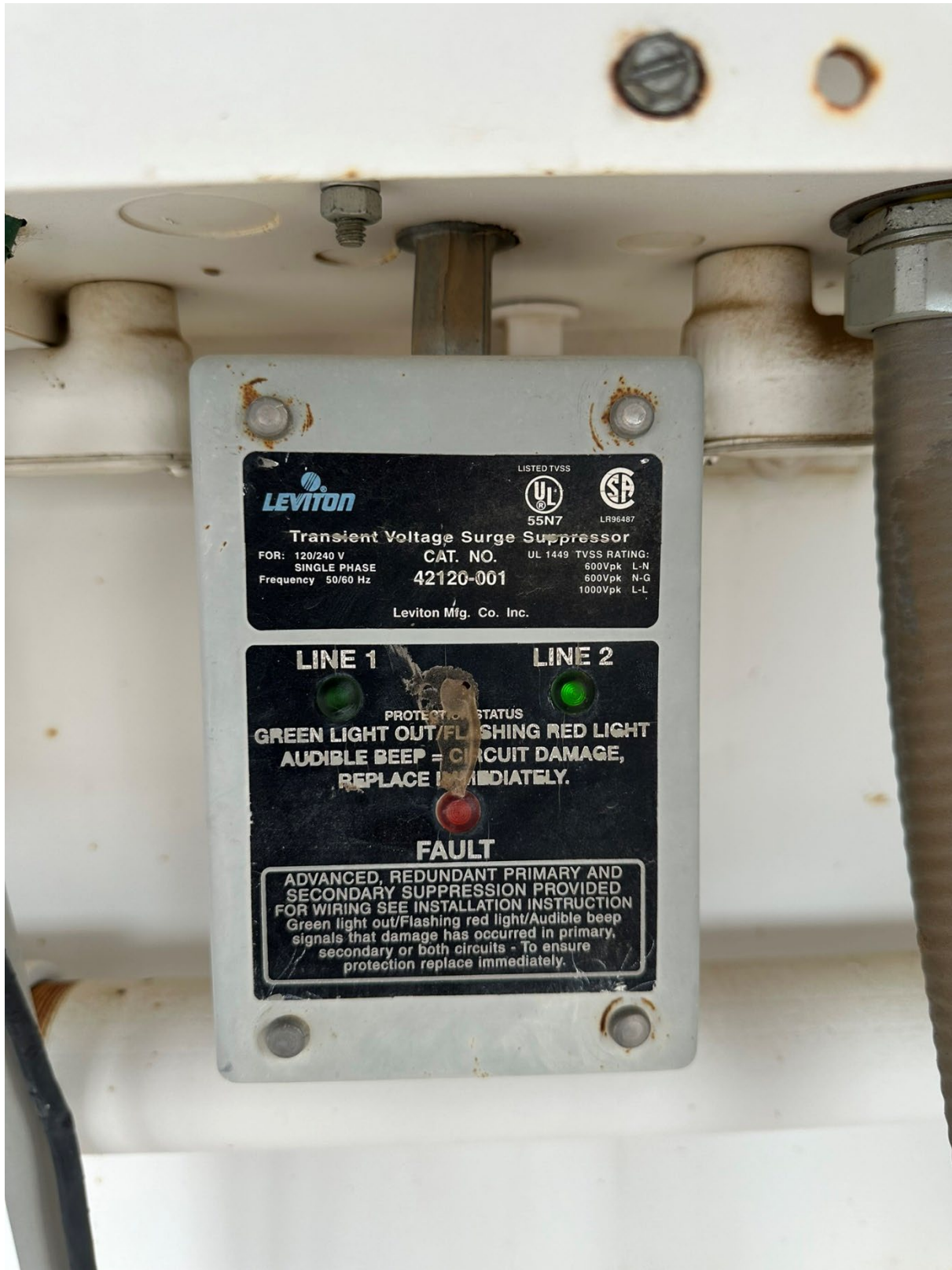
Figure 14: Well Surge Suppressor – East Well Site
