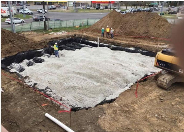
Stormwater Management – Chambermaxx System drainage pipes
