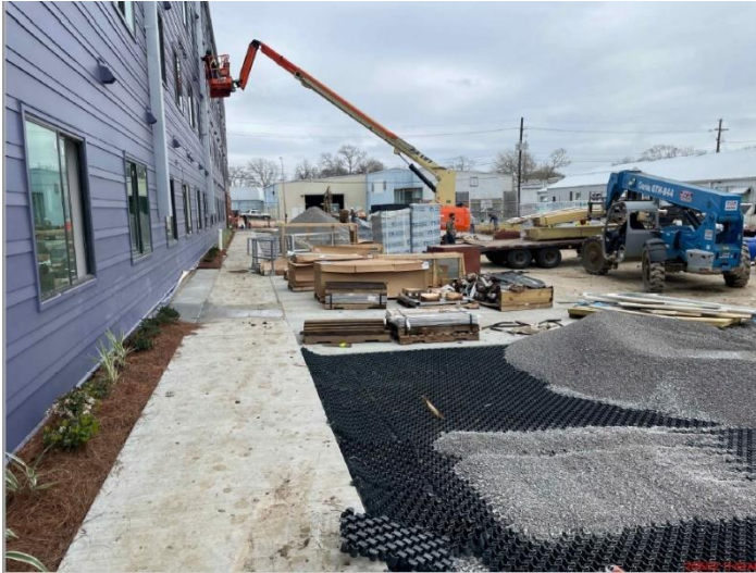
Stormwater Management – Grass and Gravel Paving System
