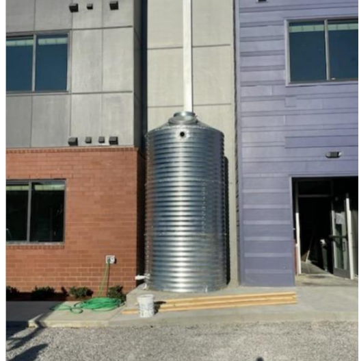
Stormwater Management – Rain Cistern
