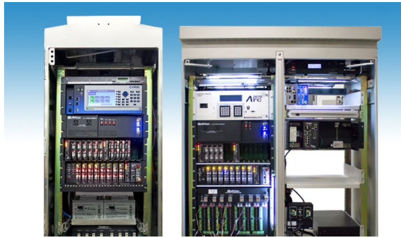
▼ FIGURE 8.1.2C – ATC CABINET
