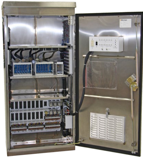
▼ FIGURE 8.1.1A - M CABINET
