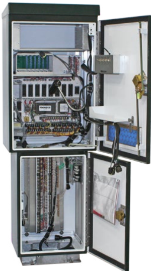
▼ FIGURE 8.1.1C - G CABINET
