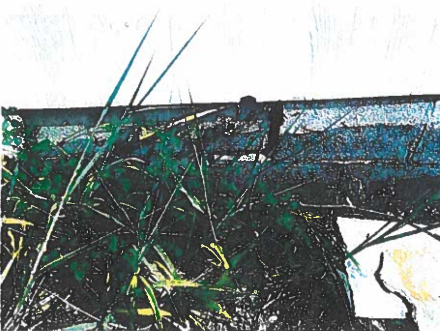
Figure 2 Misaligned blocks at foundation wall
