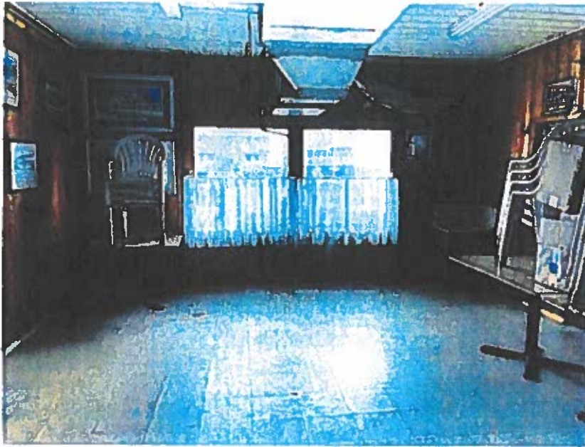
Figure 5 Bow in wood floor system.
