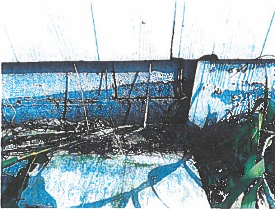
Figure 1 Cracks in mortar at foundation wall
