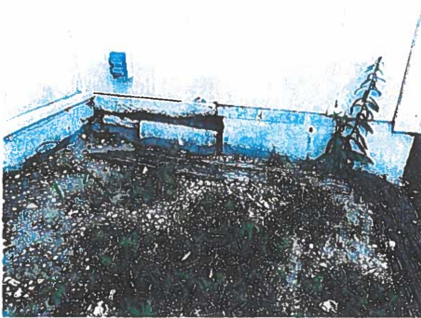
Figure 3 Damaged foundation on wall
