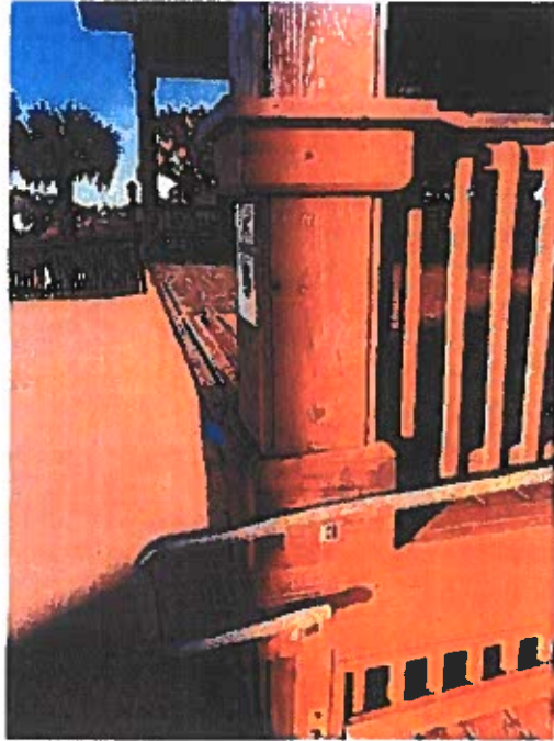
Photo 3 - Corner pile with no pile repairs
