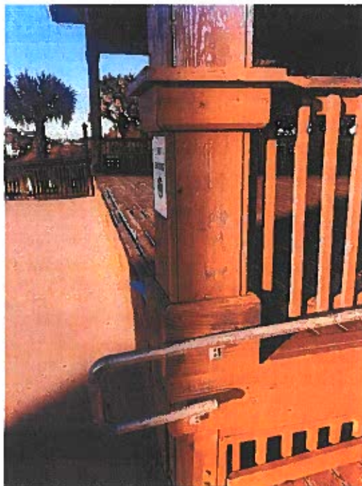
Photo 3 – Corner pile with no pile repairs
