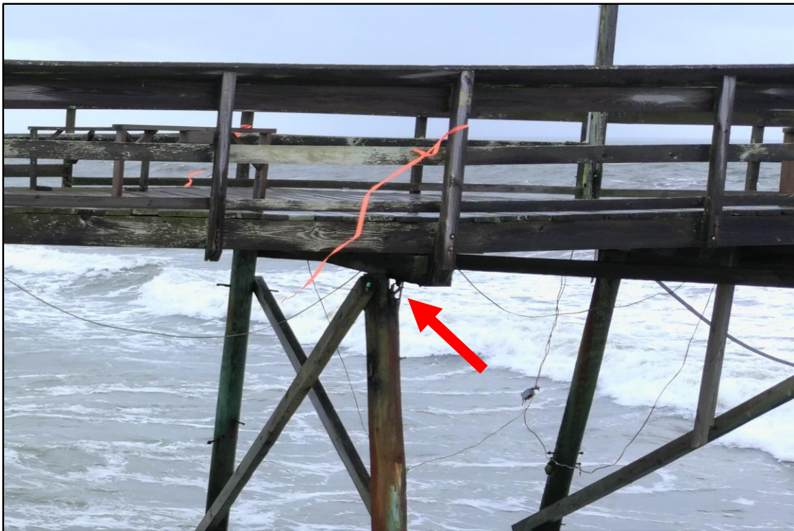
Photograph 8: Pile 25B - Top 18-inch pile is broke/overstressed
