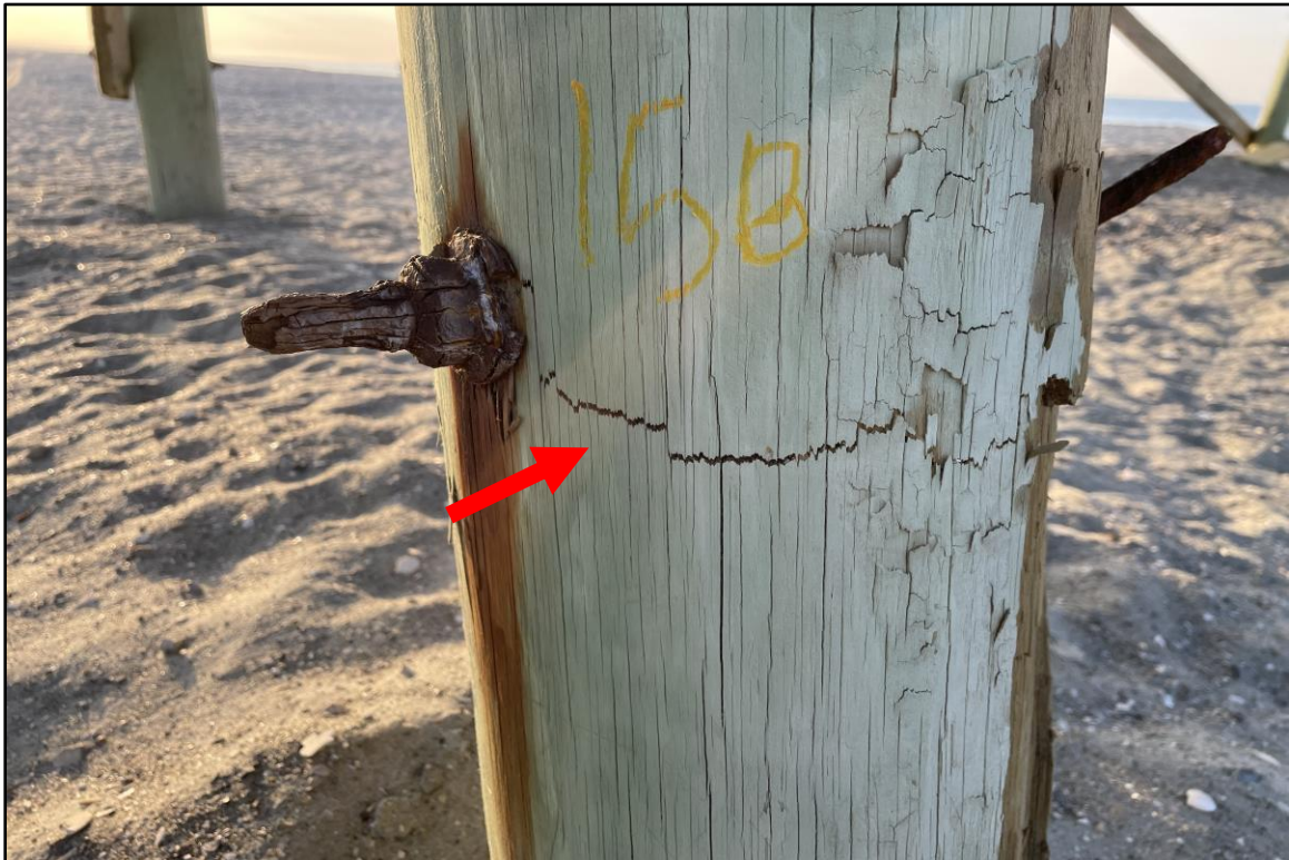
Photograph 5: Pile 15B – Pile fractured
