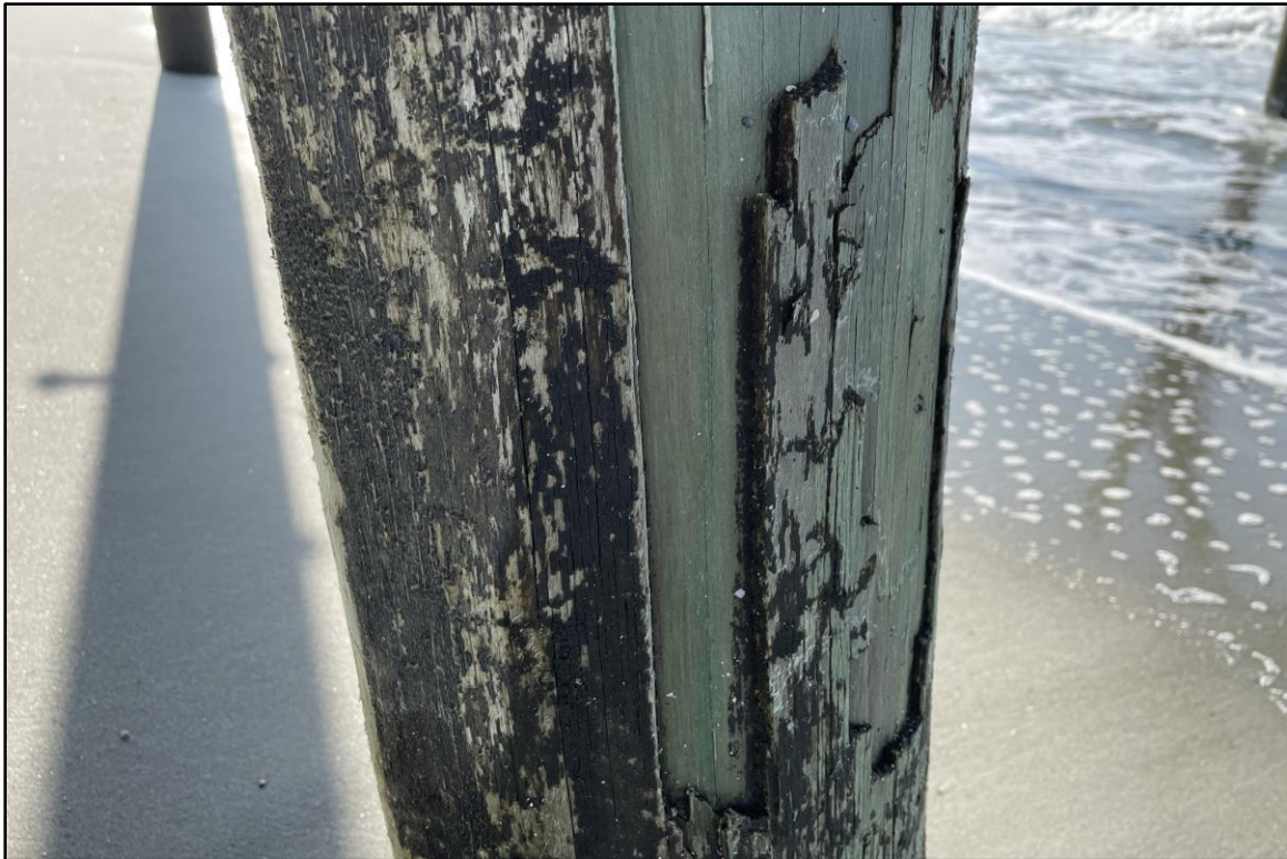
Photograph 2: Pile 25B – Typical shell peeling found on greenheart piles
