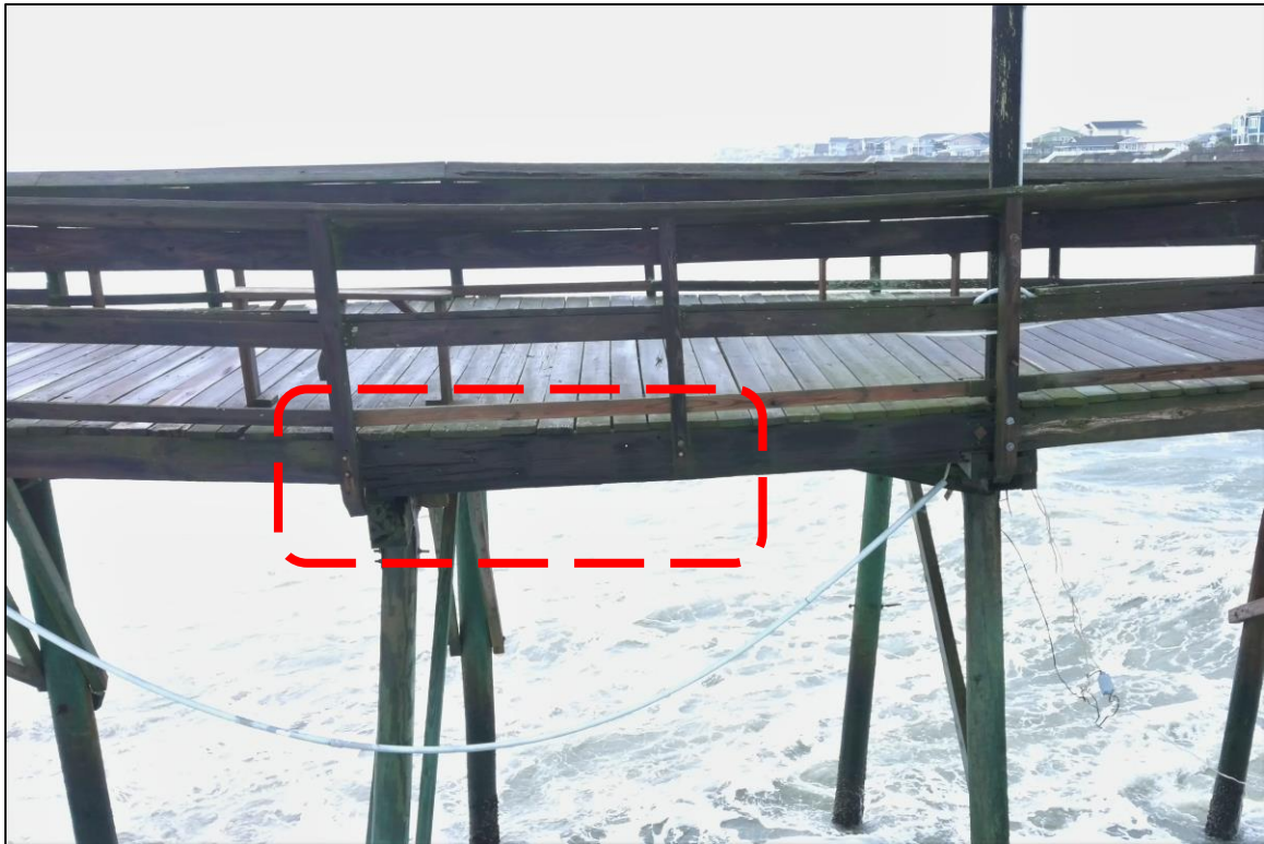
Photograph 14: Bent 27 - Overstressed pile cap & stringer
