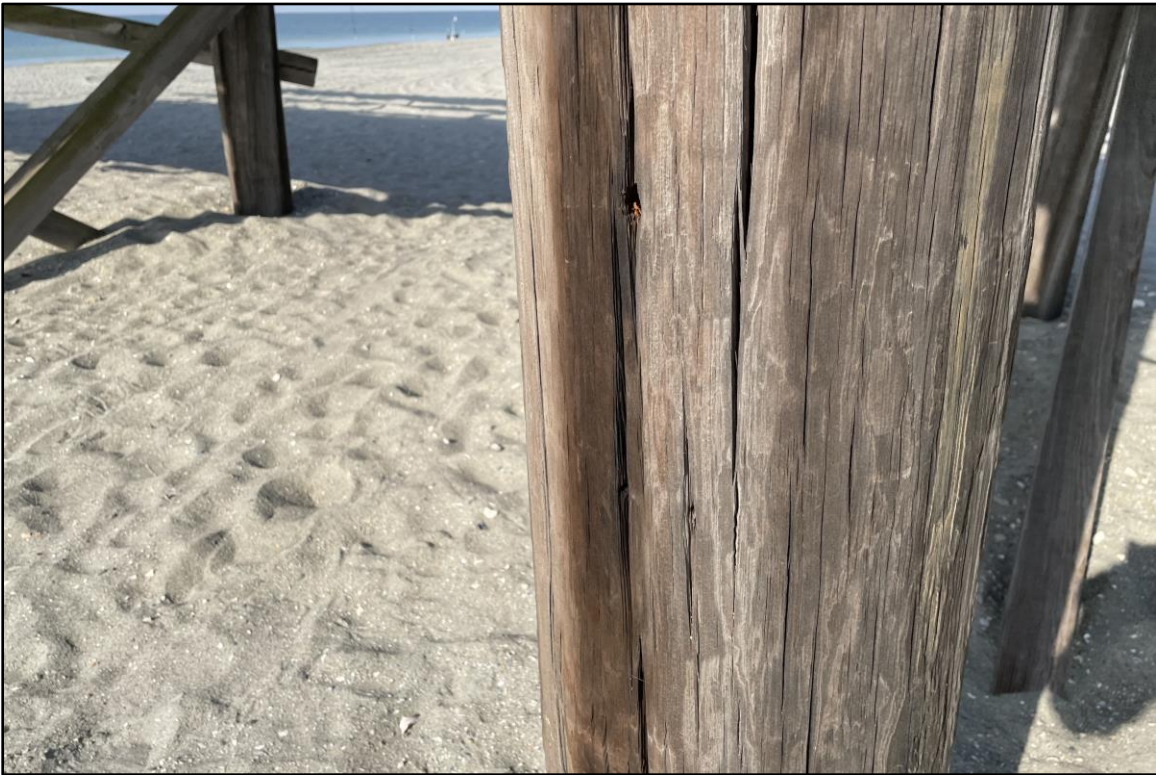
Photograph 3: Pile 7A – Typical checking and weathering found on original vintage piles
