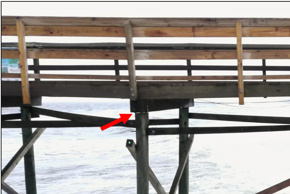
Photograph 6: Pile 17A - 100% Non-Bearing pile, timber cap supported by steel fish plates
