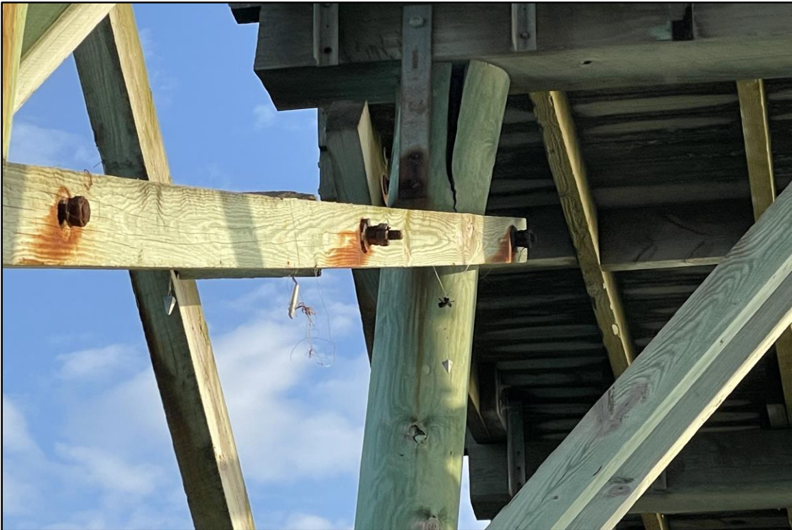
Photograph 12: Pile 50B - Top 18-inch pile is broke/overstressed
