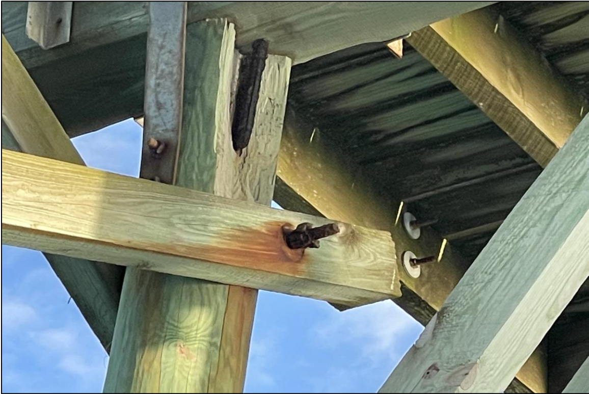
Photograph 11: Bent 49B - Overstressed pile cap & stringer
