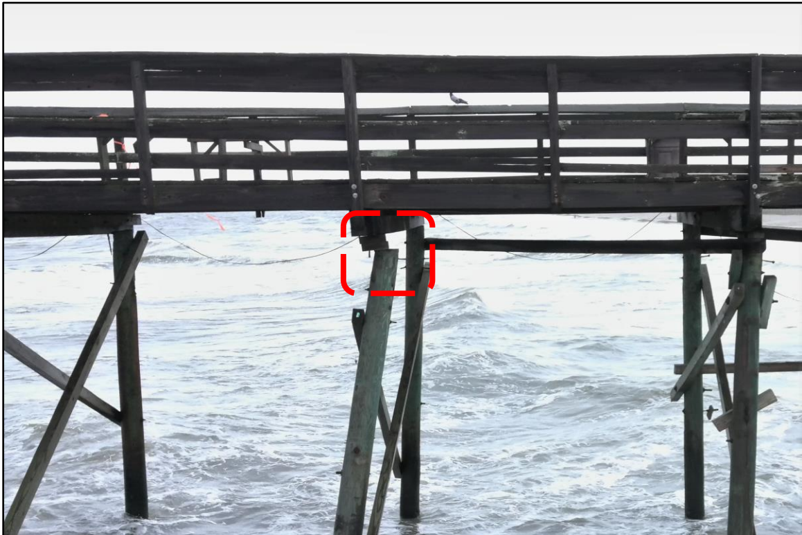
Photograph 7: Pile 24A - 50% Bearing due to displaced pile shims
