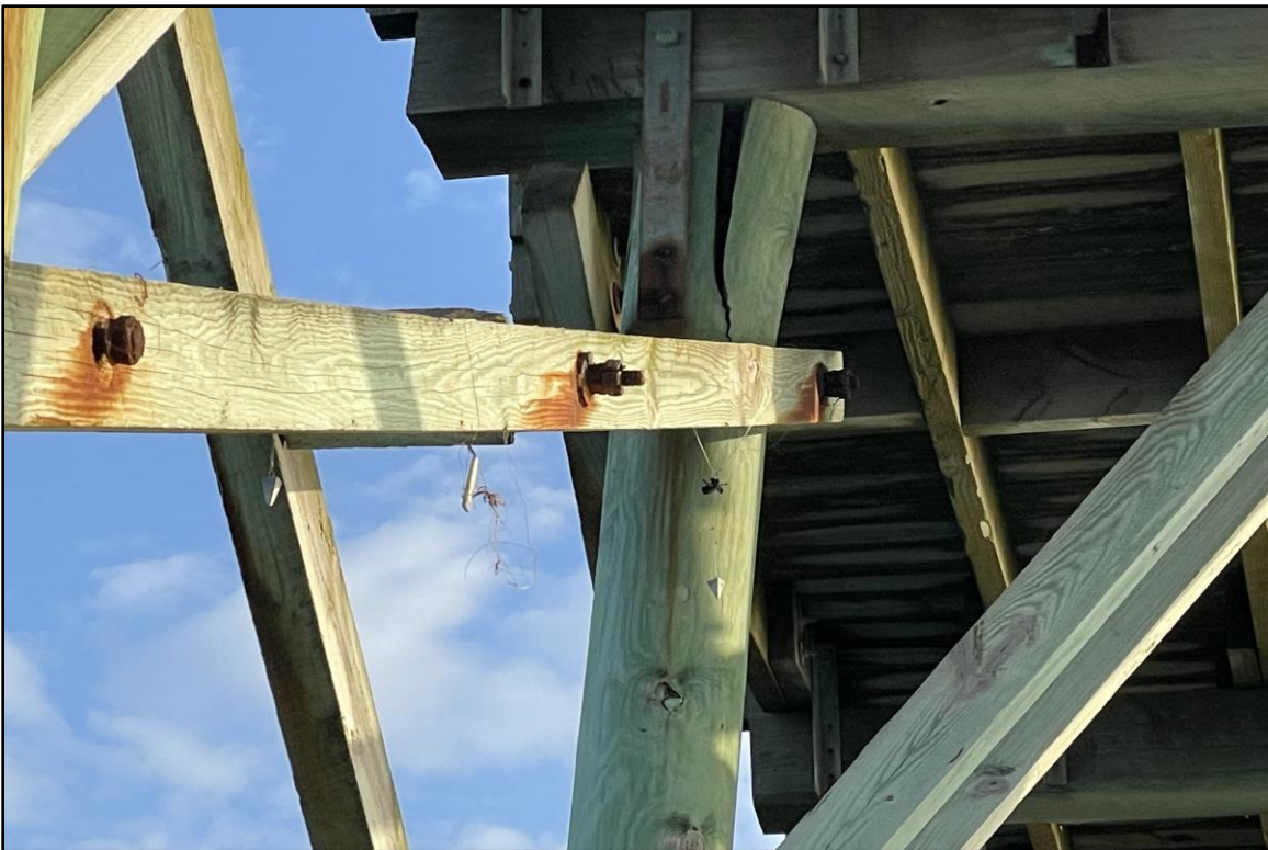
Photograph 12: Pile 50B - Top 18-inch pile is broke/overstressed
