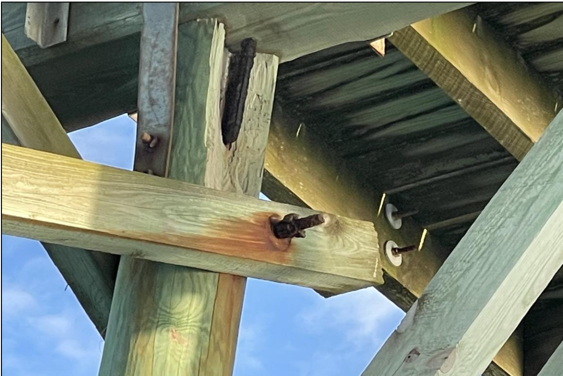
Photograph 11: Bent 49B - Overstressed pile cap & stringer
