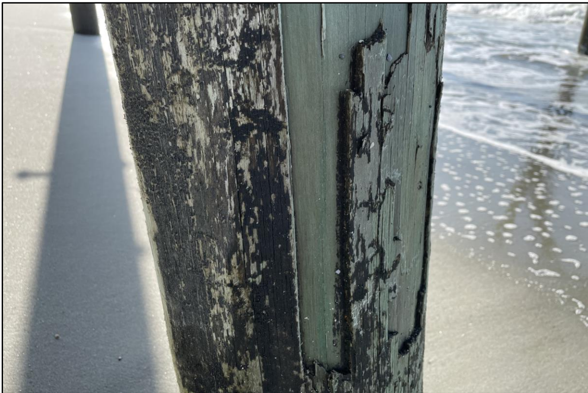
Photograph 2: Pile 25B – Typical shell peeling found on newer vintage piles
