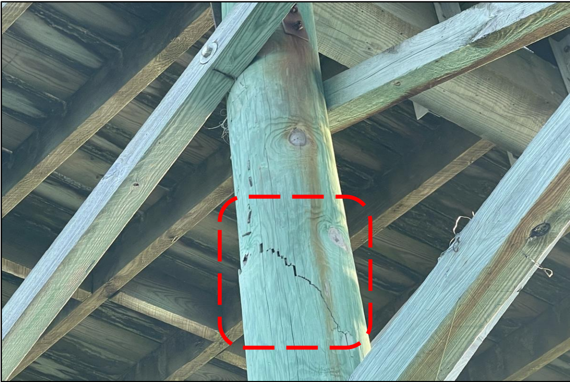
Photograph 10: Pile 47B - Pile is fractured 5feet down from top.
