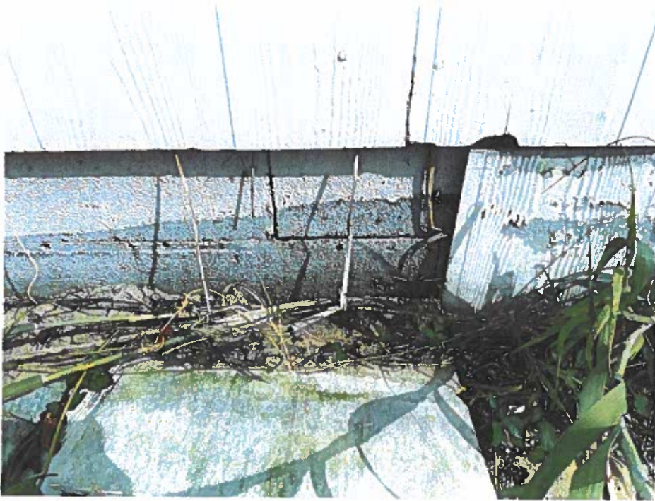
Figure 1: Cracks in mortar at foundation wall
