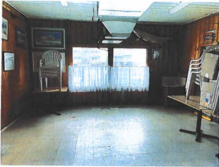
Figure 5: Bow in wood floor system.
