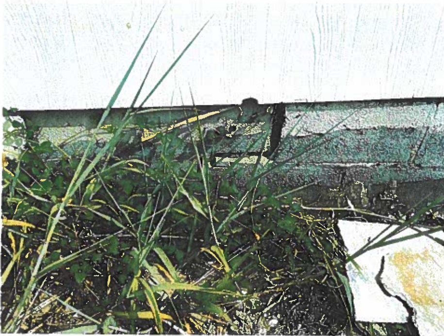
Figure 2: Misaligned blocks at foundation wall
