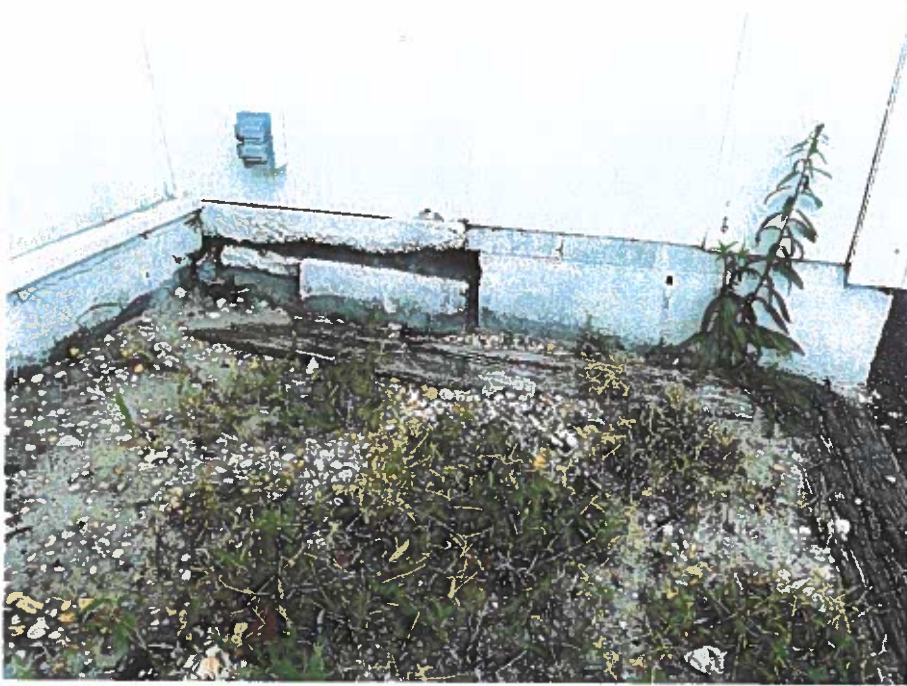
Figure 3: Damaged foundation wall
