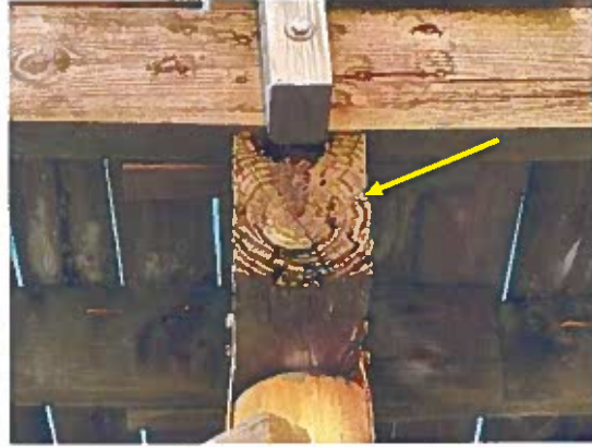
Photo 2 - Typical wood decay, when present, limited to exposed end grain.
