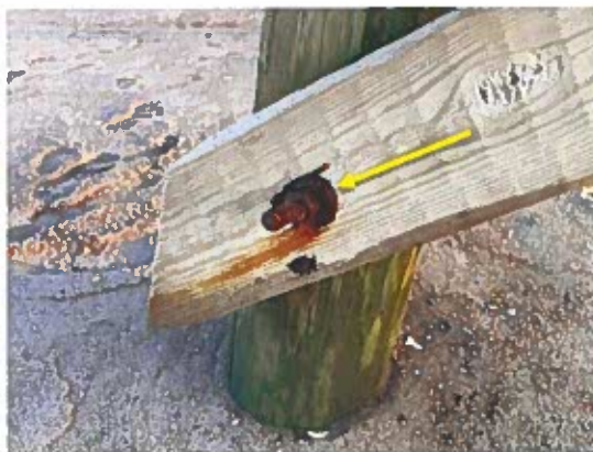
Photo 5 - Typical fastener corrosion.
