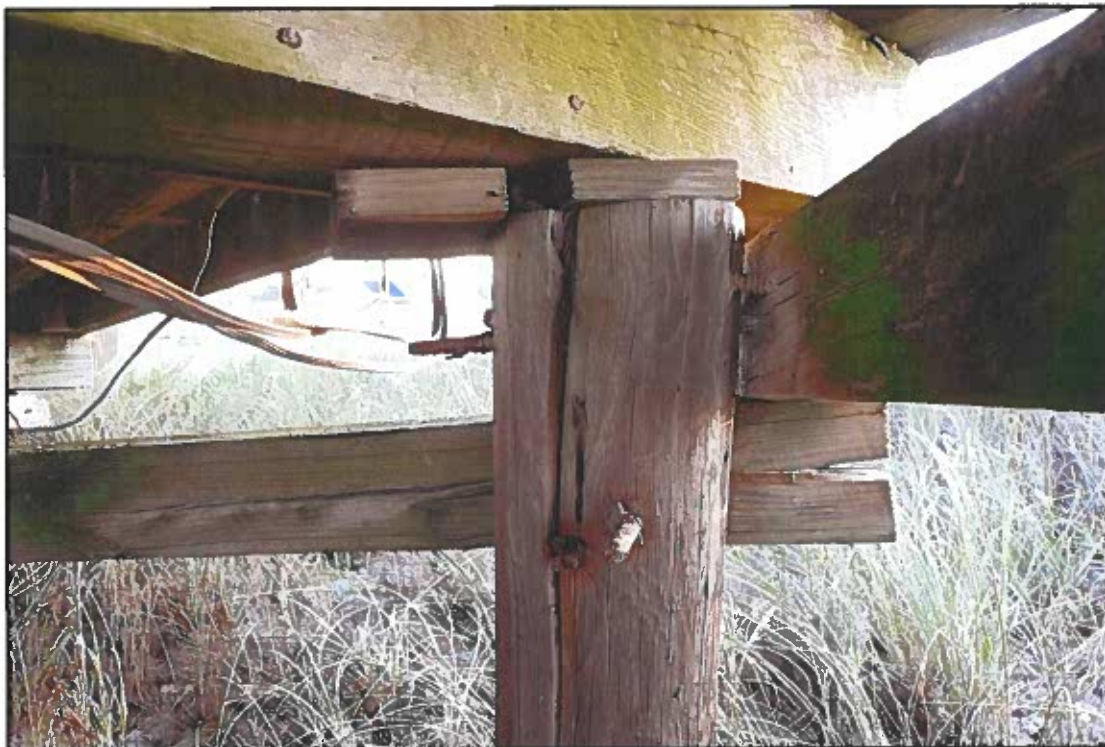
Photograph 7: Pile -4A – Typical split in top of pile.
