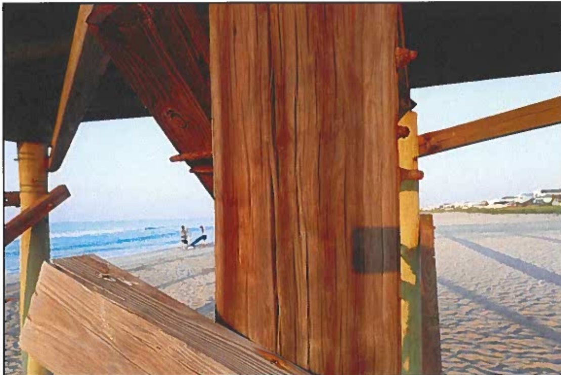
Photograph 4: Pile 12A – Typical light weathering and checking.
