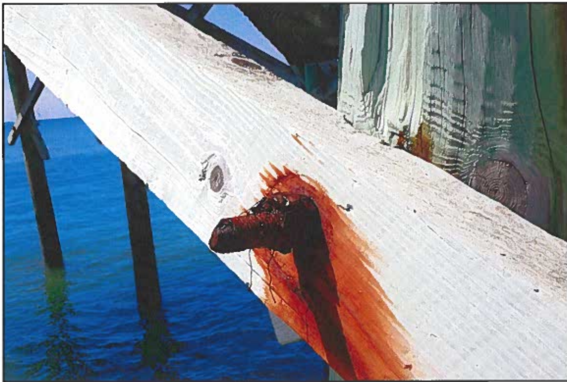
Photograph 18: Typical corrosion to lower bracing connection hardware.
