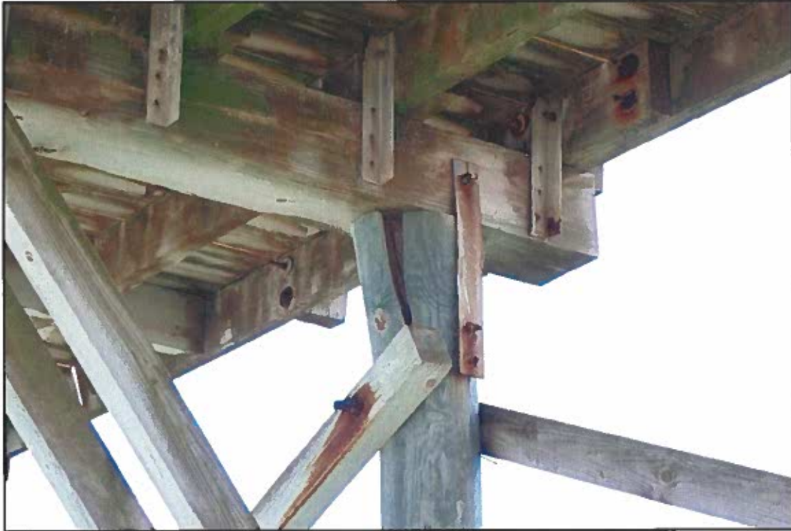
Photograph 13: Pile 50B – Typical split in top 18” of pile.
