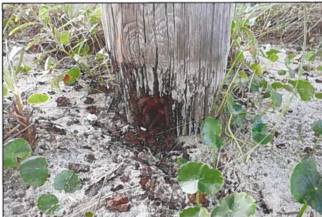
Photograph 8: Pile -2A – Insect damage at base of pile.
