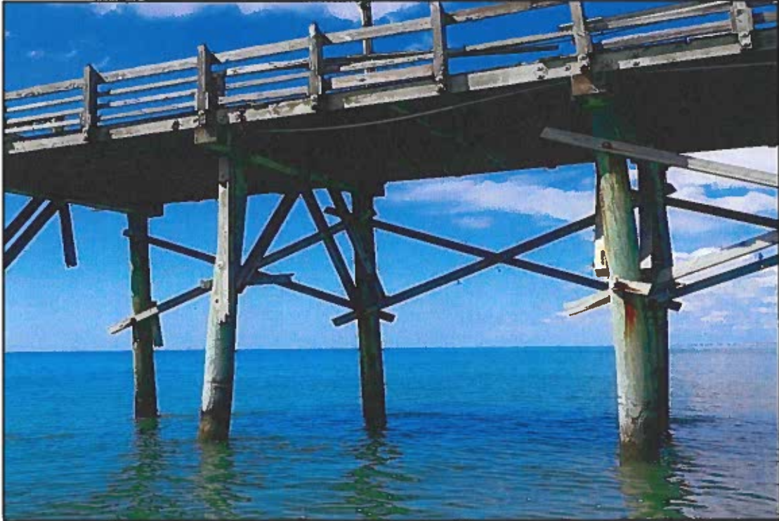
Photograph 17: Bent 51-52 – Typical bent-to-bent bracing broken and missing, looking west.
