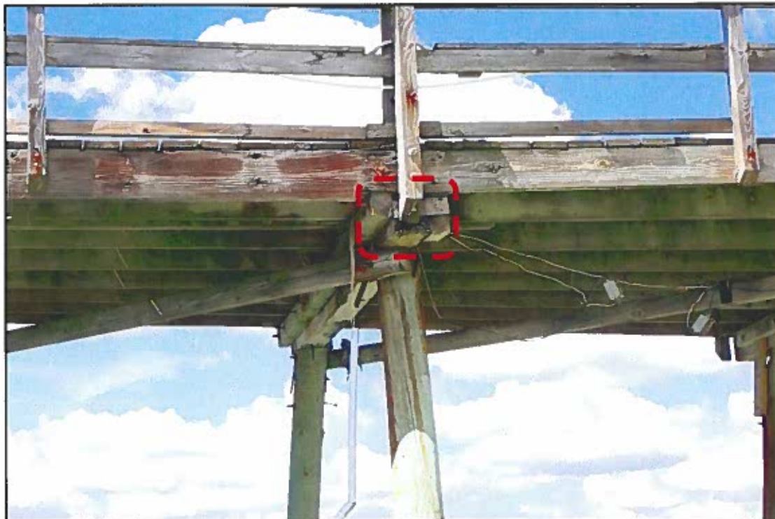
Photograph 16: Bent 26 – End grain rot on east end of cap, looking west.
