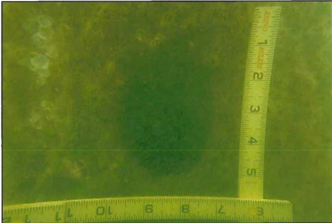
Photograph 15: Pile 52B – Hole in pile with section loss and hollowing due to marine borer.
