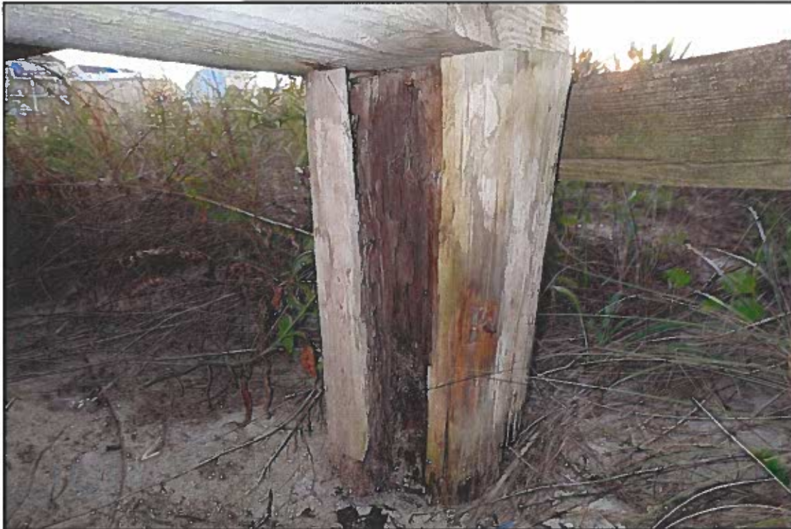
Photograph 6: Pile -5A – Heavy rot throughout pile.
