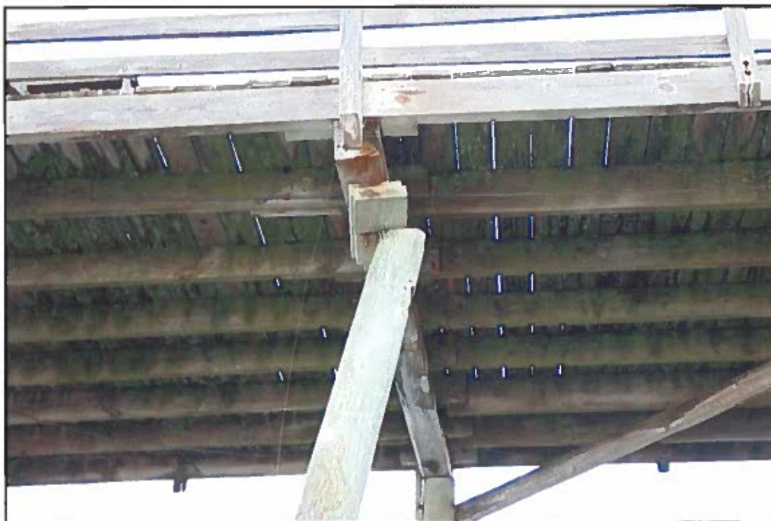
Photograph 10: Pile 24A – 50% non-bearing pile due to being displaced.
