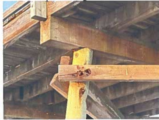
Photo 4 - General visual grade quality of timbers is at least consistent with No. 1. Fastener corrosion also visible.
