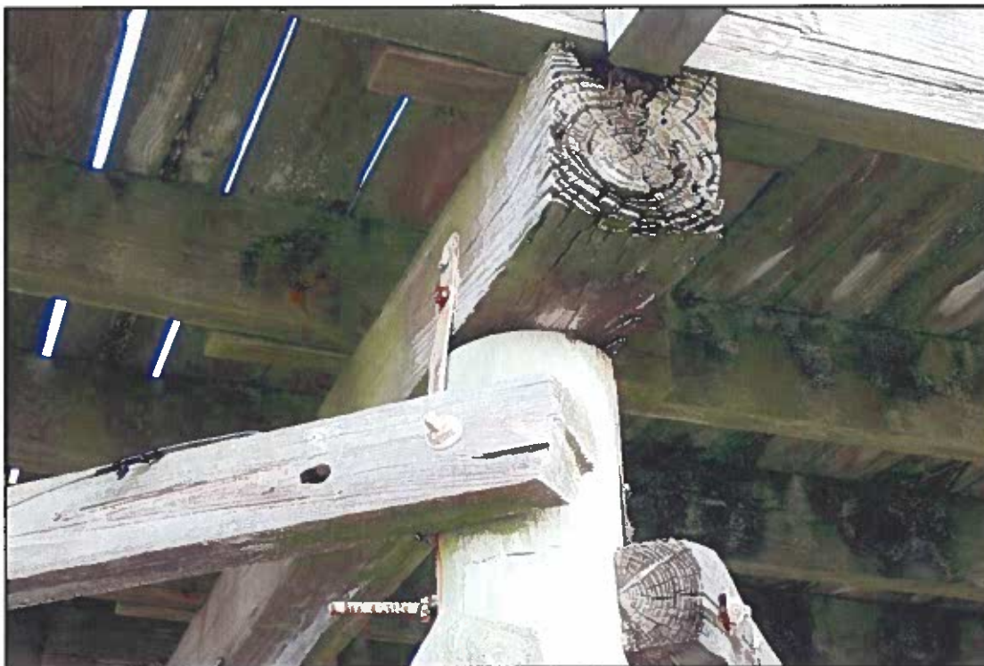
Photograph 9: Pile 17A – 100% non-bearing pile being supported by fishplates.
