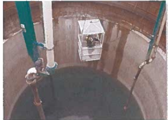
Potable water storage facilities
