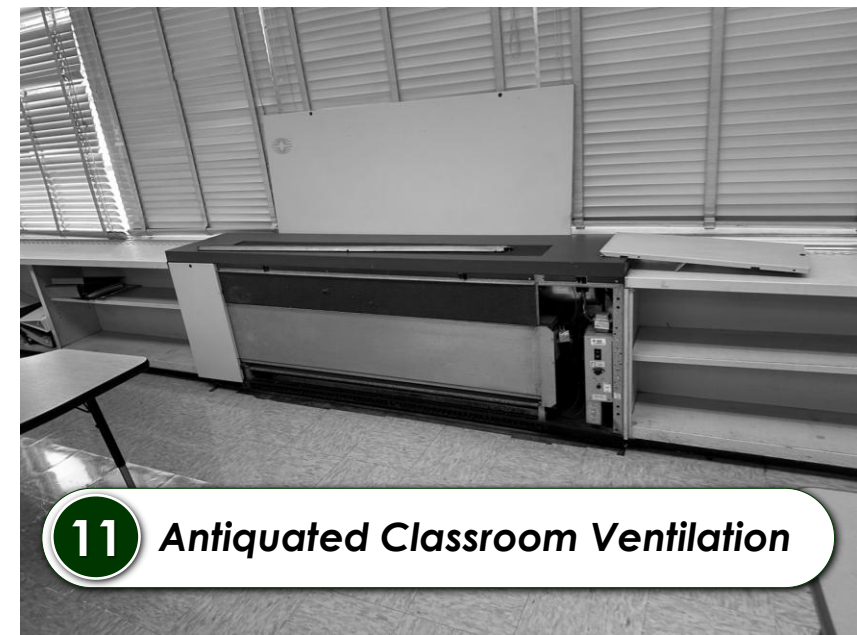
11 Major Equipment at "EOUL" (End of Useful Life)
