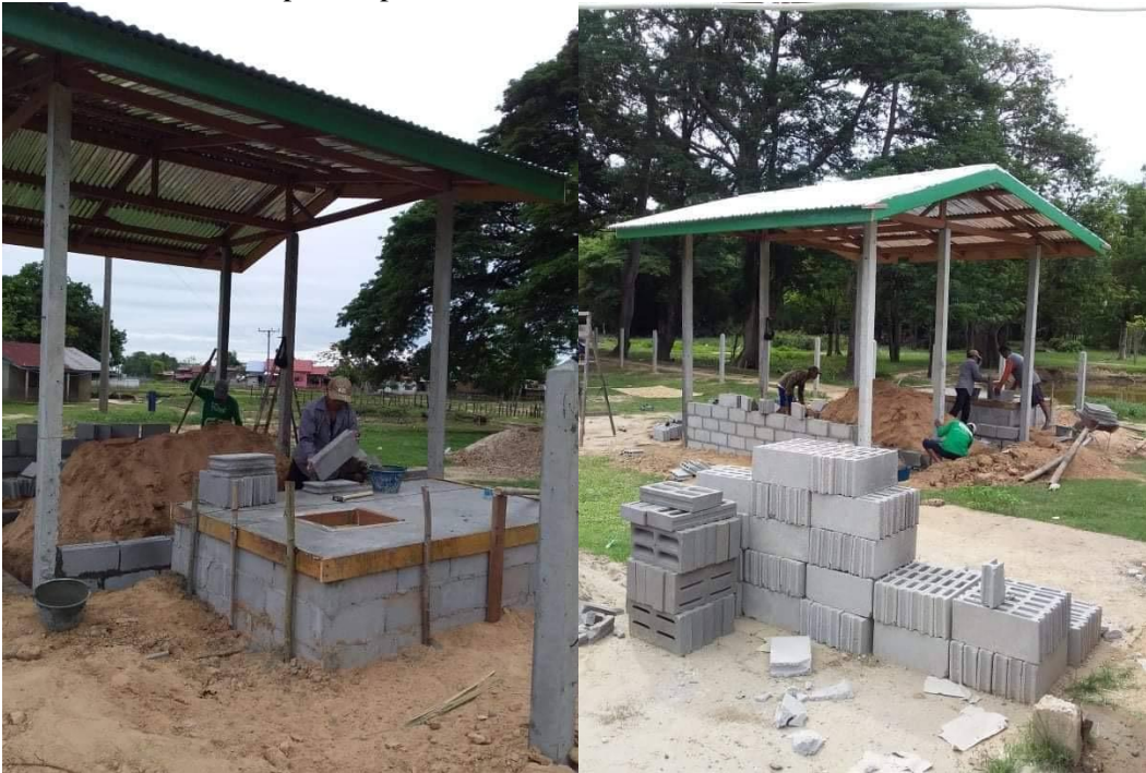
Motion 22-01 Laos Quality of Life - School Bathrooms in Ban Lam Phan, Laos Construction and completion photos.
